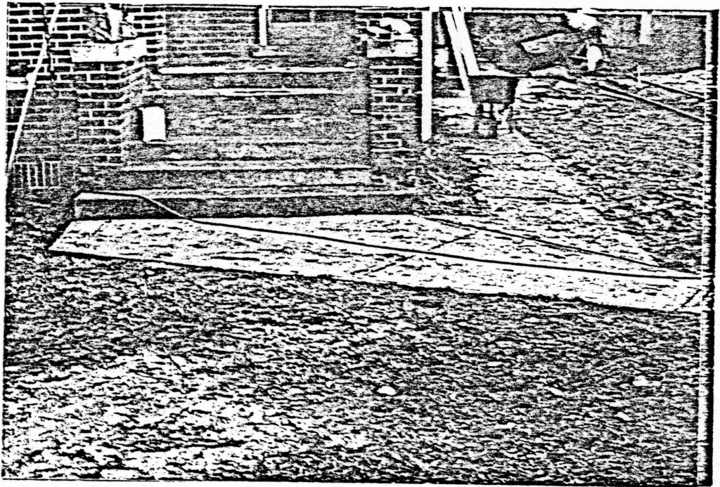
Photo showing the deterioration in the brick work along the front approach. Also, the sidewalk along the front and to the rear entry had been replaced.
