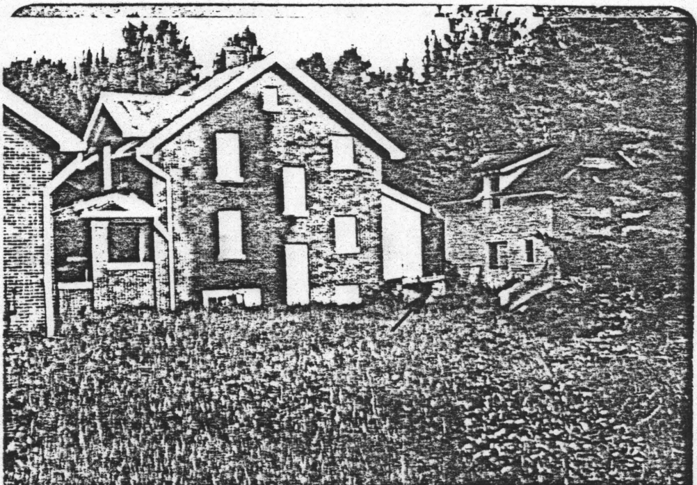
East view of Keeper's Quarters. Arrow shows the deterioration in the rear porch.
