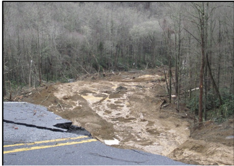
Figure 4. Landslide and road wash-out on US 441, January 2013
