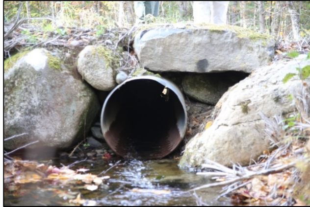
Photo 4: Obstructed Culvert on Loop Road
