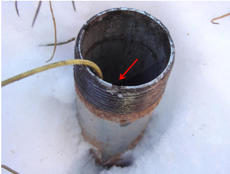
Figure 8. The measuring notch on the well casing
