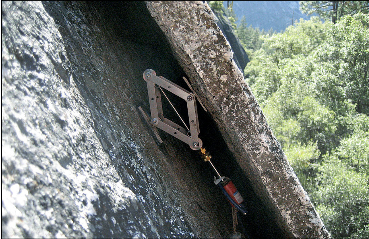
Figure 30. Vibrating wire scissor-jack crackmeter (image: Geokon Inc.) installed in a crack in Yosemite.
