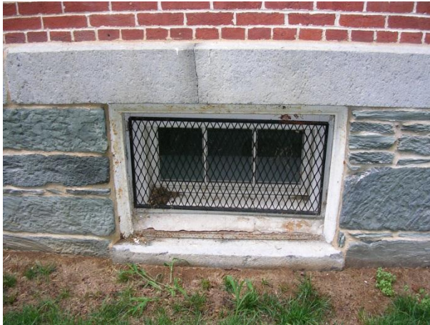
Figure 1 : An example of the window conditions prior to the preservation work completed by the HPTC wood crafting team.
