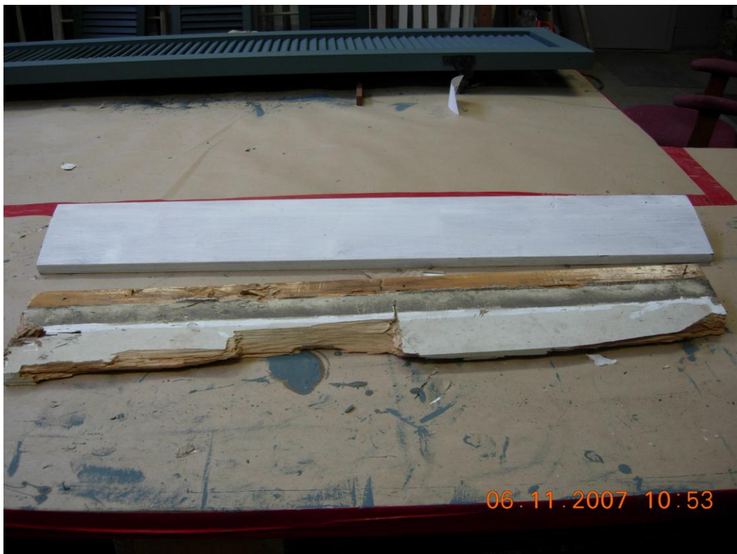
Photo 4: Deteriorated jamb and freshly primed replacement jamb
