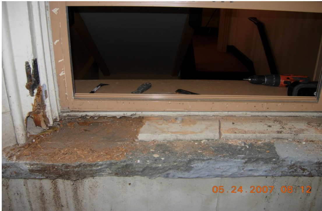
Photo 3: Sill removed due to deterioration and left jamb rot pocket being removed for consolidation.
