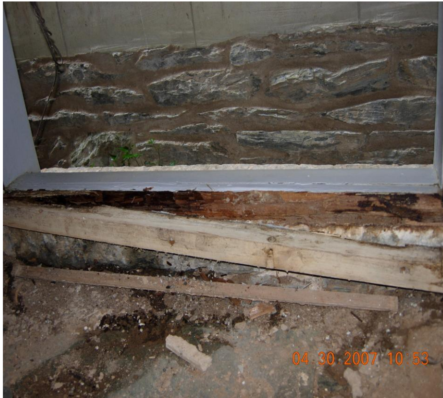
Photo 2: Deteriorated sill located on the basement level of building 36.
