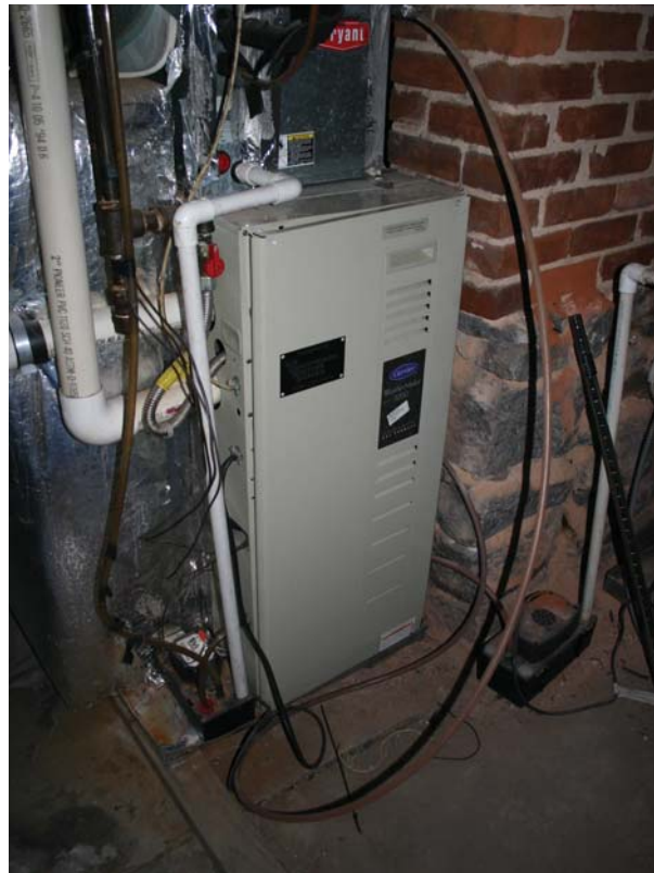
Figure 72. Unfinished Room 004, air handling unit.
