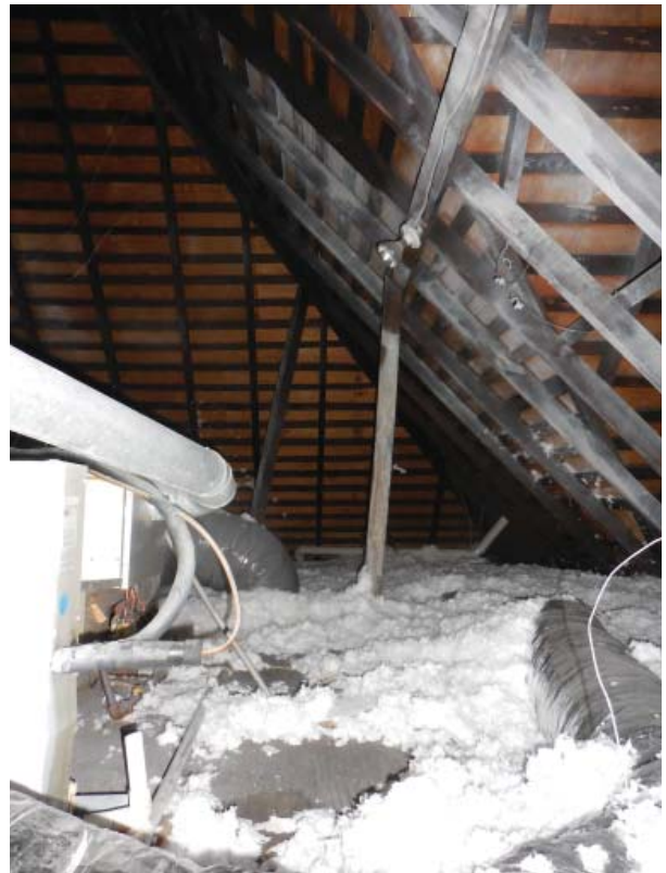
Figure 58. Attic view toward south with HVAC equipment.
