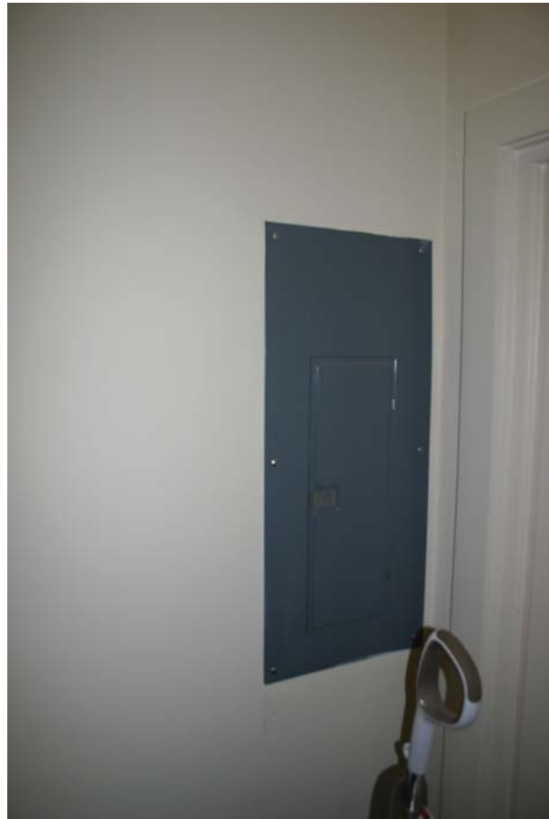
Figure 98. Electrical panel, Stair Hall 110.
