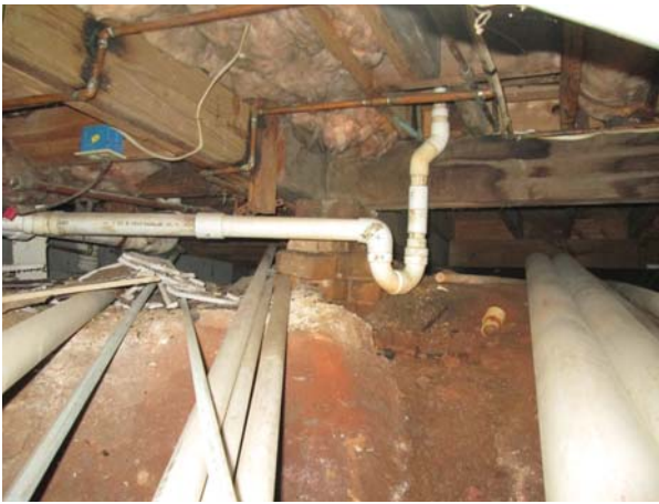
Figure 47. Undermined and deteriorated pier in crawlspace.
