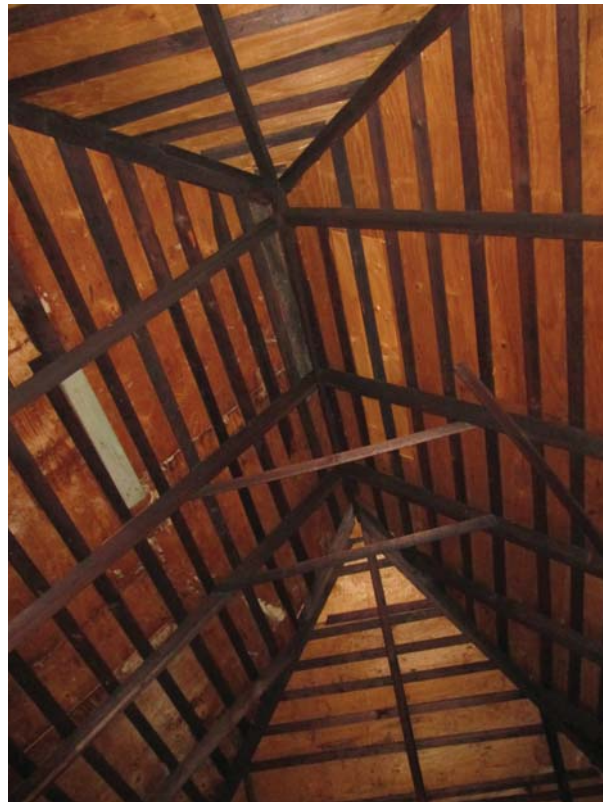
Figure 51. Roof framing in attic with missing collar tie.
