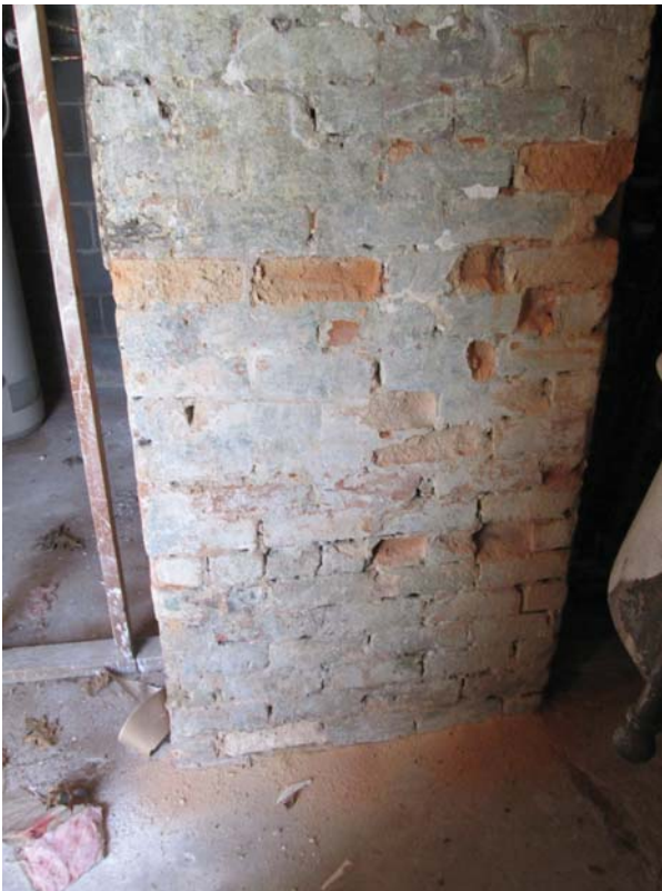
Figure 48. Base of chimney in basement showing failing brick and mortar.
