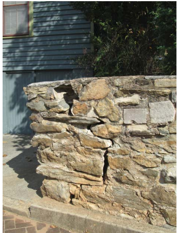
Figure 49. Cracked wall at north west corner of site wall. Northern segment is overturning, causing crack at the western face of the wall at the corner.
