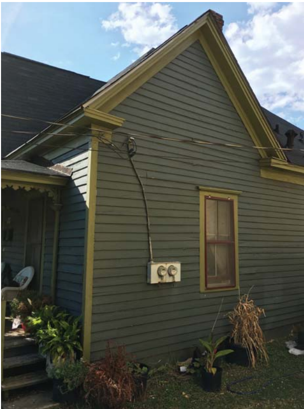
Figure 54. Electric service and meter, east elevation.
