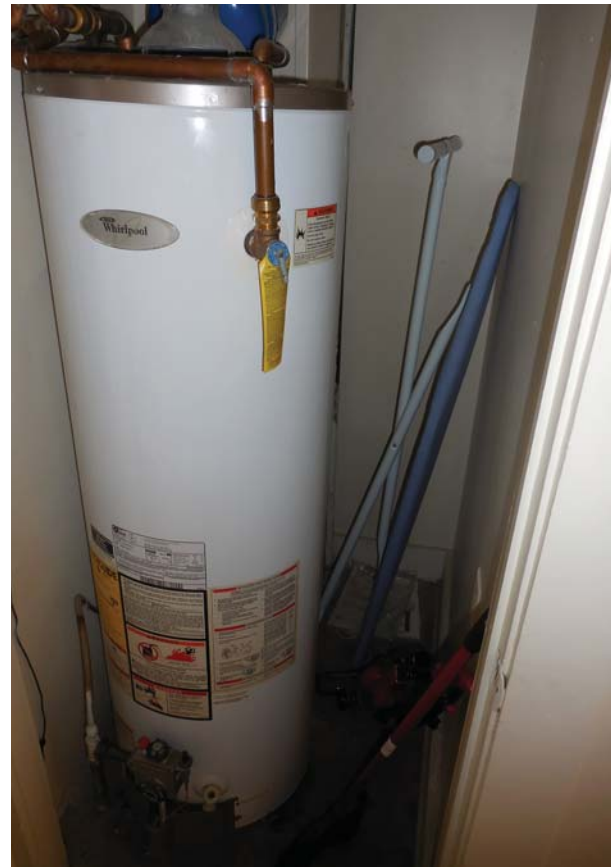
Figure 75. Hall 203, water heater in utility closet.
