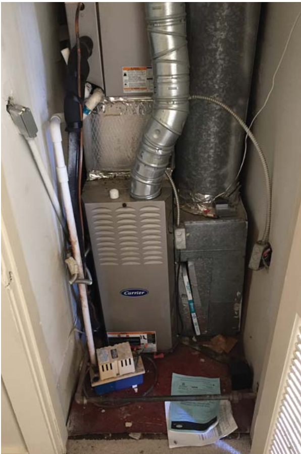
Figure 67. Hall 103, mechanical closet and air-handling unit.
