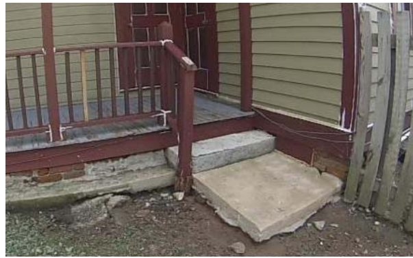
Figure 49. Undermining of concrete and decayed post at rear porch.
