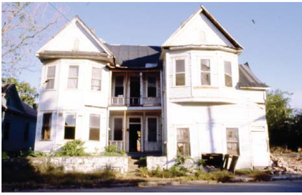
Figure 31. 550 Auburn Avenue prior to rehabilitation efforts (undated photo, pre-1988 repairs), SERO Archives, Slide 550014.
