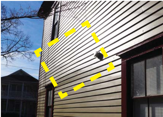
Figure 50. Bulge in wall sheathing on east side of house. Outline of area added for emphasis.
