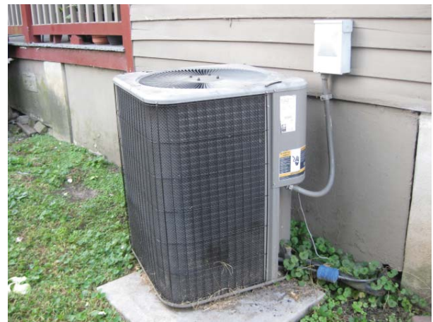
Figure C9. Heat pump at north side of building.
