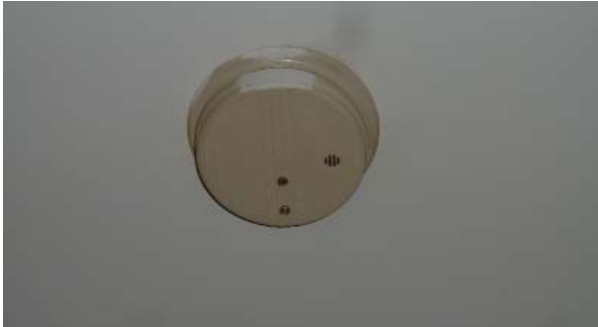
Figure C12. Ceiling-mounted, combination smoke and carbon monoxide detector.
