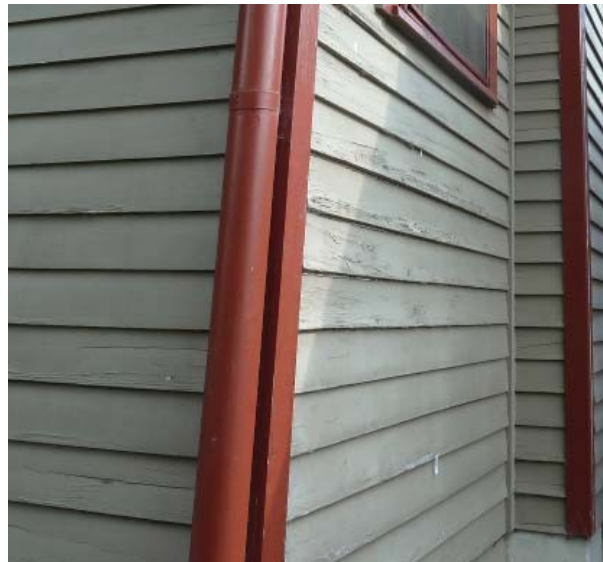
Figure C14. Note the checks and splitting of the siding.
