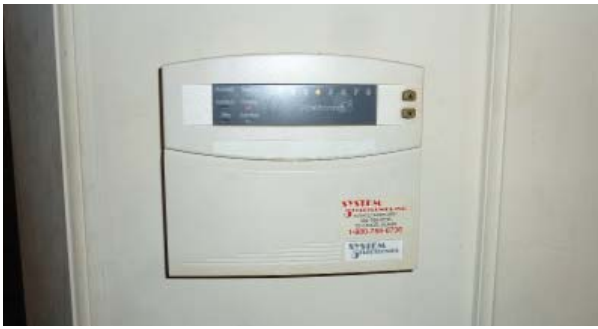
Figure C11. Panel box for modern security system.
