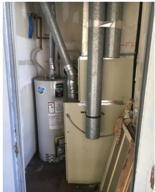
Figure C10. Water heater and Furnace in Room 109, the mechanical closet. Photograph taken at 484 Auburn Avenue, where access was provided.
