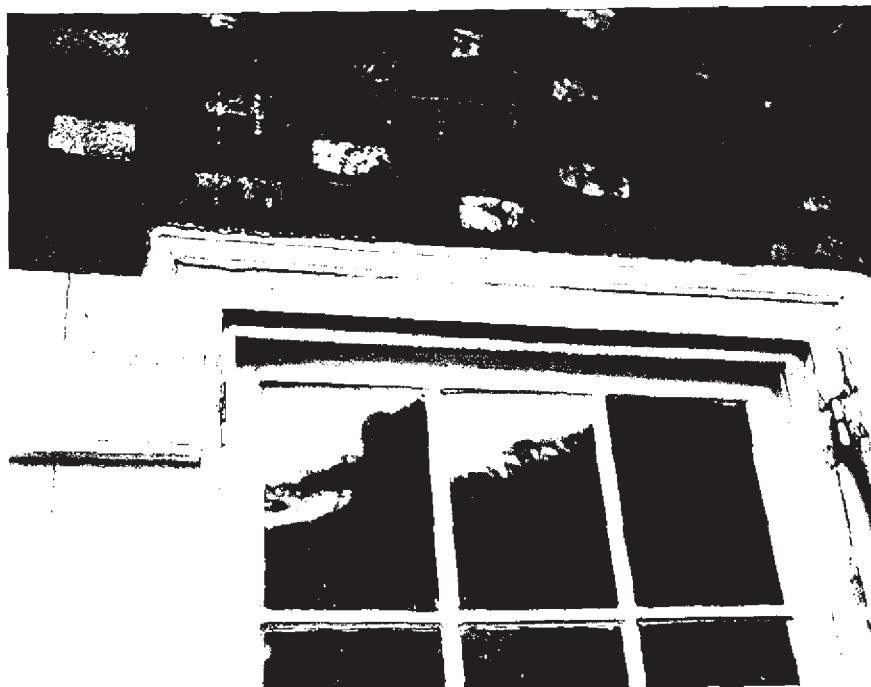
Fig. 3. West wall of north arm. Pointing above window missing, allowing water to enter.
