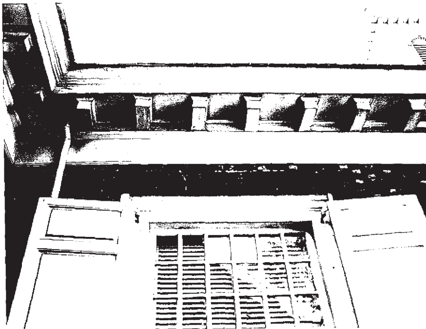
Fig. 2. Cracked lintel in north wall of west end of church.
