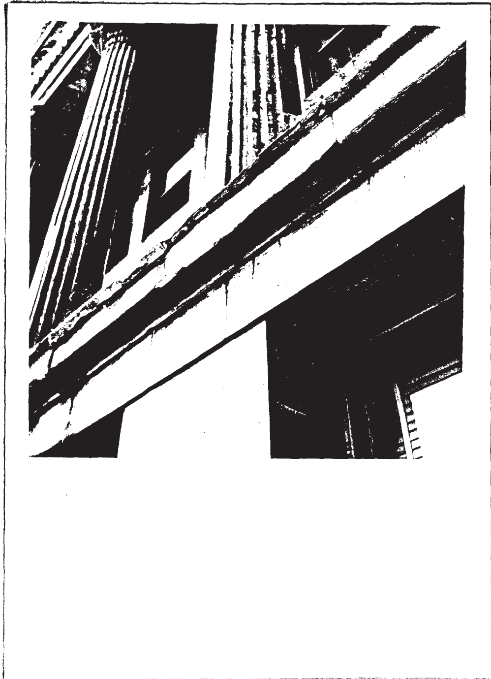
Detail of Third Street cornice at second floor. The condition of the main cornice at the roof is in similar condition.
