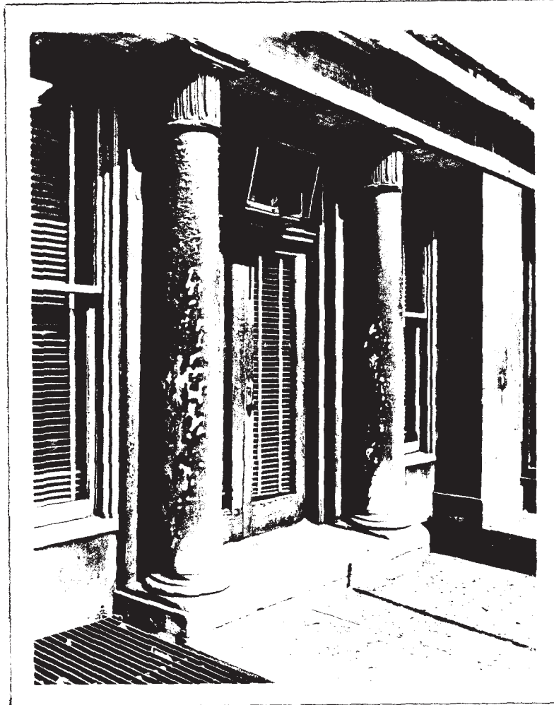
Columns along Walnut Street showing effect of dust and acid on the marble surfaces.
