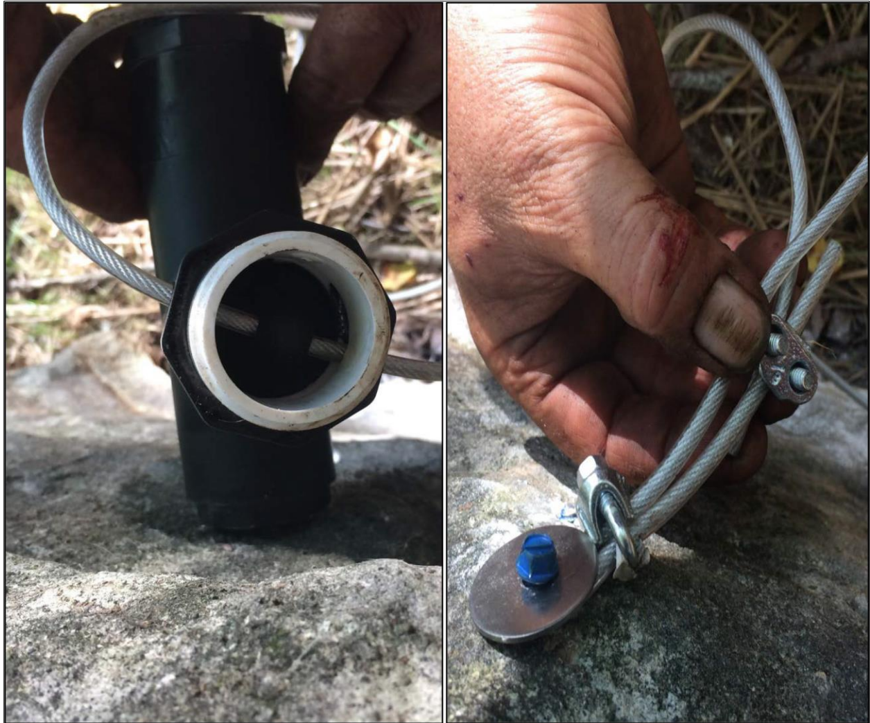
Figure SOP3-2. Concrete anchors are used to secure the stilling well at two points. One anchor point secures the stilling well and data logger (left) and the other anchor point secures a tether in case the stilling well is dislodged (right). Note these images were not taken during an installation inside a cave entrance.
