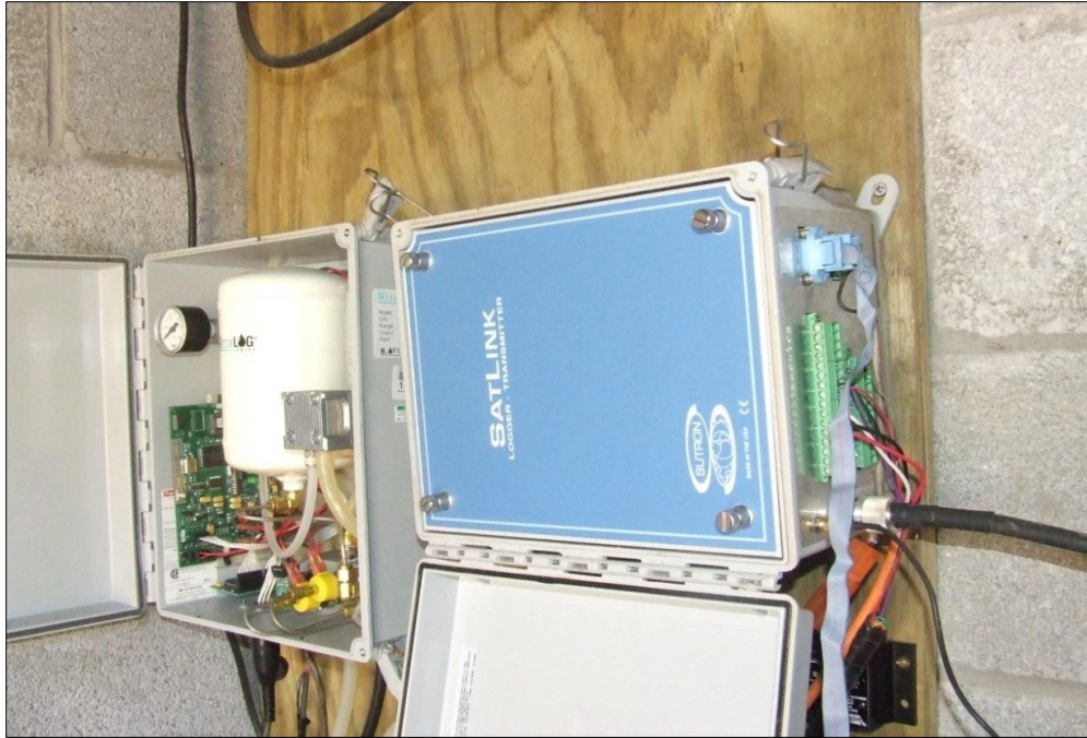
Figure SOP 6-5. Open cabinet view of Sutron Waterlogger H-355 and Satlink 2 DCP.
