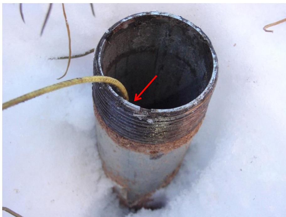
Figure 24. The measuring notch on the well casing
