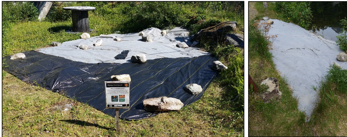
Figure 8. Photos of tarp 1 (left) and tarp 2 (right) after maintenance in 2018 at Lower Dewey Reservoir
