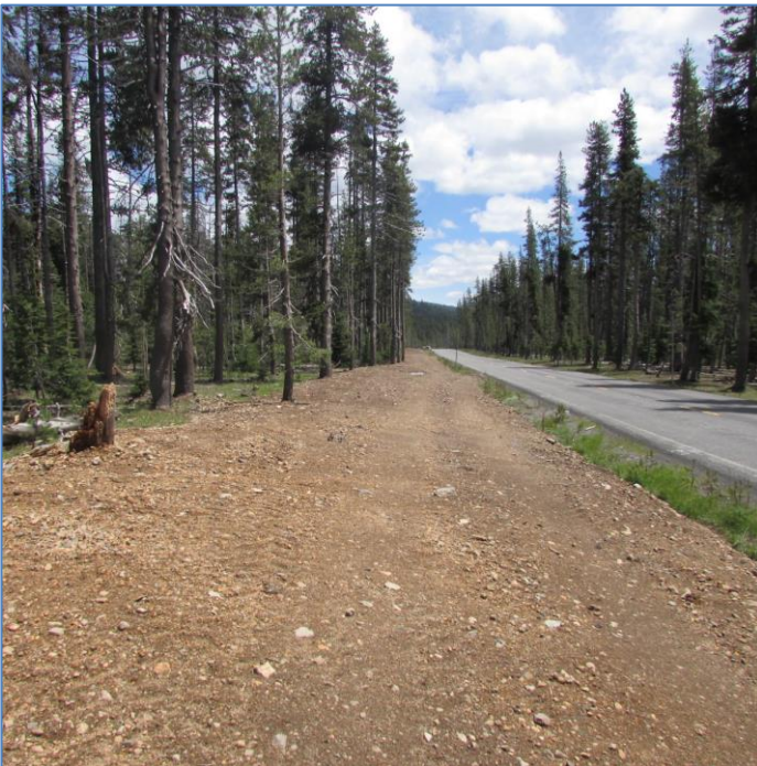
Figure 2. Roadside soil and vegetation disturbance resulting from construction of a new well and waterline. Photo by Jen Hooke.
