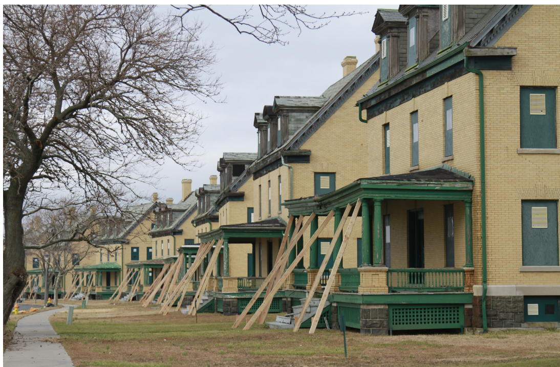
Shims support the front porches of the historic houses along Officers' Row at Fort Hancock, Sandy Hook Unit, Gateway National Recreation Area. Photo by NPS/Wickersty
