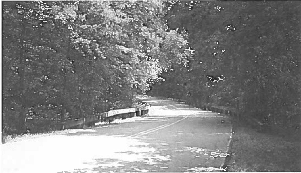
Figure 31 – Guard rails on Loop Road. (Robinson & Associates, Inc., July 28, 2005)
