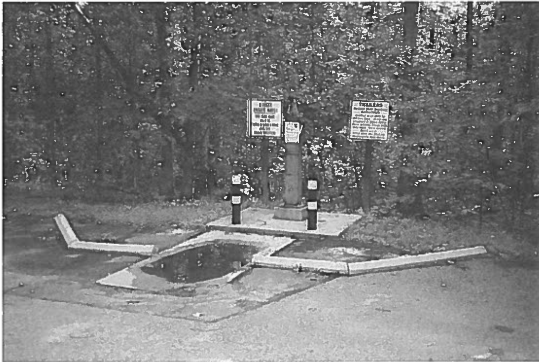
Figure 66 – Disposal Station. (Robinson & Associates, Inc., July 28, 2005.)
