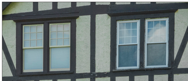
Historic 9/1 wood windows at left with replacement windows at right. Note that the historic, wood frame is narrower, providing a larger glazed opening.
