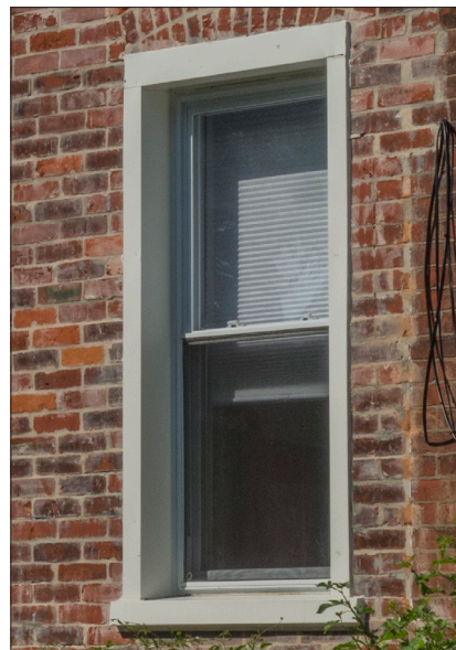
Stock replacement units may not match detailing of historic windows. Changes to the stile and rail dimensions and sill, head, casing and muntin profiles alter the appearance of a window.
