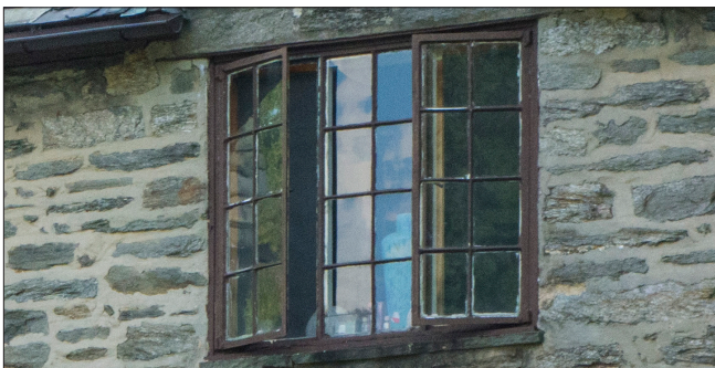
Although aluminum-clad windows can include exterior muntins, the profiles may not have the same refinement as historic windows, as seen here.
