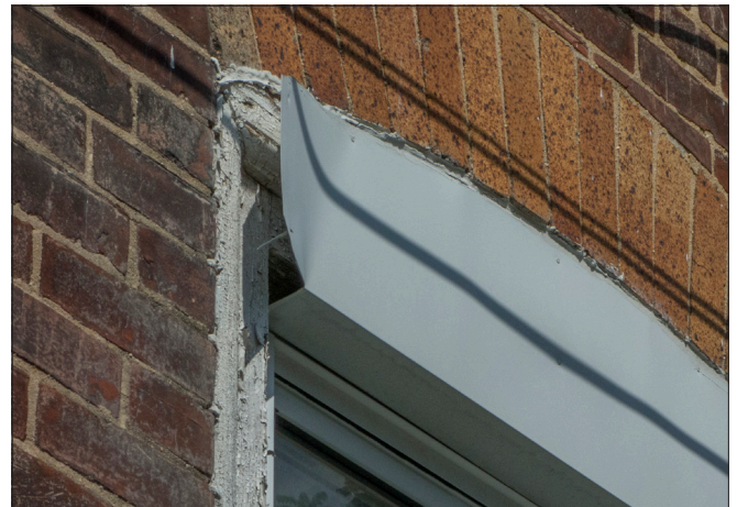
The historic wood casing and sill should be repaired and repainted. Enclosing wood elements can hide deterioration and lead to additional problems.
