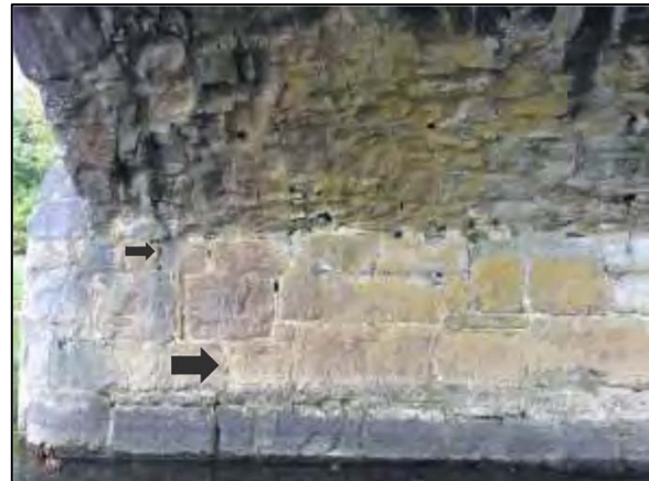
Figure 84. West Pier. Arrows indicate cracked stone. Photo: 2014 Pre-Design report.
