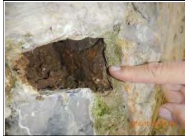
Figure 88. Missing mortar in arch barrel. Note the thin layer of pointing mortar in front of the brown sand at the back of the recess. Photo: 2014 Pre-Design report.
