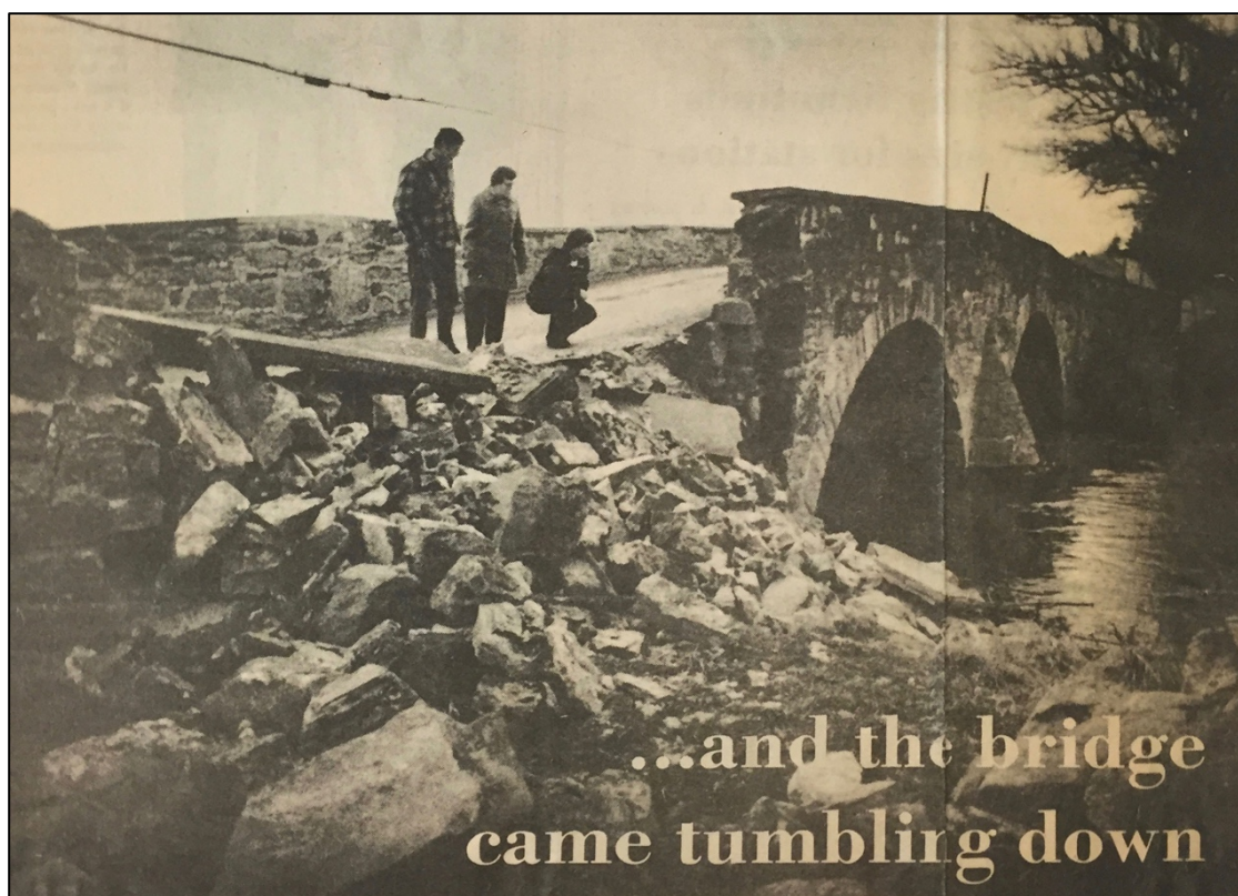
Figure 10. A wall collapses at Leitersburg bridge (also referred to as Strite's Mill Bridge in 1982. Source: Washington County Free Library, Washington County Bridges vertical file.
