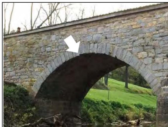
Figure 86. Arrow indicates location of slippage of ringstones on the south elevation of the west arch. No slippage has occurred in the arch’s barrel. This condition may have occurred during the original construction. Photo: 2014 Pre-Design report.
