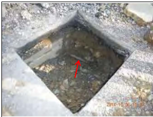
Figure 67. Test pit behind the west abutment. Arrow indicates tie bar. Note exposed surface of concrete wall on the left side of the pit. Also, note the brown color of the fill material. Photo: 2014 Pre-Design report.
