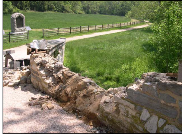
Figure 48. Severe damage on interior face looking southeast. Photo: NPS DSC eTIC No. ANTI 302 C10.
