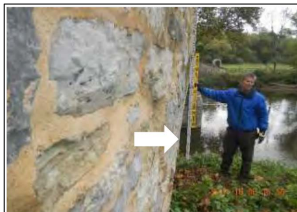
Figure 90. Checking to see if the wing wall on the south side of the West Abutment is plumb. Note the gap between the wall and the vertical survey rod at the arrow. Photo: 2014 Pre-Design report.
