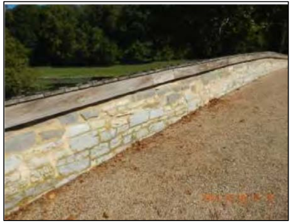
Figure 71. The deck abuts the parapet on each side of the bridge. The surface of the deck is fairly level between parapets. Water was observed to run against the northwest parapet wall during coring and during rain. Photo: 2014 Pre-Design report.
