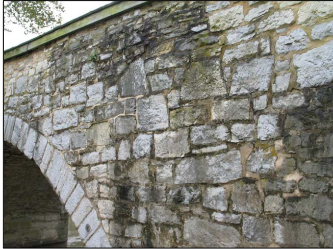
Figure 53. Condition of bulging northwest spandrel wall in 2005. Note the discoloration of the stone which is much darker near the bulge. Photo: 2005 Bridge Inspection Report, NPS DSC eTIC.
