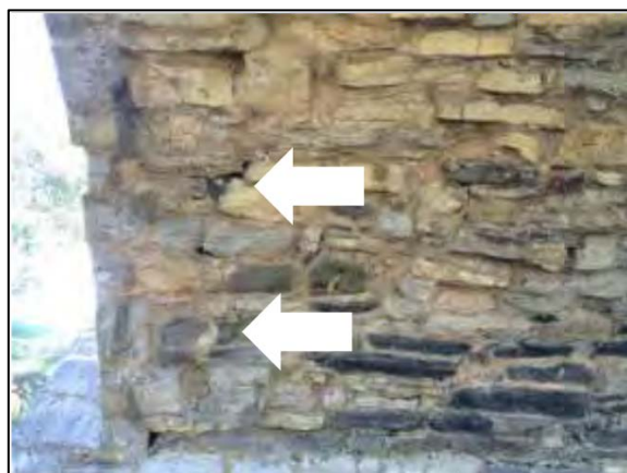
Figure 87. Barrel arch construction. The arrows indicate a crack underneath the spandrel wall. Photo: 2014 Pre-Design report.
