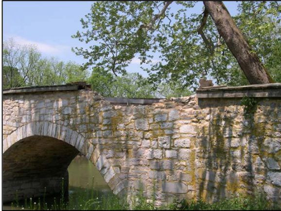
Figure 47. A witness tree limb fell and incurred damage to the bridge during 2003's Hurricane Isabel. Photo: NPS DSC eTIC No. ANTI 302 C10.
