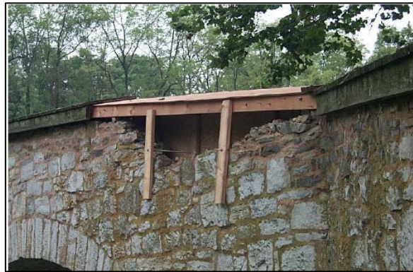
Figure 46. The park installed a temporary wood barrier at the damaged section. Photo: NPS DSC eTIC No. ANTI 302 D371.
