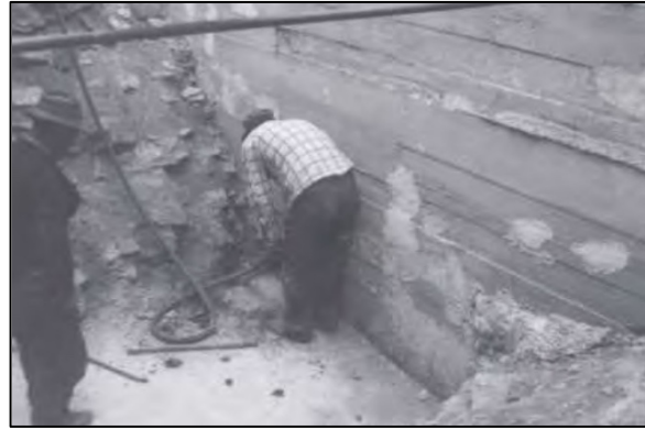
Figure 29. The 1955-56 work, seen above, included drilling holes through the arches for new weep holes. Note the condition of the back of the arch barrels. Photo: Peck Peck & Associates and McMullan & Associates Pre-Design Bridge Composition & Analysis report, 2014.
