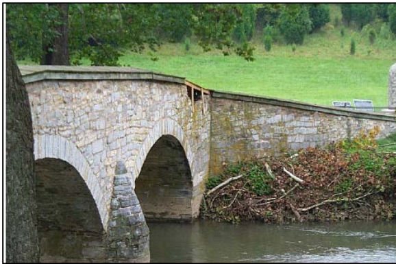
Figure 45. Damage to south spandrel wall (downstream) near east abutment. Photo: NPS DSC eTIC No. ANTI 302 D371.
