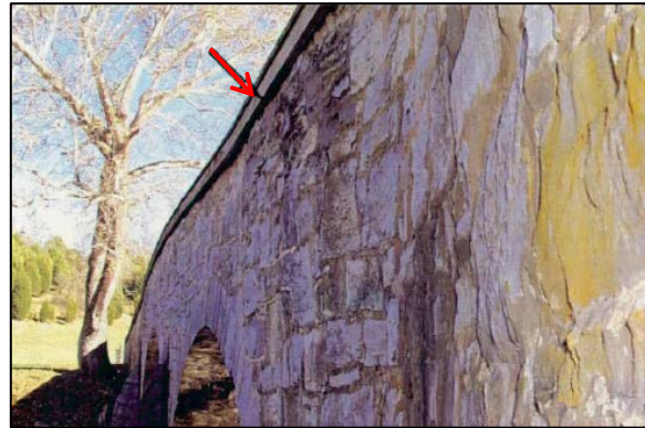
Figure 43. Bulge (arrow) in upstream side of spandrel wall noted in 2001 FHWA inspection report. Photo: NPS DSC eTIC No. ANTI 302 D37H.
