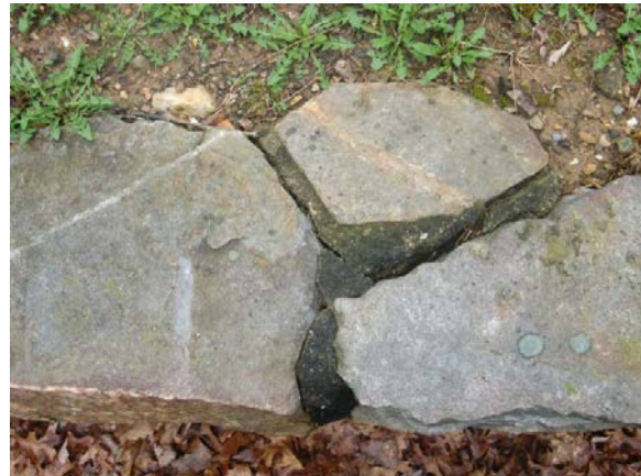
Figure 387. The rear retaining wall has degrading mortar and easily-moveable stones. Photo: HPTC (03/21/12).
