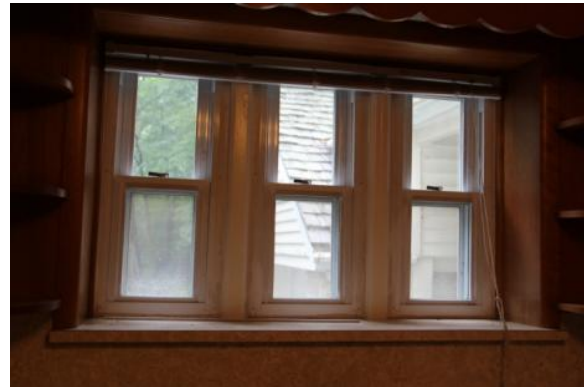
Figure 277. W128-W130 are modern vinyl replacement units. Photo: HPTC (06/12/12).
