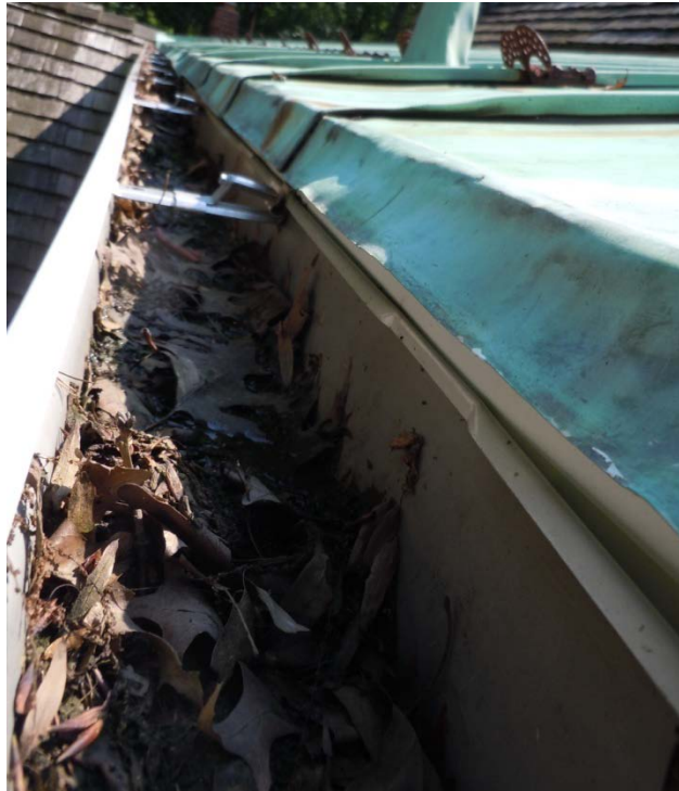
Figure 364. Vegetative debris has collected in the rear dormer gutter clogging both the gutter and the downspout. Photo: HPTC (08/29/12).
