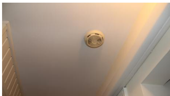
Figure 184. The battery-operated smoke detector in Room 208. Photo: HPTC (06/12/12).
