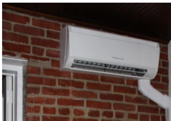
Figure 179. The mini-split unit in Room 106. Photo: HPTC (06/12/12).
