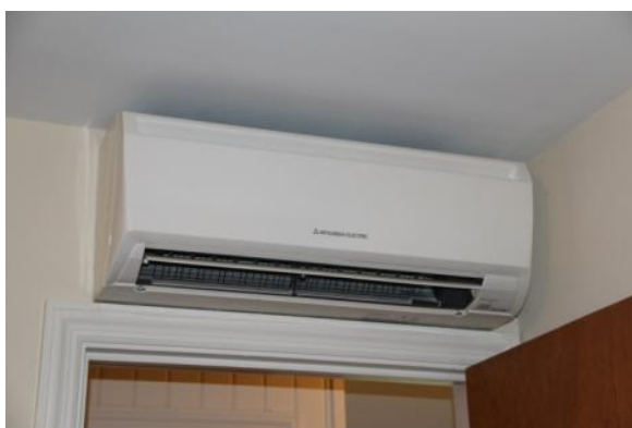
Figure 178. The mini-split unit in Room 201. Photo: HPTC (06/12/12).
