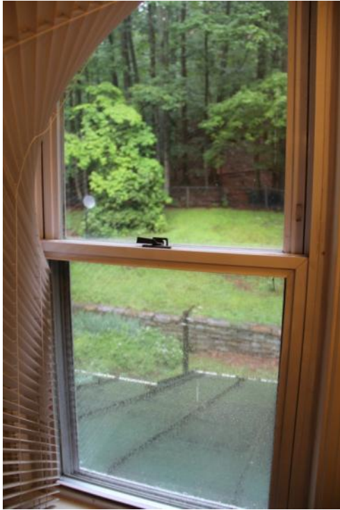
Figure 313. W206 is a modern vinyl replacement unit. Photo: HPTC (06/12/12).
