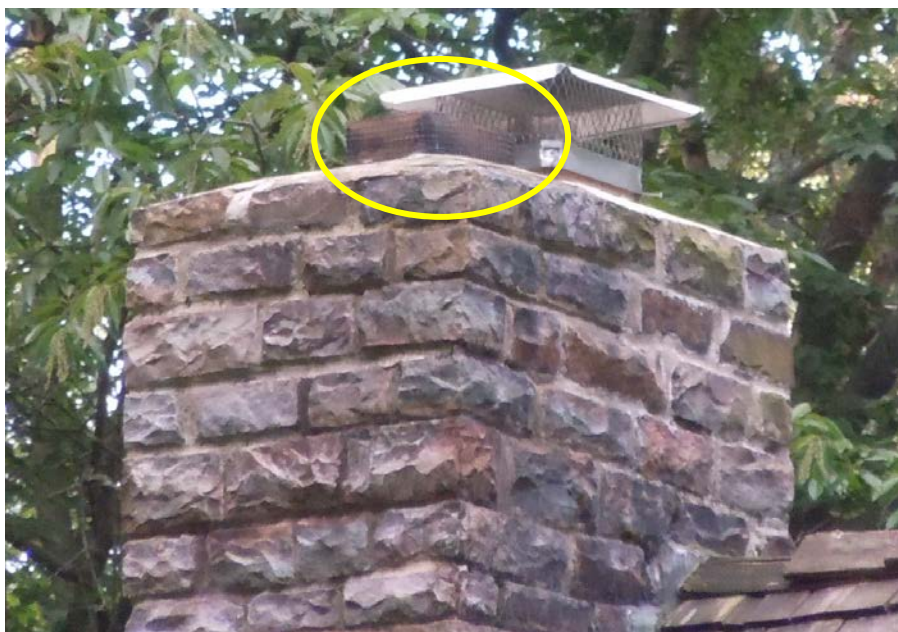
Figure 369. The eastern flue of the stone chimney lacks a chimney cap. Photo: HPTC (08/29/12).
