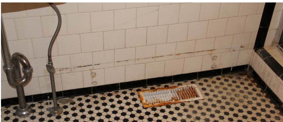
Figure 373. Rudimentary repairs were made to the ceramic wall tile in the first-floor bathroom. Note the rusty floor register due to high humidity in this area. Photo: HPTC (06/12/12).
