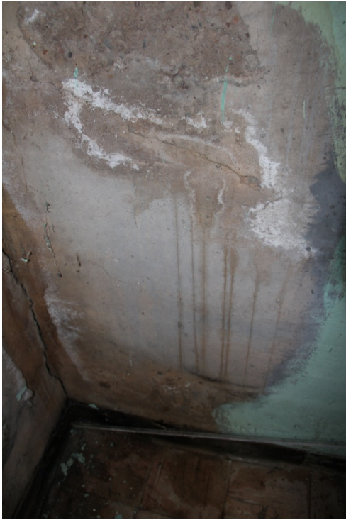
Figure 346. Cracks have formed in the concrete walls and evidence of seeping water can be seen. Photo: HPTC (06/20/12).
