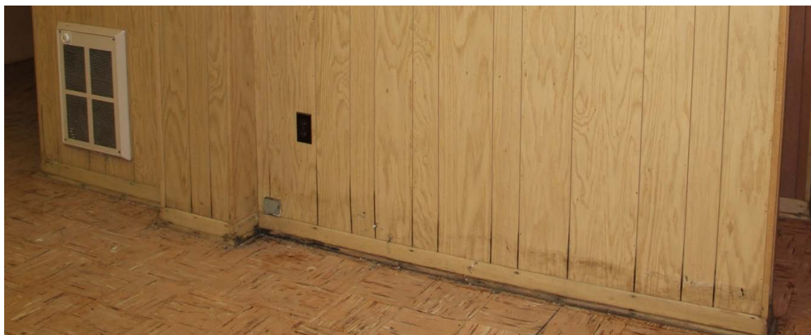
Figure 375. Water staining and bio-growth on the lower foot of the basement paneling. Photo: HPTC (06/20/12).
