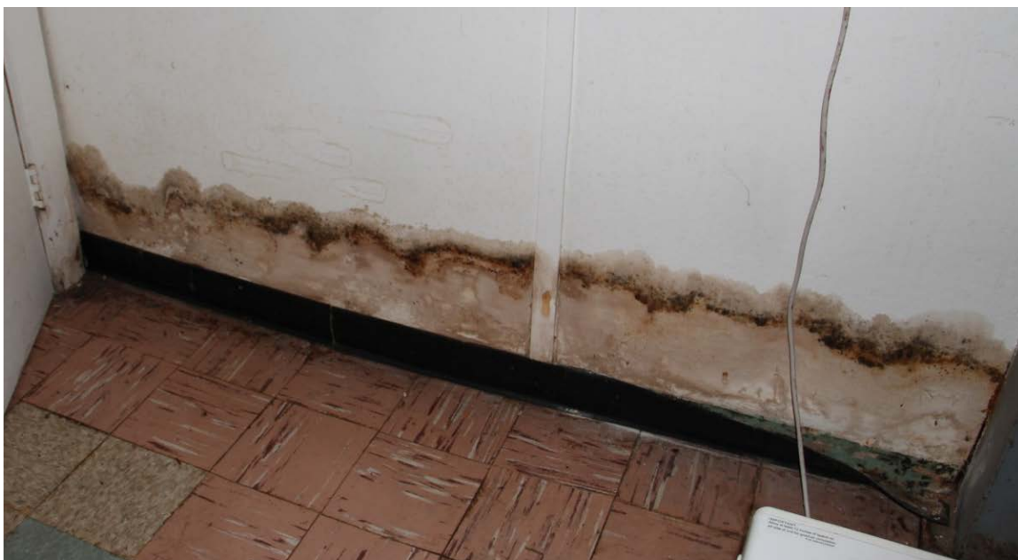
Figure 372. Water staining and bio-growth on the lower foot of the basement wallboard. Photo: HPTC (06/20/12).
