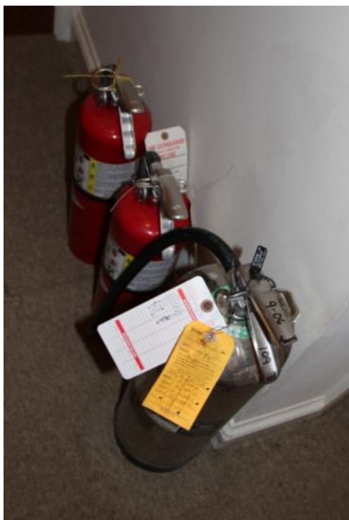
Figure 182. The three fire extinguishers for Quarters 1 need to be redistributed throughout the building. Photo: HPTC (06/12/12).
