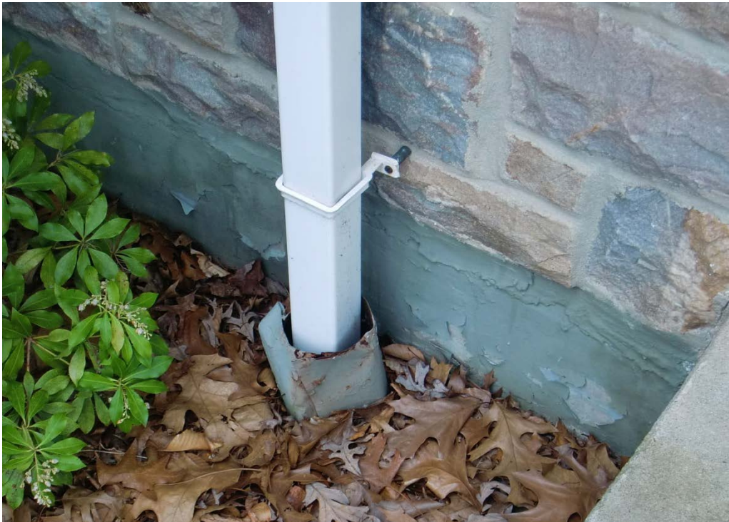
Figure 363. The extent of the underground drainage system at Quarters 1 is unknown. Photo: HPTC (03/21/12).
