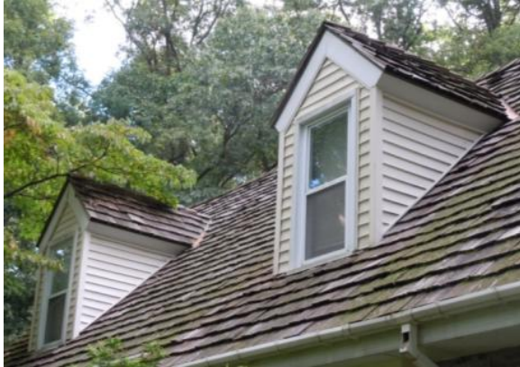
Figure 141. No flashing can be seen at the front dormers. Photo: HPTC (08/29/12).
