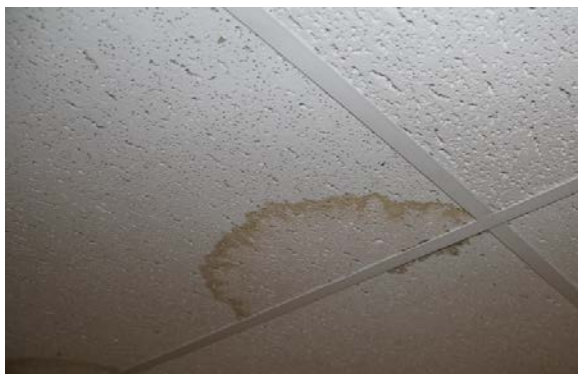
Figure 381. A water stain on an acoustical ceiling tile in Room 001. Photo: HPTC (06/20/12).
