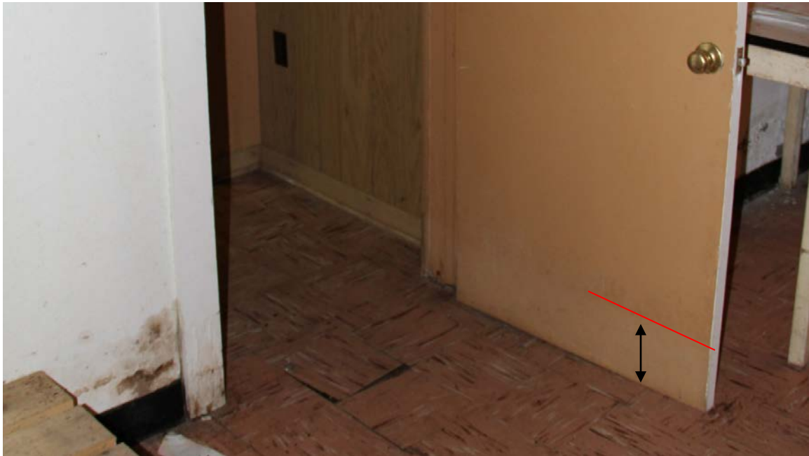
Figure 370. Water staining on the lower portion of a basement door. Arrow indicates level of rising damp on virtual surfaces. Photo: HPTC (06/20/12).
