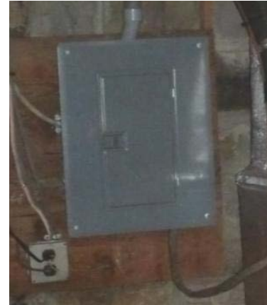
Figure 187. A modern subpanel is located in the basement. Photo: HPTC (03/21/12).
