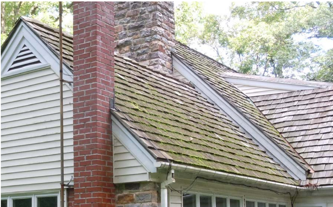
Figure 360. The eastern slope of the sun porch cedar roof exhibits biological growth. Photo: HPTC (08/29/12).
