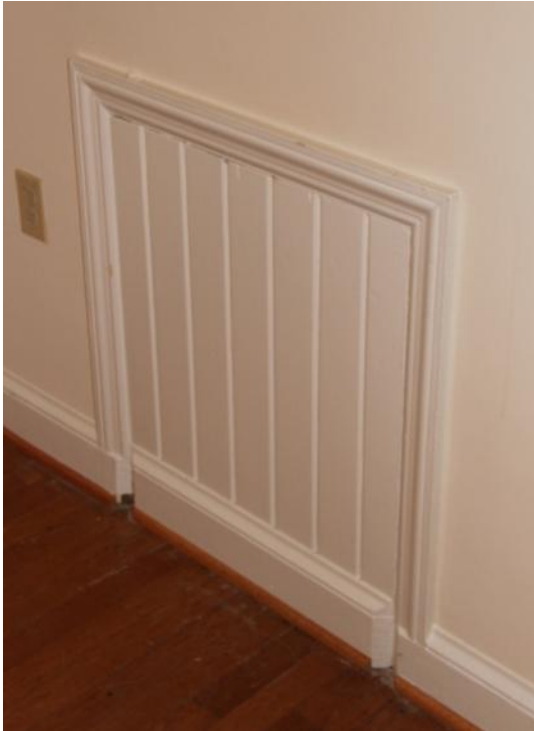
Figure 291. D201A accesses the bathtub plumbing. Photo: HPTC (06/12/12).
