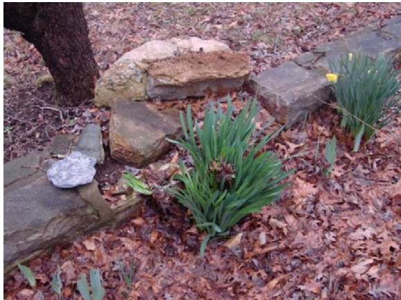
Figure 386. The front retaining wall has dislodged stones and is partially overgrown with vegetation. Photo: HPTC (03/21/12).
