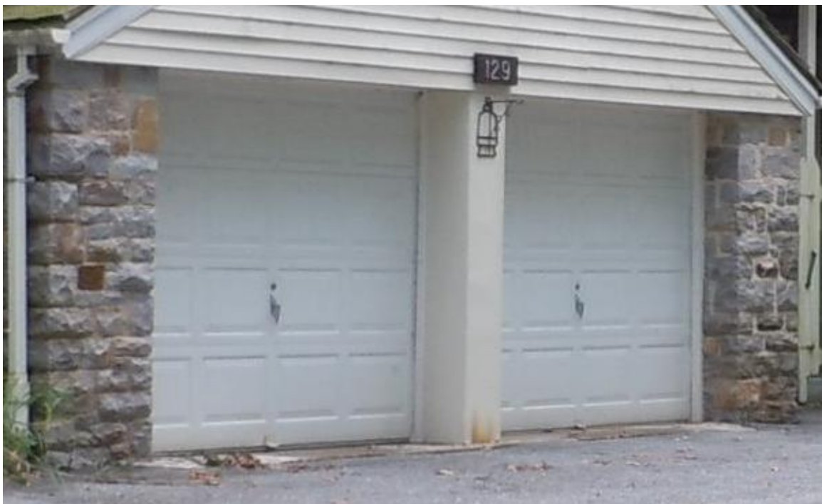
Figure 131. The overhead garage doors were replaced with sixteen-panel steel doors which are not character-defining features (DG101 and DG102). Photo: HPTC (08/29/12).
