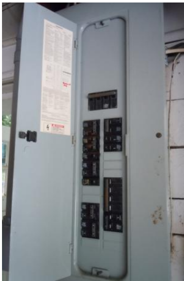
Figure 185. The main electrical panel is located in the garage. Photo: HPTC (07/17/12).
