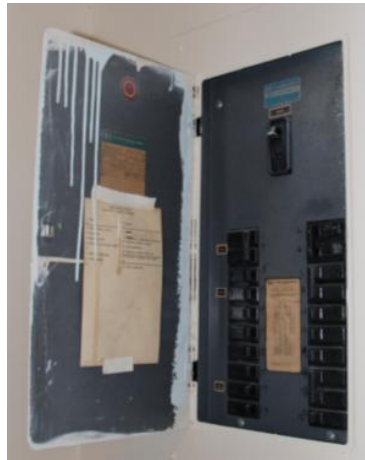
Figure 186. An original subpanel is located in the kitchen. Photo: HPTC (06/12/12).
