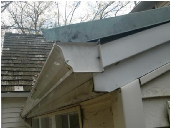
Figure 147. The aluminum drainage system on the east elevation of the breezeway. Photo: HPTC (04/21/12).
