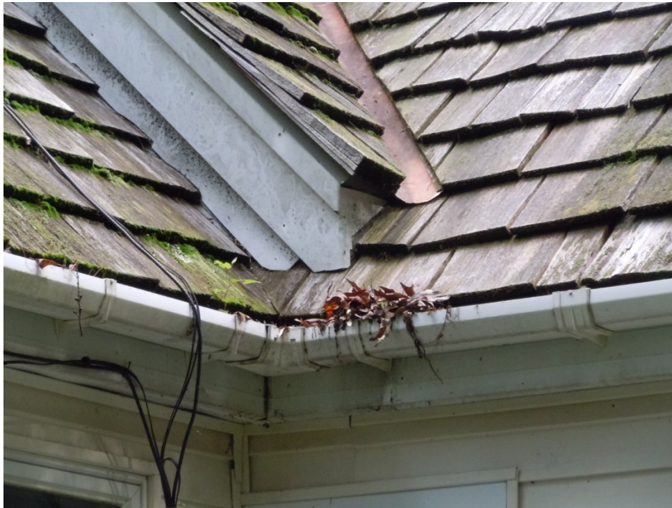
Figure 365. Vegetative debris has accumulated in the gutters of the eastern ell. The U-shaped gutters are not considered to be character-defining features. The size of the gutter is also significantly smaller and cannot carry the rain runoff from this roof. Note communications cables hung from the building – it should be determined if these are active; if not they should be removed, if they are they should be rerouted through the building in an unobtrusive manner. Photo: HPTC (08/29/12).
