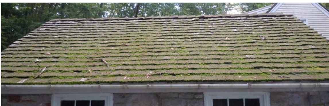
Figure 362. The cedar shakes on the garage gable roof exhibit a large amount of biological growth. Photo: HPTC (08/29/12).
