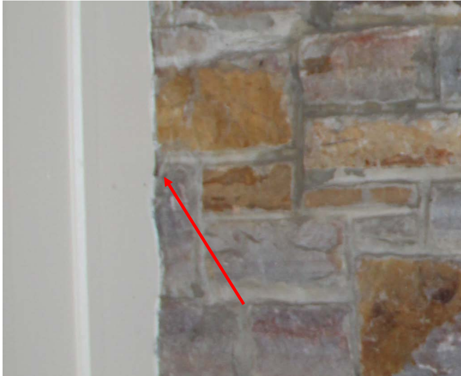
Figure 376. The "masonry seam sealant" between the stone wall and the wood wall is known to contain asbestos and is in poor condition. Photo: HPTC (06/12/12).
