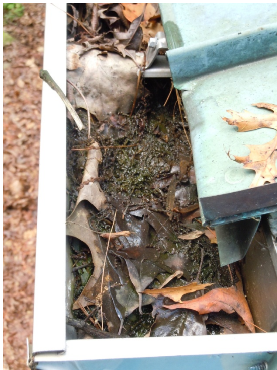
Figure 366. The accumulation of vegetative debris in a gutter at the breezeway roof has caused the retention of water in the system. Photo: HPTC (08/29/12).
