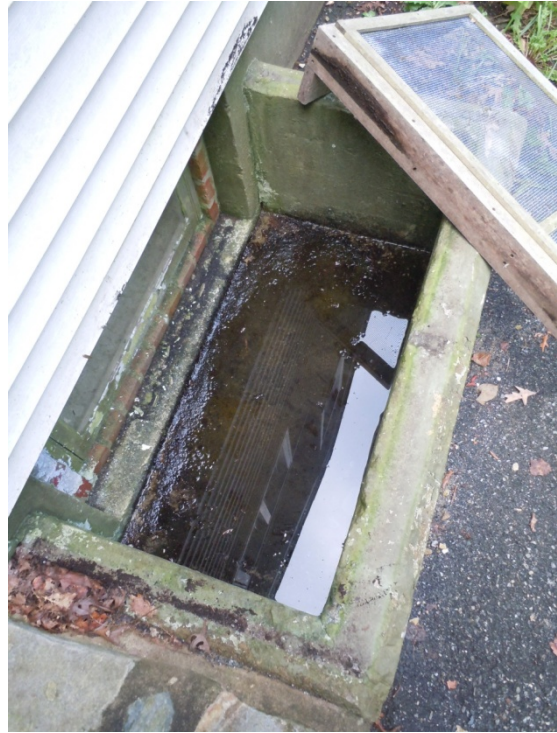
Figure 347. Water is being retained in the well of W001 adjacent to the northwest corner of Room 001. Photo: HPTC (08/29/12).
