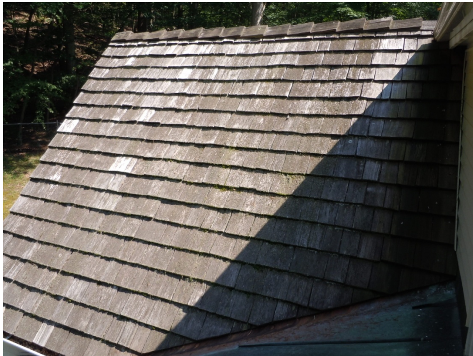
Figure 359. The northern slope of the eastern ell cedar roof exhibits warped and weathered shakes nearing the end of their lifespan. Photo: HPTC (07/17/12).
