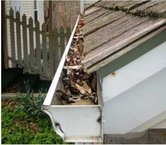
Figure 367. Collected vegetative debris can be seen in the garage roof gutters. Photo: HPTC (08/29/12).
