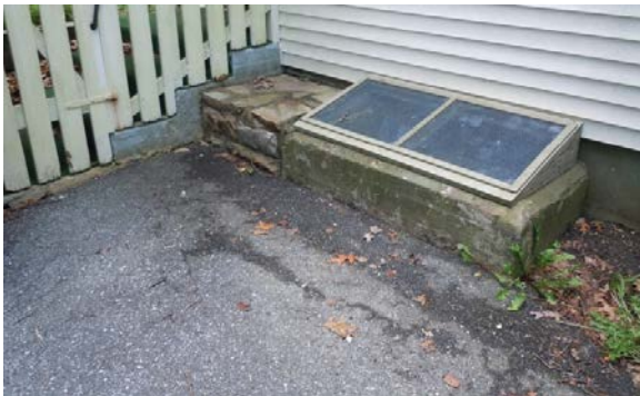
Figure 348. The mostly-paved area around the well of W001 and the stone structure in the corner is causing the retention of water at the northeast corner of Room 001. Photo: HPTC (08/29/12).
