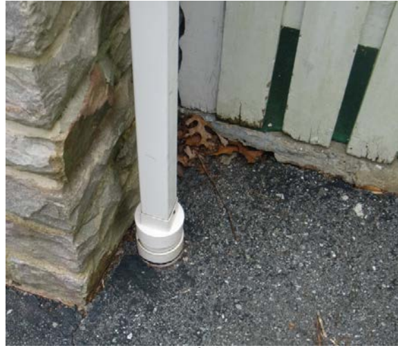
Figure 368. The extent of the underground drainage system at Quarters 1 is unknown. Photo: HPTC (08/29/12).
