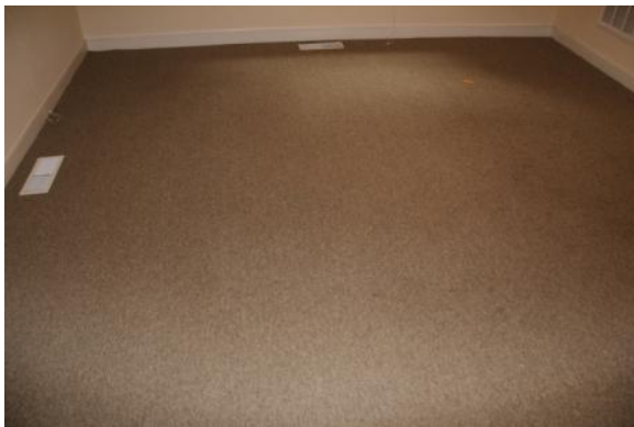
Figure 236. Carpet covers the floor of Room 101. Photo: HPTC (06/12/12).
