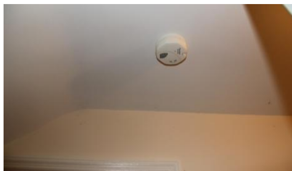
Figure 183. The battery-operated smoke and carbon monoxide detector in Room 110. Photo: HPTC (06/12/12).
