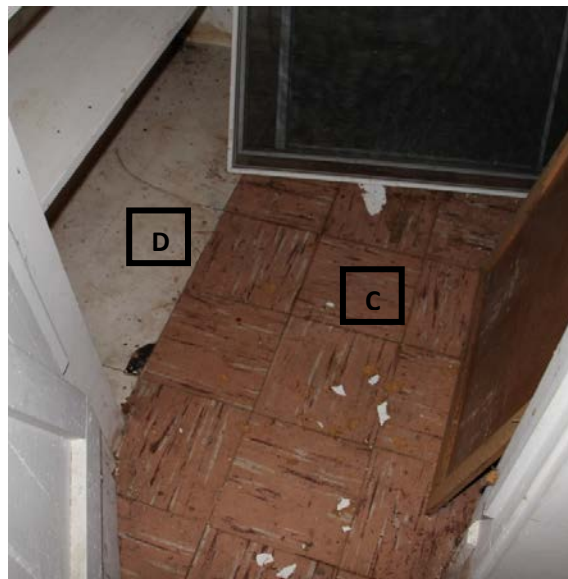
Figure 380. The white vinyl floor tiles (D) also contain asbestos. Photo: HPTC (06/20/12).
