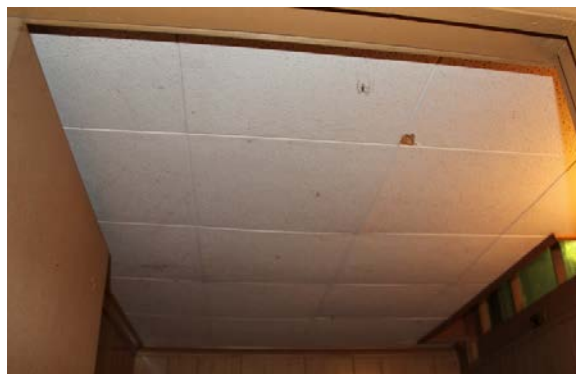
Figure 382. Acoustical ceiling tiles in Room 002 are pulling away from the substrate. Photo: HPTC (06/20/12).
