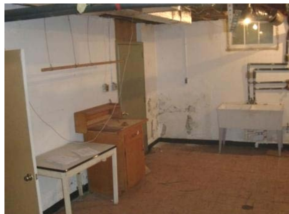
Figure 75. In Room 004, the north wall (left) was rebuilt after the fire and the east wall was reused. Photo: HPTC (04/21/12).
