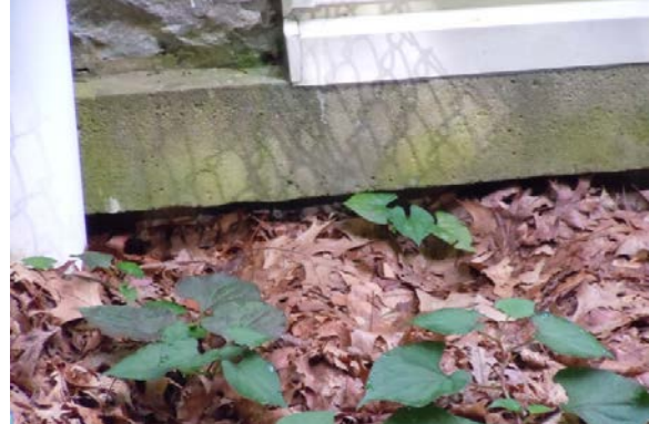
Figure 351. The sun porch concrete slab is mostly hidden by vegetative growth on the exterior. Photo: HPTC (03/21/12).
