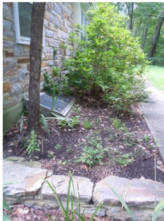
Figure 201, right. The front planting bed includes plantings which are very close to the foundation. Photo: HPTC (08/29/12).
