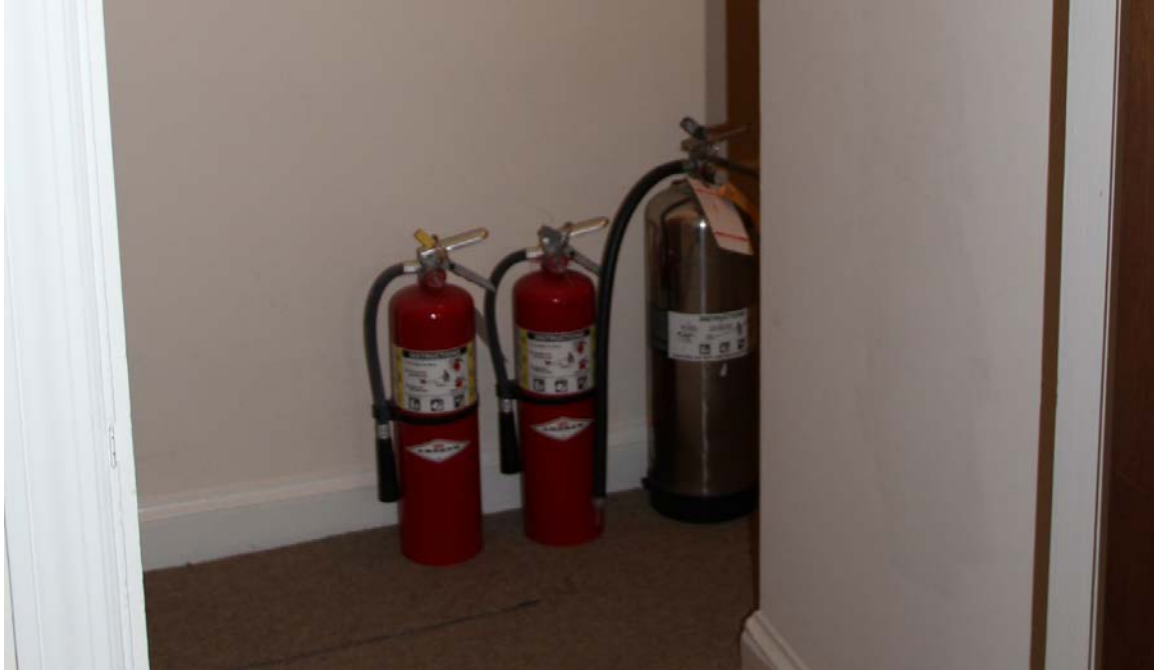
Figure 383. The fire extinguishers were not redistributed throughout Quarters 1 after they were last serviced. Photo: HPTC (06/12/12).
