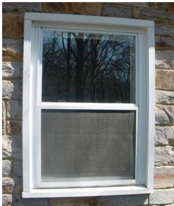
Figure 113. The dining room windows have been replaced with vinyl-clad units. Note lite patterns do not match. Photo: HPTC (04/21/12).
