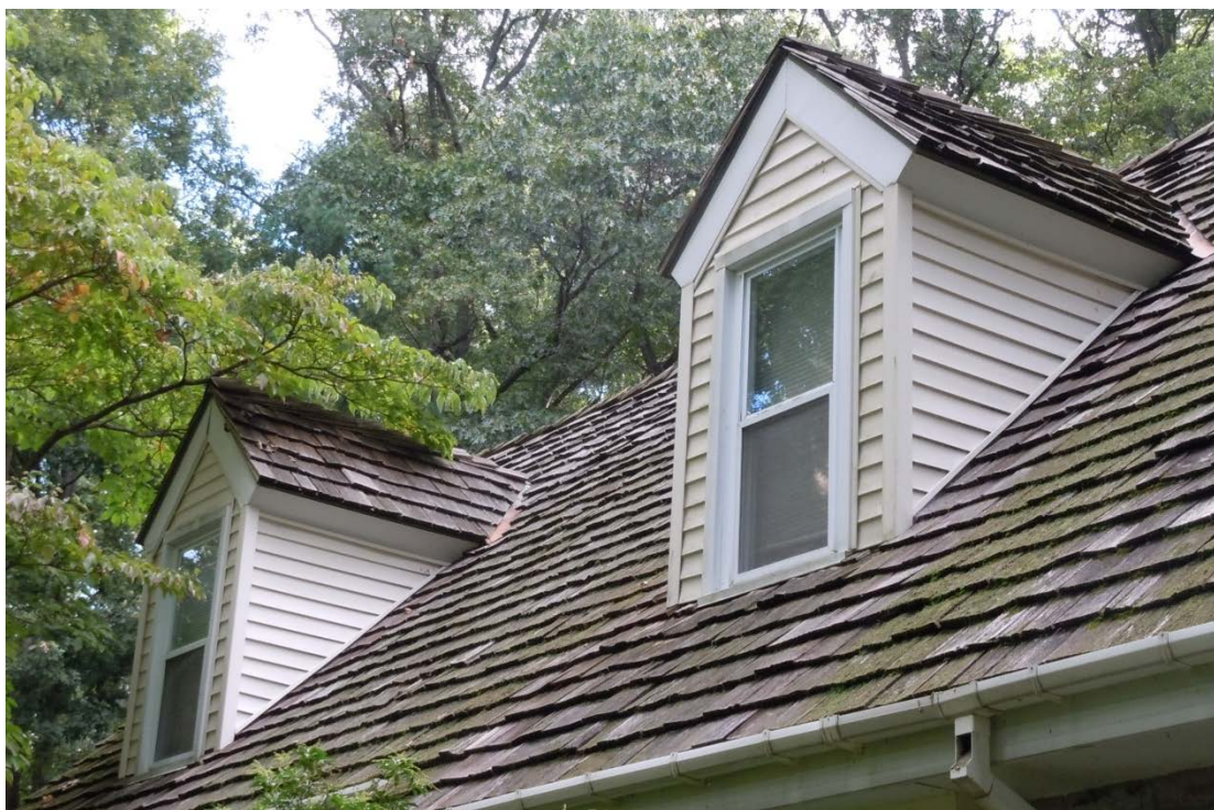
Figure 358. The cedar shakes of the main block hipped and gable roofs have neared the end of their useful lifespan. Note the overhanging vegetation that should be cut away from the building. Photo: HPTC (08/29/12).
