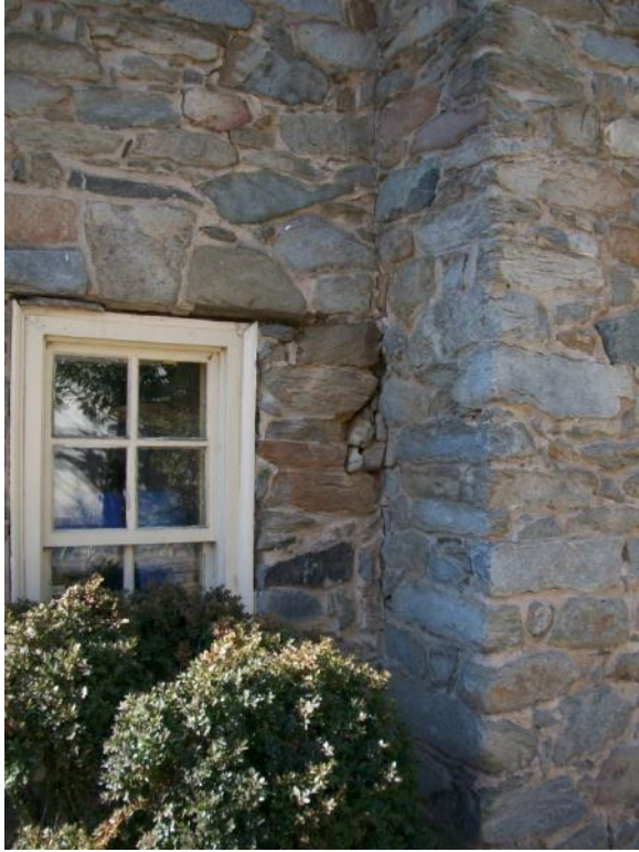
Figure 90. A crack runs along the junction of the chimney and the exterior wall. (NPS, 2012)
