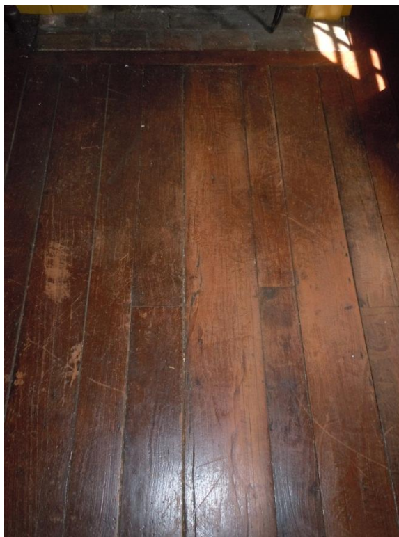
Figure 205. Random-width wood floor in Room 304; scratches can be seen across the surface. (NPS, 2013)
