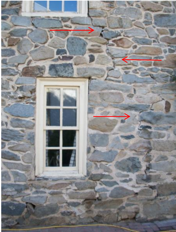
Figure 86. The east elevation of the north addition exhibiting a long crack, starting at the lower corner of W207 and running to the foundation, prior to repointing. (NPS, 2012)
