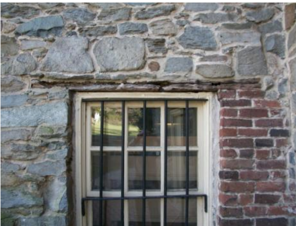
Figure 84, above. W103 degraded lintel and mortar above prior to rehab work. (NPS, 2012)
