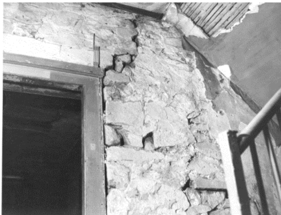
Figure 69. Open mortar joints ready for repointing in Room 201B. (NPS, 1957)
