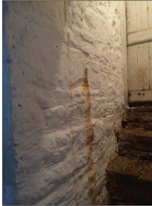
Figure 67: Water staining in basement wall, room 001.
