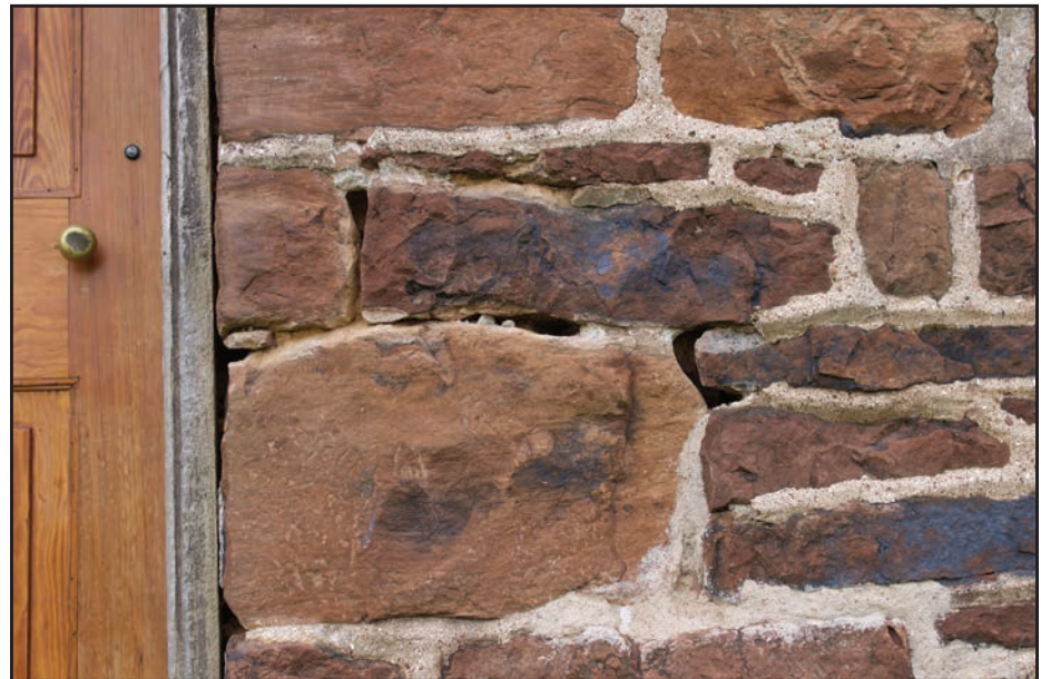
Figure 69: North elevation detail – mortar lost.
