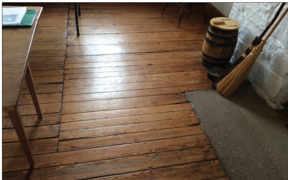
Figure 84: Evidence of wood floor replacement after basement fire, Tavern Room, 104.
