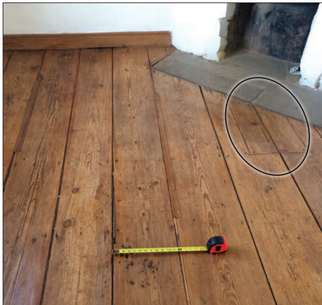
Figure 87: Floor in Bedroom 203. Note 12" width boards. Location of former vent register is circled.
