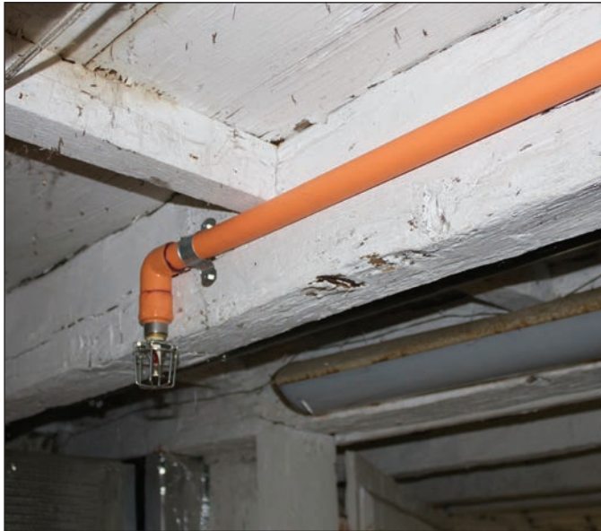
Figure 128: Sprinkler head in basement.
