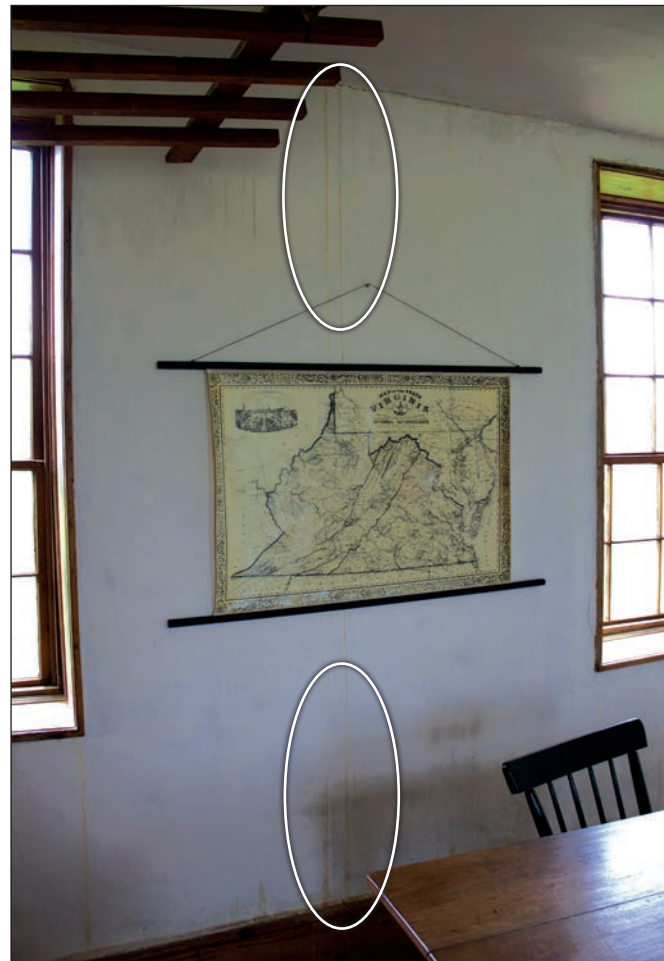
Figure 66: Water staining in room 104.
