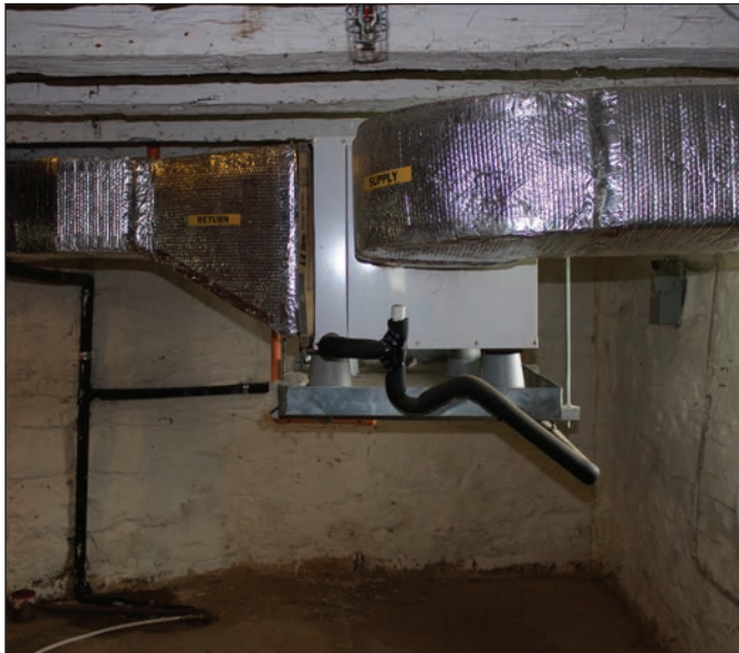
Figure 126: HVAC Distribution system in the basement.
