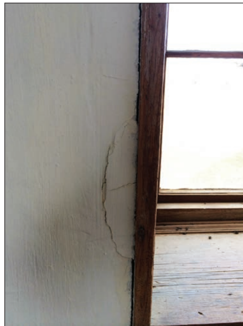
Figure 123: Plaster delaminating around first floor window.
