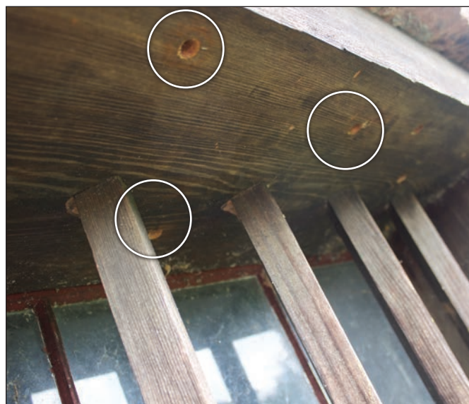
Figure 76: South elevation upper frame – window 002—carpenter bee damage.
