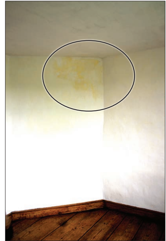
Figure 64: Water staining in room 302.
