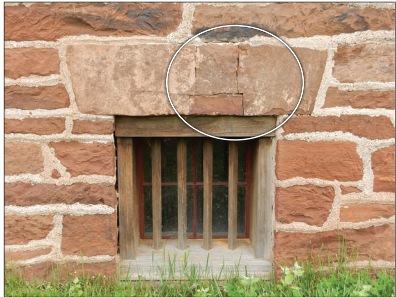
Figure 73: Fractured lintel, window 005.
