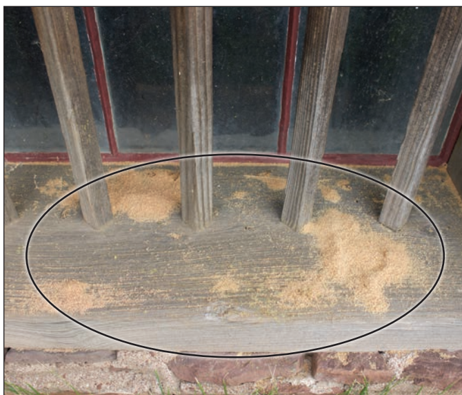
Figure 75: South elevation – window 002—sawdust accumulation.
