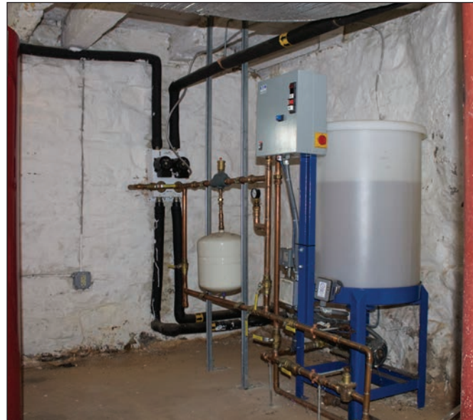
Figure 127: Geothermal heat pump in the basement.
