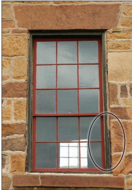
Figure 93: Window 101, first floor, south elevation. Lost mortar flashing (circled).
