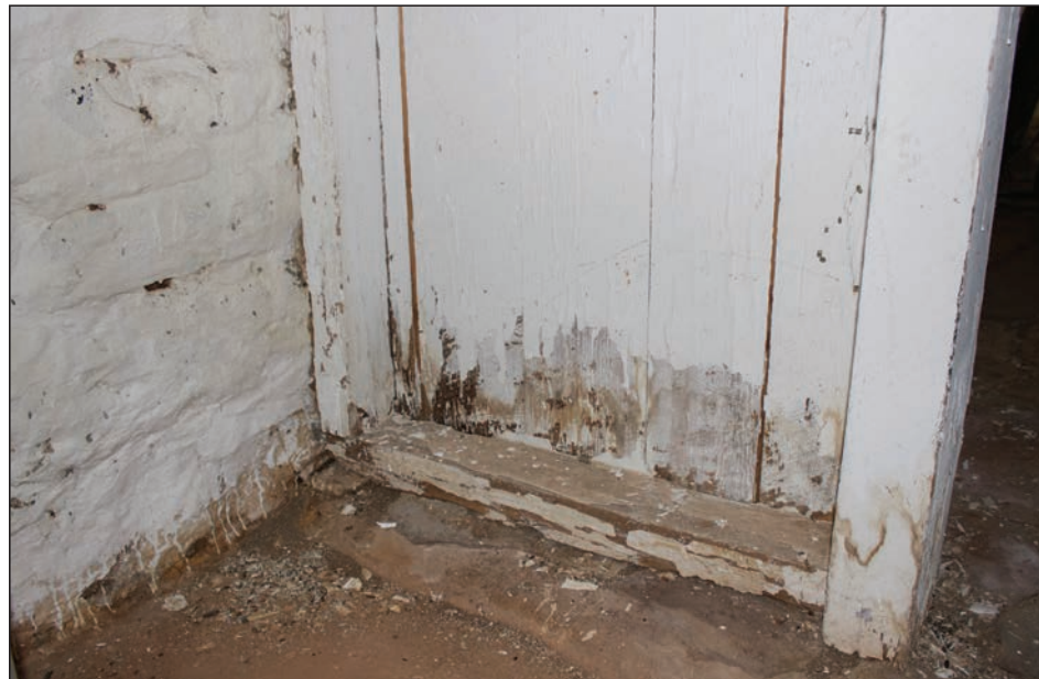
Figure 116: Rising damp on the basement partition wall.
