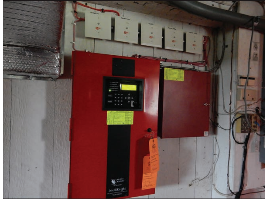
Figure 131: Fire alarm enunciation panel.
