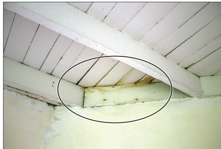
Figure 65: Water staining in room 303.
