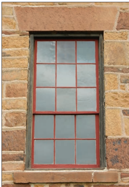
Figure 96: Window 103, first floor, south elevation. Lost mortar flashing.
