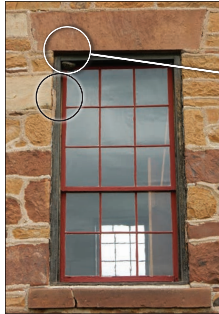
Figure 94: Window 102, first floor, south elevation. Only remaining mortar flashing (circled).
