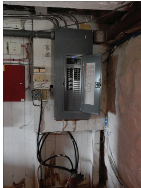
Figure 133: Main electrical distribution panel.
