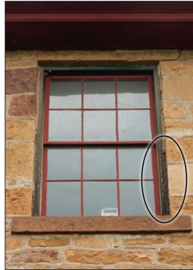
Figure 102: Window 202, second floor. Incomplete mortar flashing (circled).
