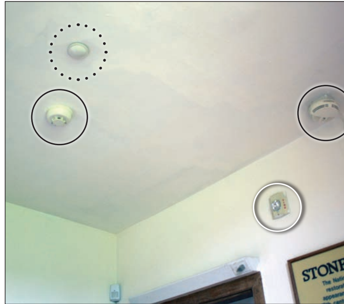
Figure 129: Fire alarm light indicator (white circle), smoke detectors (black circles) and sprinkler (dotted circle) in the dining room.
