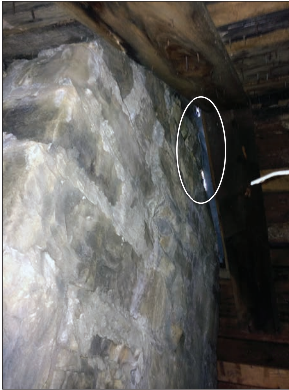
Figure 63: Daylight between roof and east chimney.
