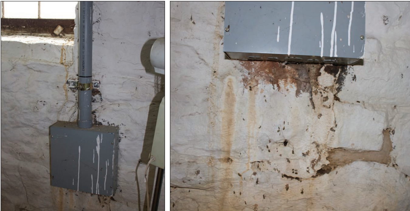
Figure 79: Electric junction box mounted on south wall of the basement, east side, 002.
