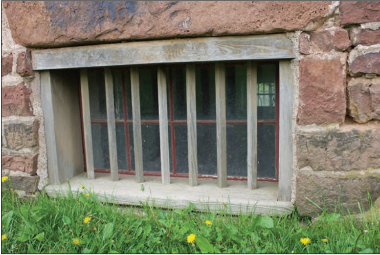
Figure 70: North elevation, window 004 – mortar lost.
