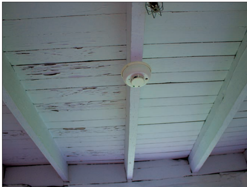
Figure 125: Ceiling of Bedroom 303. West side paint is peeling, east side is not.
