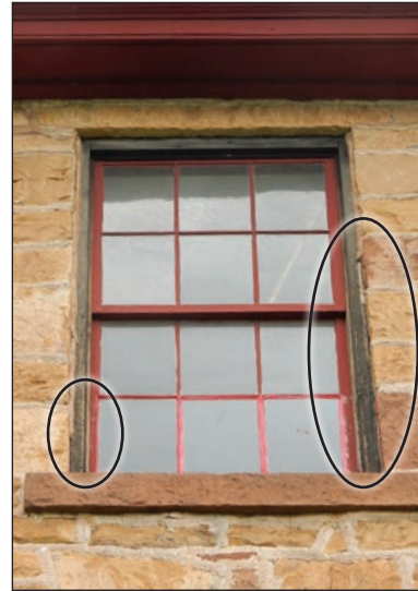
Figure 103: Window 203, second floor. Incomplete mortar flashing (circled).
