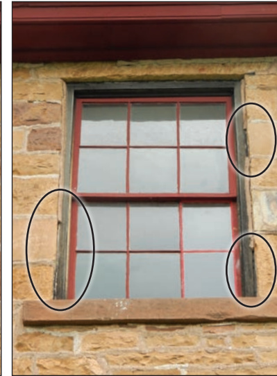
Figure 104: Window 204, second floor. Incomplete mortar flashing (circled).
