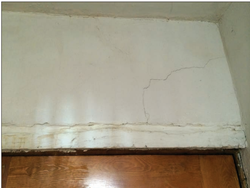
Figure 122: Plaster cracking around rear entrance door 101B.
