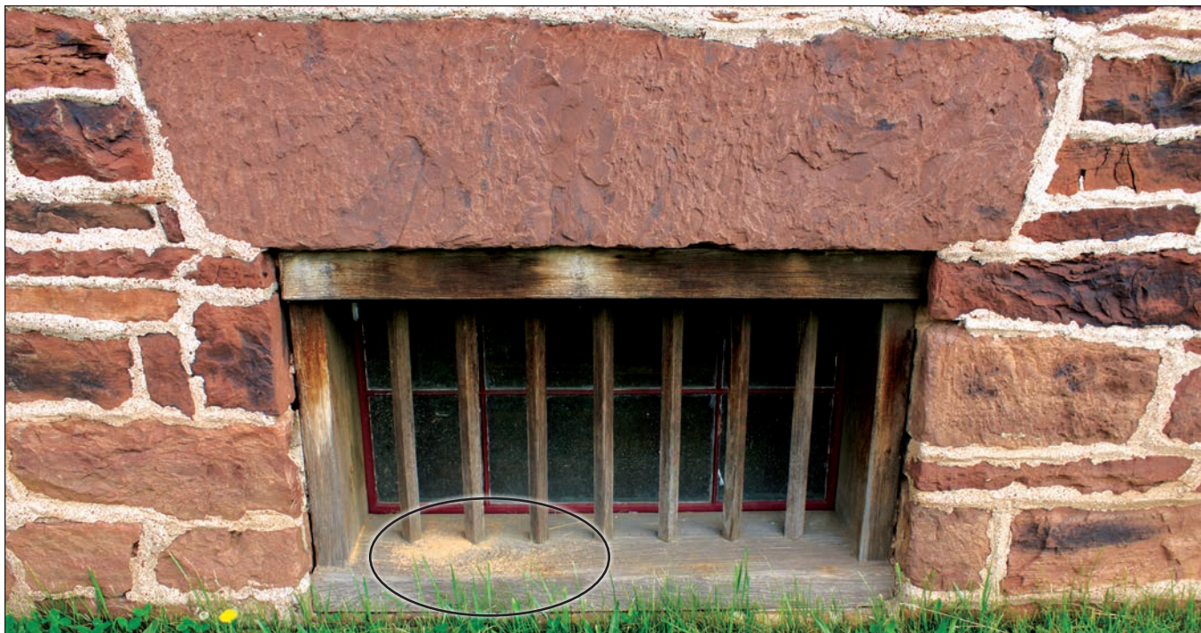
Figure 74: South elevation – window 001—sawdust accumulation.
