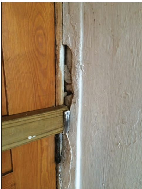
Figure 124: Plaster delaminating around rear entrance door 101B.
