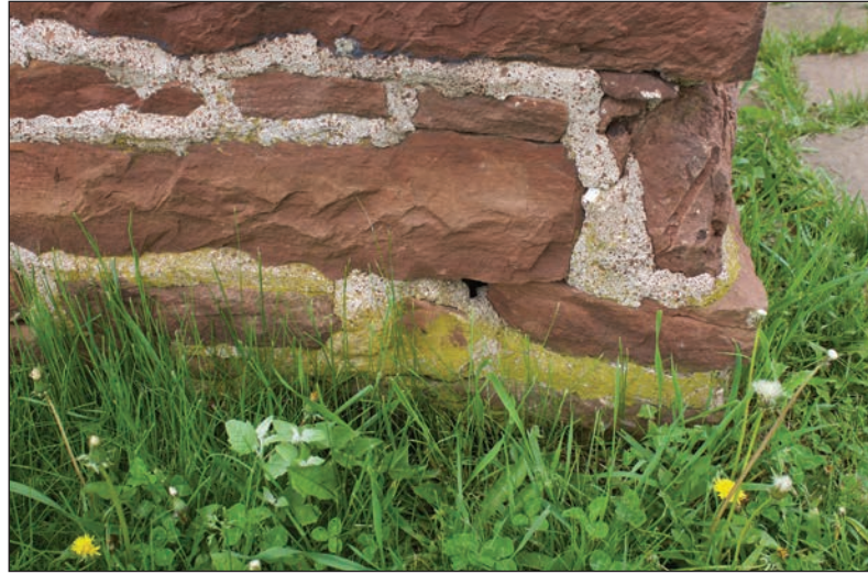
Figure 71: Northwest corner – mortar lost.
