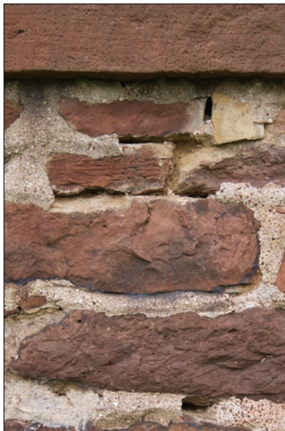
Figure 68: North elevation detail – mortar lost.
