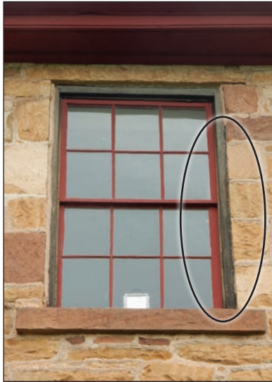
Figure 101: Window 201, second floor. Incomplete mortar flashing (circled).
