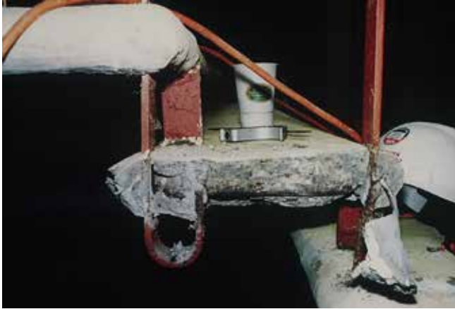
Figure 3: Failed patches at the stairs to the stream
