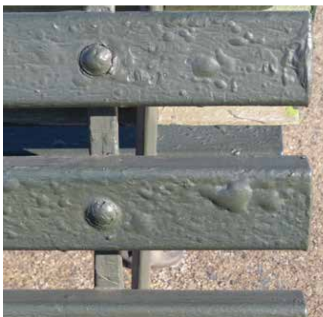
Figure 4: Bubbling and blistering paint on bench slats. Photograph by author
