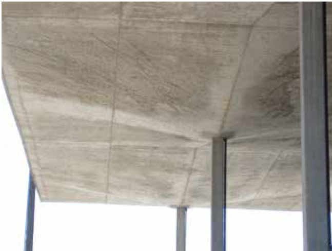
Figure 8: Grant County Fairground Grandstand, Shell discoloration. Photo by the author, 2014
