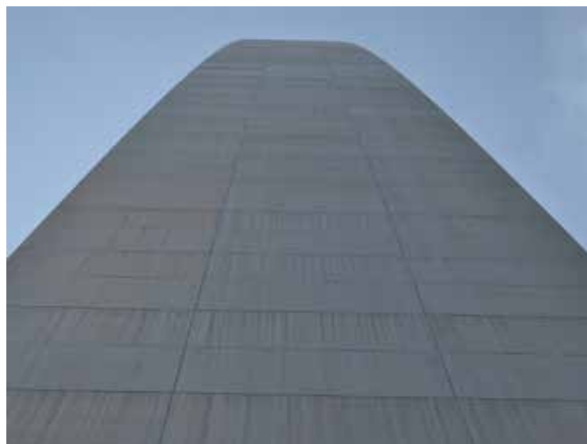
Figure 4. Deposits from run off from horizontal welds
