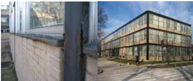
Figures 8, 9: Wishnick Hall deterioration (left); Wishnick Hall, 2009 (right)
