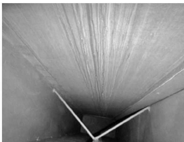
Figure 16: Image looking upward into the interstitial spaces. The water streak orientation reveals that they were formed after the segment was set in place, but there are no signs of active water leaking.
