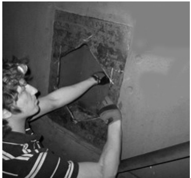
Figure 14: One of the hexagonal openings in the carbon steel skin.
