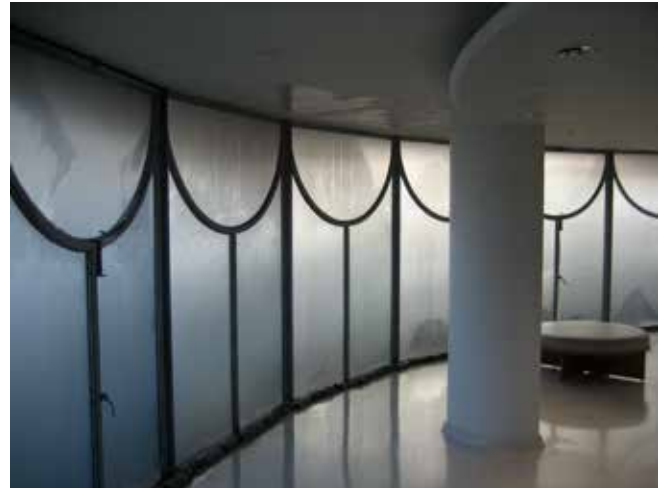
Figure 4: Extreme condensation on the window-walls of the Guggenheim's Thannhauser Pavilion obscured the connection of the building to Central Park. (Photo by Angel Ayón.)
