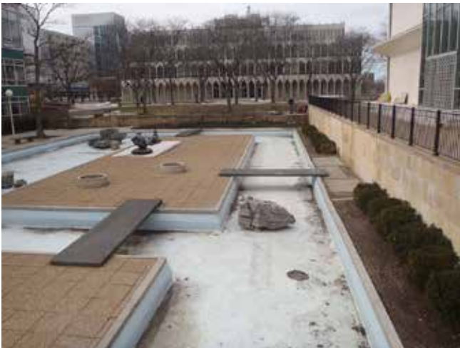
Figure 14: McGregor Center, Detroit, Michigan. Prior to restoration, pools had been coated light blue and brown pavers installed on the islands and surrounding walks. QEA, 2011
