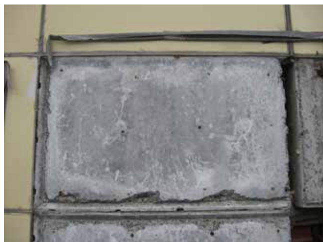
Figure 6: Panels where the metal panel has sheared away from the concrete
