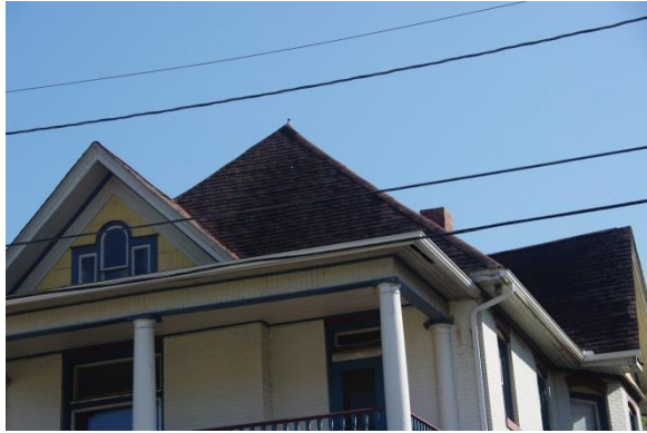
Irregular Roof Line
