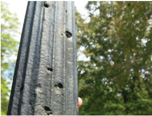
Figure 72: Detail of holes and pock-marks in cast iron shaft, 25 September 2017.
