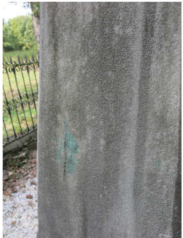
Figure 57. Detail of 1993 stucco showing exposure of fiberglass mesh, 25 September 2017.
