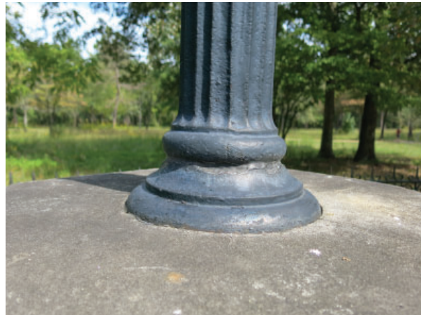
Figure 71: Detail of cast iron column and base with later patch between them, 25 September 2017.
