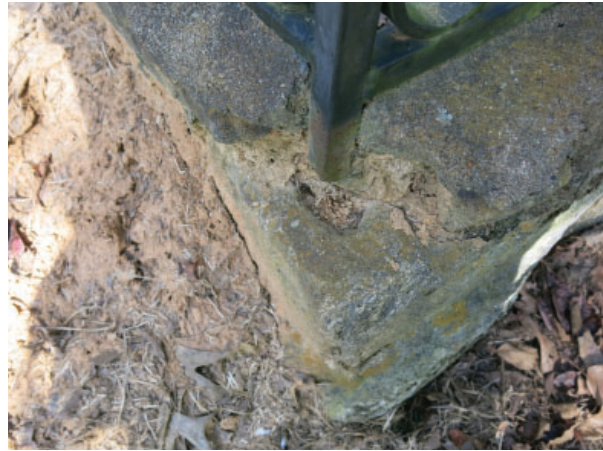
Figure 79: Detail of spalled mortar and former embedment hole in stone wall, 25 September 2017.
