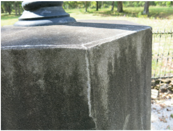
Figure 69: Detail of top of pedestal showing cracks in 1993 stucco, 25 September 2017.
