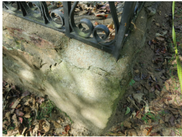
Figure 78: Detail of typical condition with mortar at connection between wall and iron fence, 25 September 2017.
