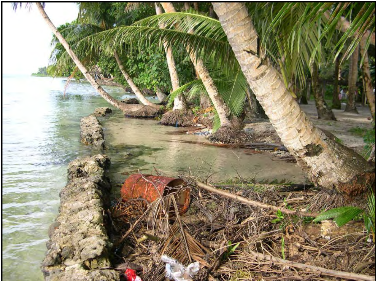
Fig 23: High tide breaches the seawall on Satawan
