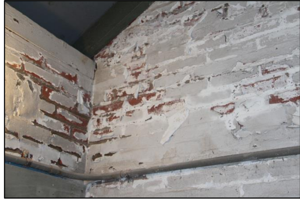
Figure 85. The paint on the interior of the walls is peeling and degraded. Note the presence of Portland cement-based mortar (not original). Photo: HPTC, 05/12/16.
