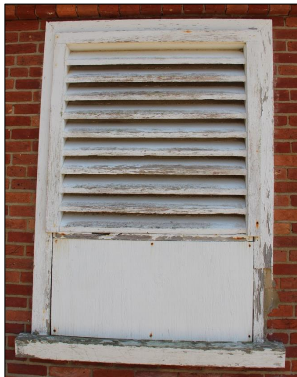
Figure 86, right. An example of one of the deteriorating and non-character-defining window openings. Photo: HPTC, 05/12/16.
