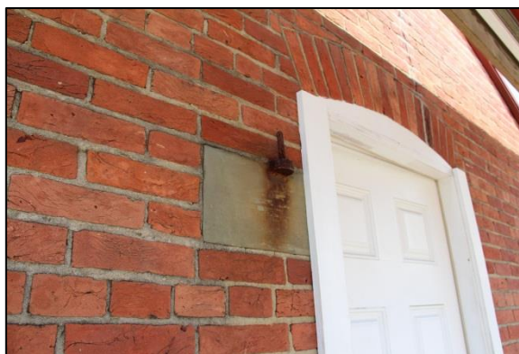
Figure 77. A pair of slate blocks with metal pintles have been retained at the door opening, however the original metal door has been replaced with one that does not match the original in any way. Photo: HPTC, 05/12/16.
