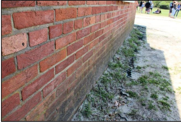
Figure 84. Biological growth present at the base of the exterior wall due to splashback from water draining from the roof. Note the presence of Portland cement-based mortar (not original). Photo: HPTC, 05/12/16.
