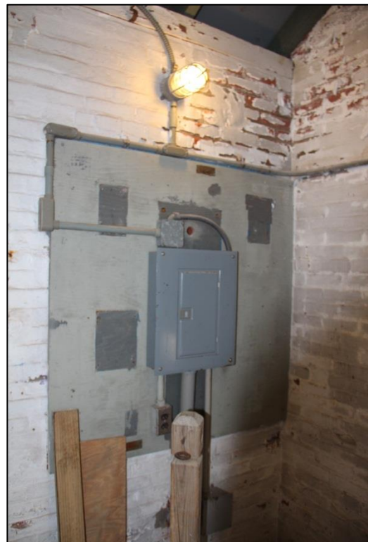
Figure 72, right. The modern 200-amp electrical panel and a light. Photo: HPTC, 05/12/16.
