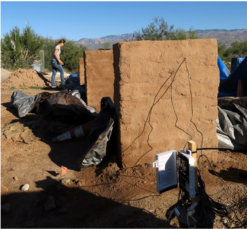
Each wall was fitted with two moisture sensors built into bricks.
