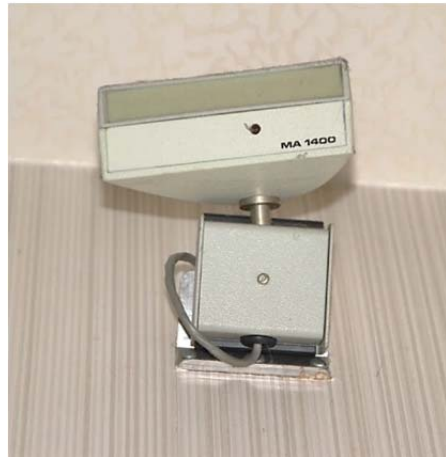
FIGURE 216. Security device likely obsolete.
