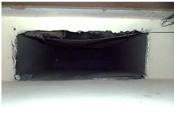
FIGURE 165. Return air opening in closet of Martin Jr. and A.D.'s room. Grille was removed when duct was cleaned.
