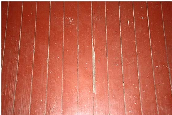
FIGURE 203. Typical wear on wood flooring.
