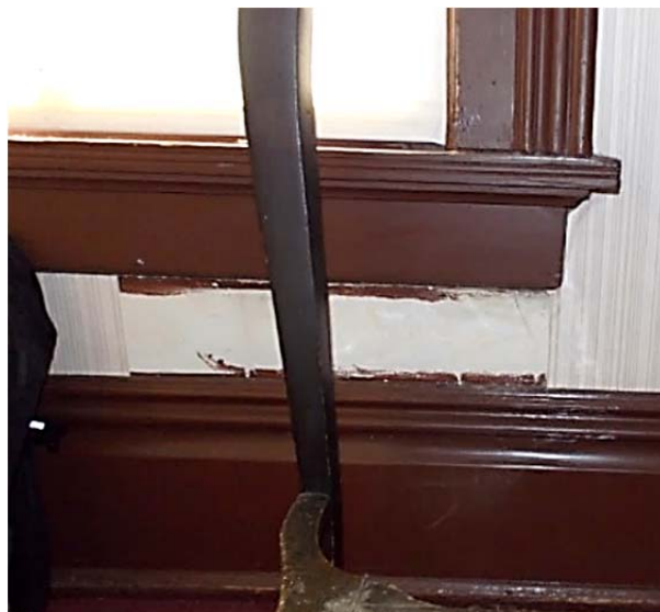
FIGURE 160. Deterioration of plaster below window.
