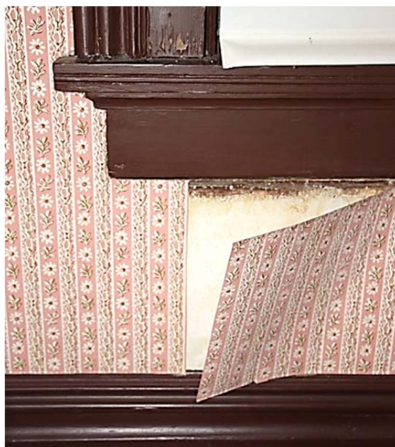
FIGURE 161. Delamination of wallpaper below window.
