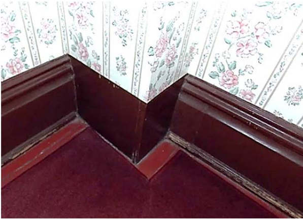
FIGURE 206. Non-original furred enclosure in the dining room, bottom painted brown to match trim but with no actual wood trim.
