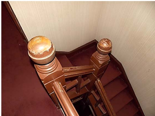
FIGURE 198. Worn finish on newel posts.
