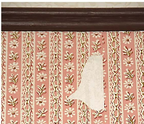
FIGURE 159. Wallpaper damage at Christine's room.
