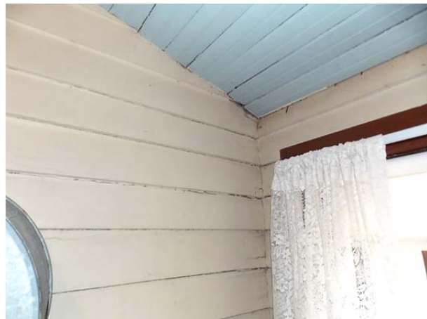
FIGURE 201. Deteriorated wood siding inside the back porch.
