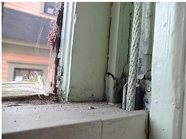
FIGURE 174. Damaged parting strip above lower window sash.
