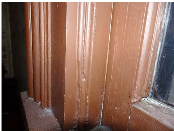
FIGURE 183. Jamb with bead molding at first-floor window. Note damage including chips and divots at bead molding.
