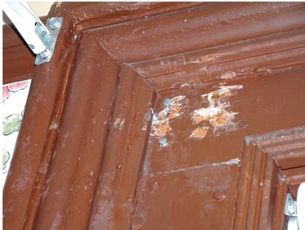
FIGURE 182. Wood casing where a curtain rod had been previously removed.
