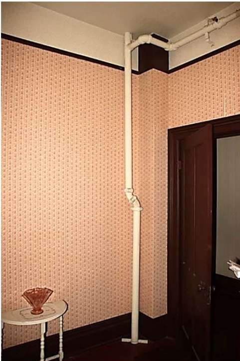
FIGURE 207. Sprinkler riser at Christine's bedroom. Furred enclosure painted brown above picture rail and at the bottom.
