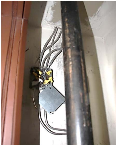
FIGURE 214. Open junction box in a closet.
