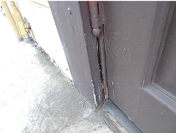
FIGURE 186. Open joint between the door casing and door jamb.
