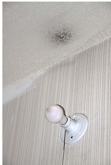
FIGURE 212. Discolored wallpaper above wall mounted light fixture at the stair landing.
