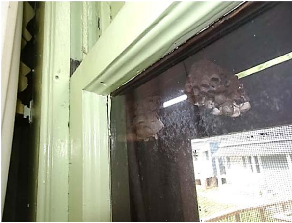
FIGURE 177. Mud dauber nests between the window sash and screen.
