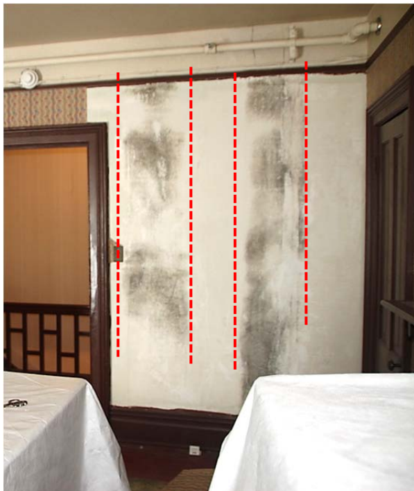
FIGURE 163. Mold and mildew following paths of two in-wall HVAC ducts in the birth room.
