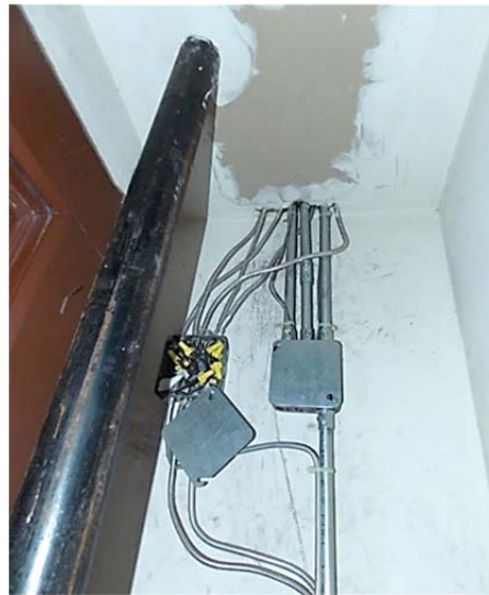
FIGURE 215. Open junction box and conduit penetrations at closet.
