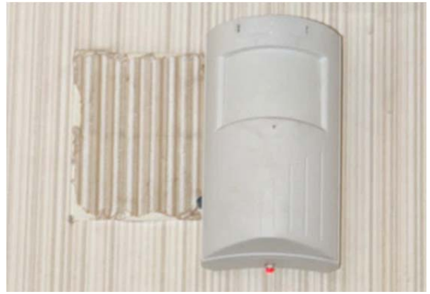
FIGURE 56. Exposure of previous wallpaper at wall mounted device in hall.
