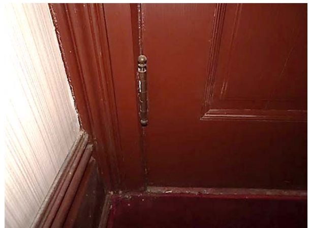
FIGURE 88. Hinge at side entrance door.
