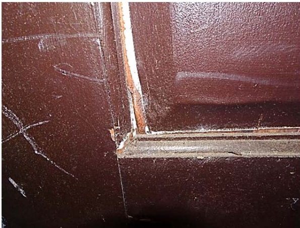
FIGURE 185. Displacement of recessed wood panel on the first-floor rear door.
