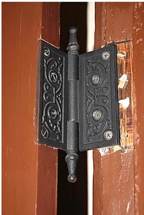
FIGURE 191. Displaced door hinge. Note the white wood filler in the screw holes of the original hinge.
