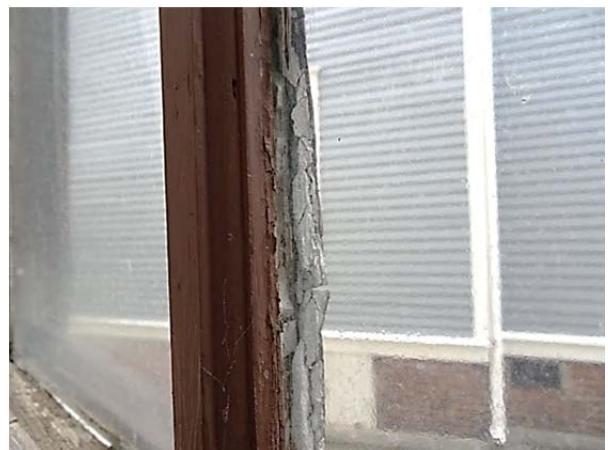
FIGURE 172. Exterior glazing putty that is cracking and deteriorating. The paint coating appeared to be keeping the putty in place.
