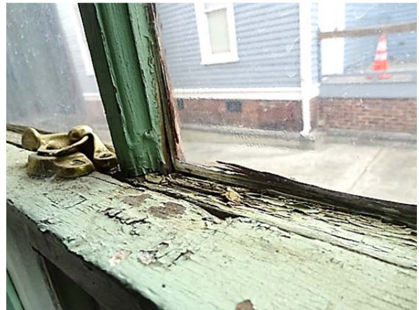
FIGURE 171. The sash where the wood stop and exterior glazing putty were missing.
