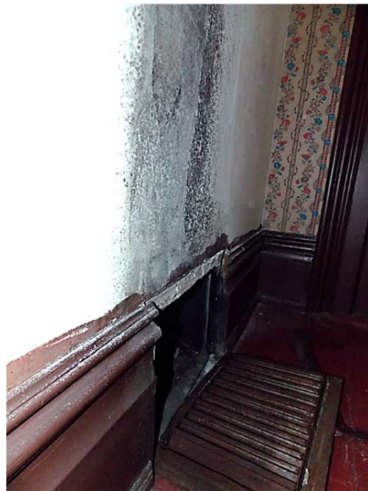
FIGURE 164. Mold / mildew following paths of two in-wall ducts at birth room.
