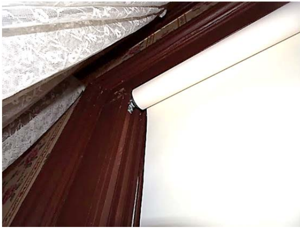
FIGURE 65. Typical roller shade at window opening.
