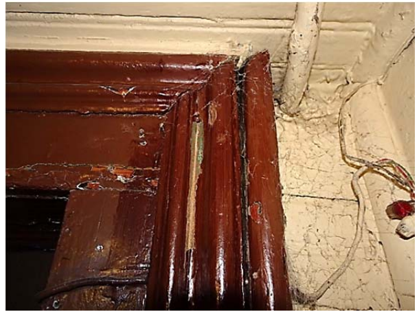
FIGURE 187. Displaced trim at second-floor exterior door.
