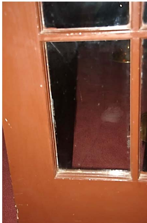
FIGURE 192. Cracked glass light at French door.
