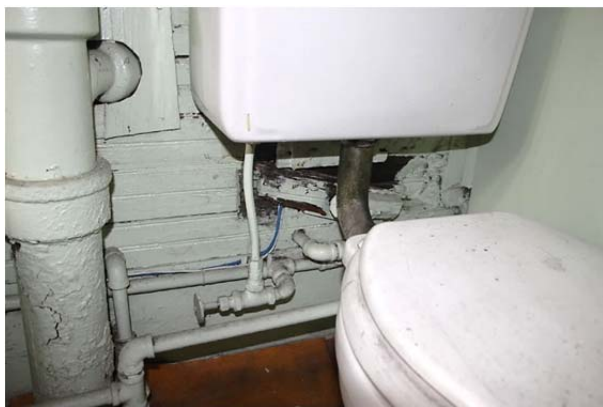
FIGURE 199. Damaged wainscot panel behind the toilet.
