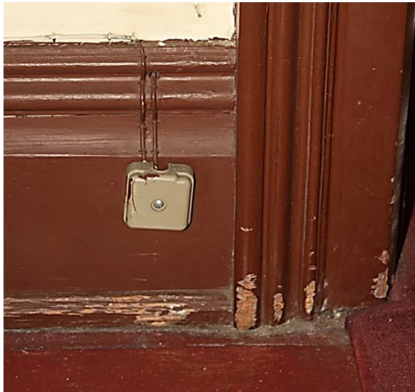
FIGURE 194. General wear at wood casing and base.
