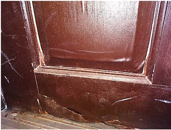
FIGURE 184. Severe damage at the bottom of the rear door on the first floor.
