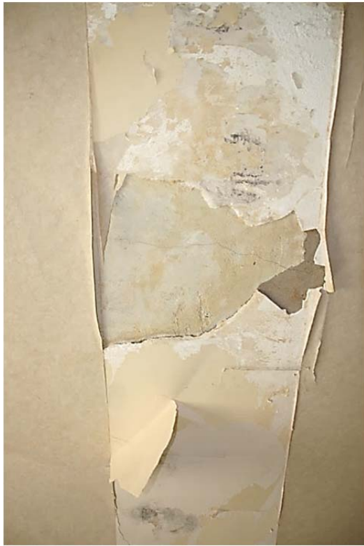
FIGURE 162. Moisture damage to the ceiling paper and plaster ceiling of birth room.
