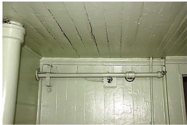
FIGURE 200. Deteriorated ceiling boards in the bathroom.
