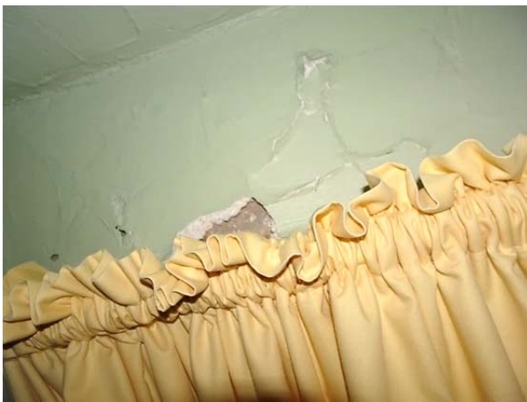
FIGURE 178. Deteriorated plaster and moisture staining above the window unit.
