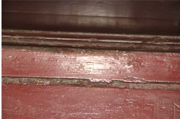
FIGURE 202. Aged separation at wood flooring.
