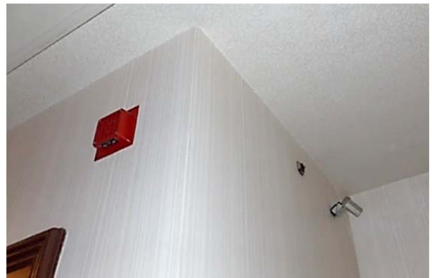
FIGURE 211. Typical installation of alarm and security devices in the second-floor hall.
