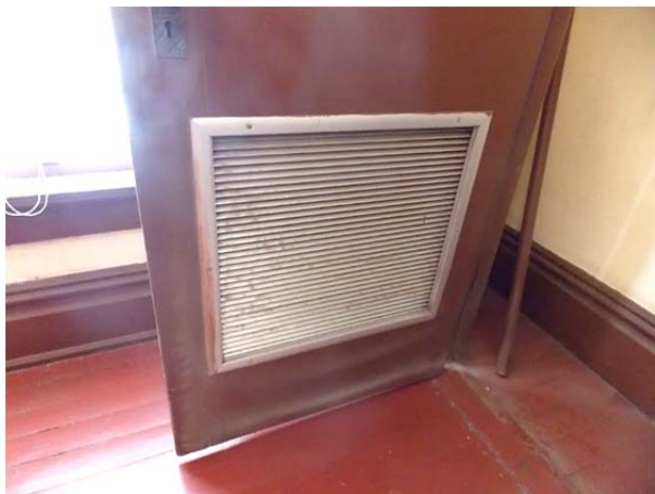
FIGURE 166. Return air grille in the door to of the closet in Martin Jr. and A.D.'s bedroom.
