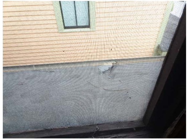
FIGURE 179. Tear in the window screen at west elevation.
