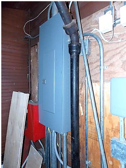
FIGURE 209. Main electrical panel at rear porch pantry.
