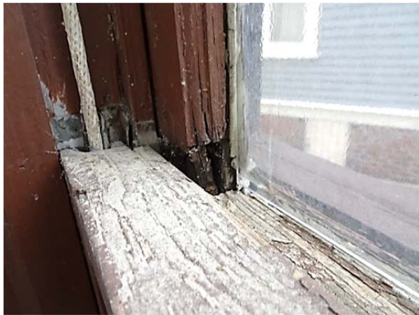
FIGURE 173. Note, the meeting rail of the upper sash has deteriorated and dropped.
