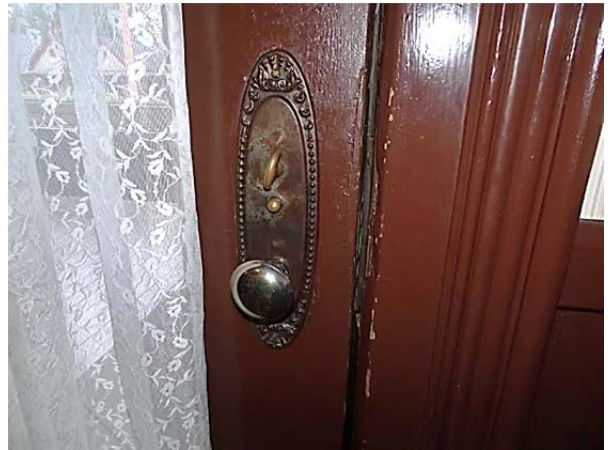
FIGURE 189. Door knob and escutcheon plate on the front door. Note the original finish has been worn away at some places.
