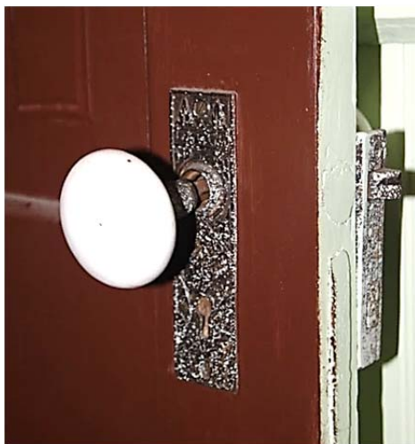
FIGURE 106. Surface-mounted latch set at bathroom.
