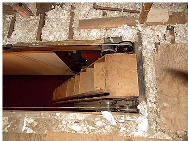
FIGURE 168. Attic access ladder. Previous seal over the access door has deteriorated.
