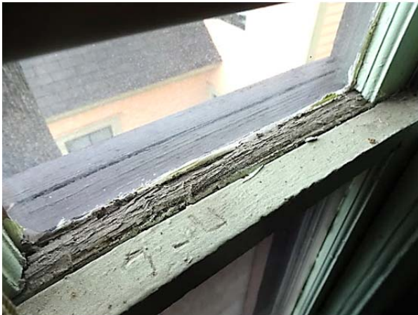
FIGURE 169. Top surface of meeting rails between sash. Note that the upper sash rail has degraded paint and extensive weathering of the wood.
