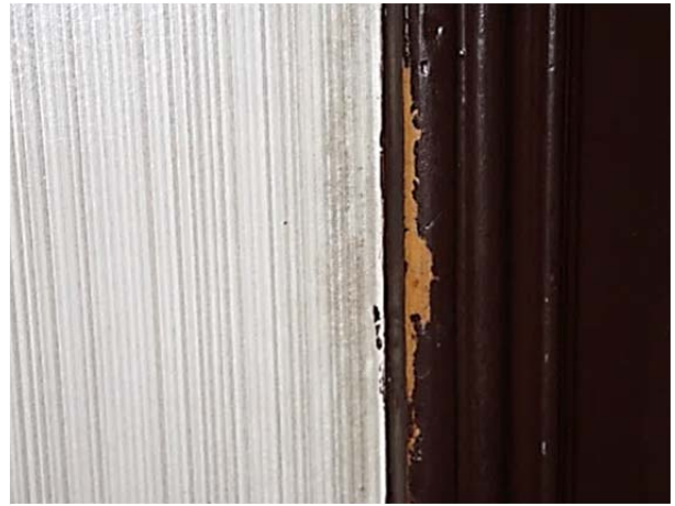
FIGURE 195. General wear at a door casing.
