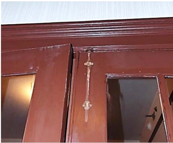
FIGURE 97. Flush bolt at French door.
