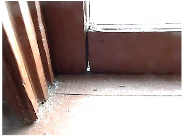
FIGURE 170. A second-floor window sash on the north elevation with an open joint. Note daylight visible at the joint.
