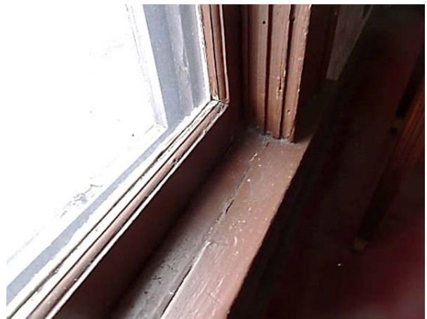
FIGURE 180. Previous dutchman repair to this window stool has open joint.
