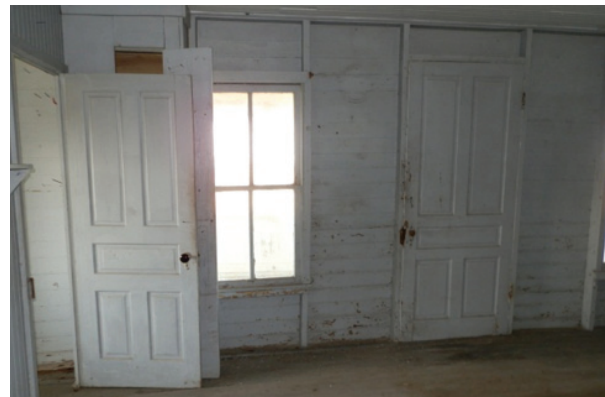
Figure 9. View of framing at north side of Room 101 in the original building. Note the lack of proper headers at the openings.
