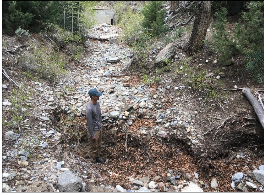
Figure 11.4. Researcher standing in a sinkhole below the Snake Creek pipeline inlet structure, part of which is visible in the background.
