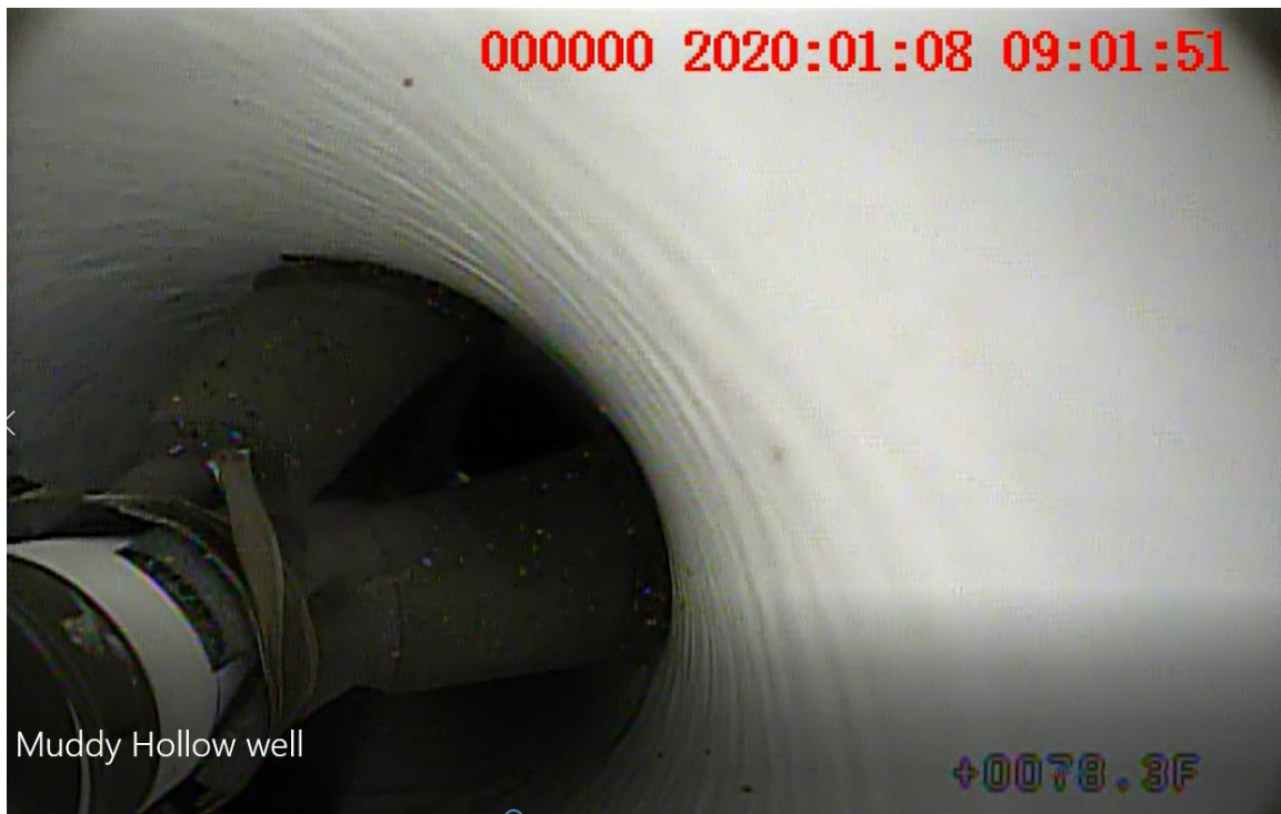
Casing centralizer on upper section of the production pump.
