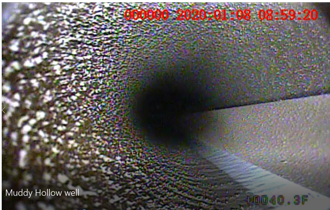
Minor mineral encrustation on well casing. Drop pipe rubbing along one side of the casing, indicating the borehole is not plumb through this section.
