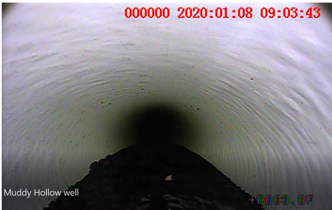
Base of pump motor showing accumulation of black material, likely iron and manganese.
