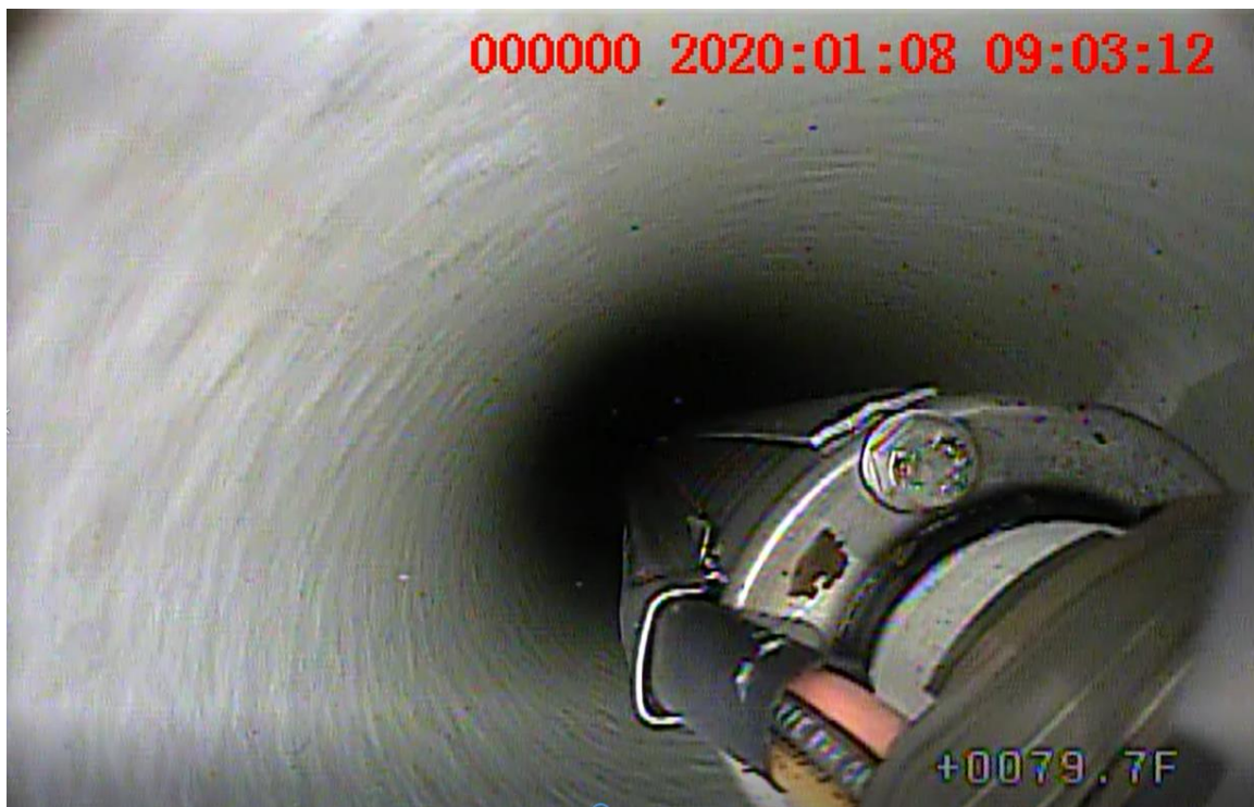
Top of pump immediately below casing centralizer, sitting in a section of blank casing between the upper and lower screened intervals.
