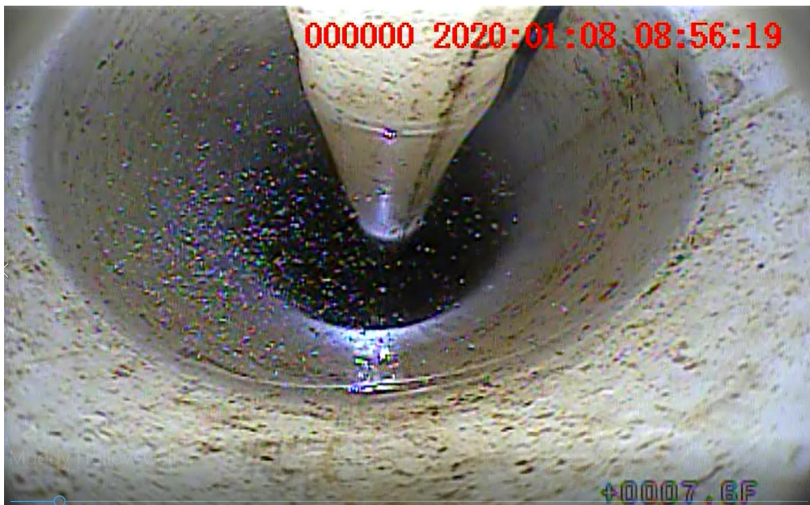
Depth to water at approximately 8 ft. 2-inch PVC drop pipe is supporting production pump.
