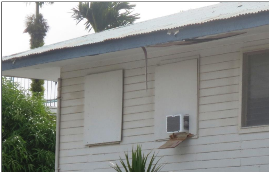
Figure 44. Sablan House, detail of boarded windows on east elevation.
