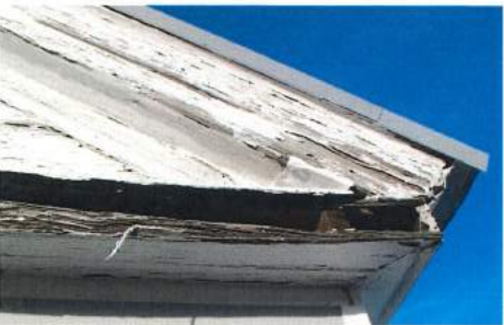
Photo 3- South Gable deterioration
