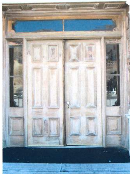
Photo 12 - Existing 3rd Floor Porch Door Showing the Threshold
