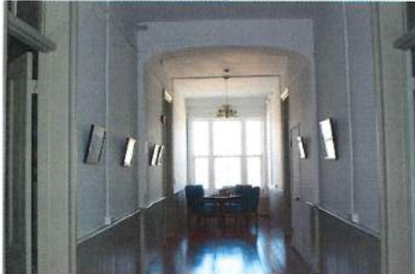
Photo 24 - 2nd Floor Hallway showing masonry transverse wall arched
