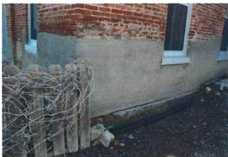
Photo 21 - Northwest Exterior Corner of building showing brick foundation and cement plaster applied to the surface of the brick which is counterproductive as it seals in the moisture.
