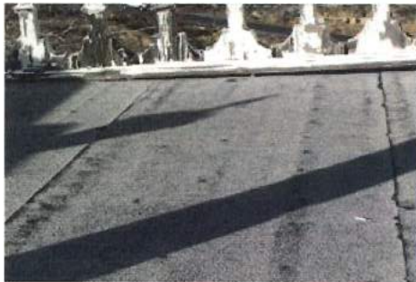
Photo 4 - Existing 3rd Floor Porch Finish
