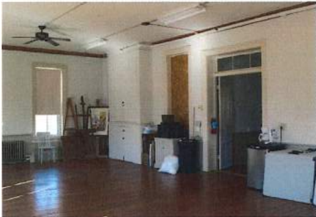
Photo 30 - 3rd Floor Studio space with plaster ceiling and surface-mounted fixtures
