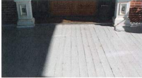
Photo 13 - Second Floor Porch Floor Boards
