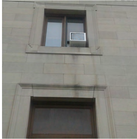
P26: Limestone staining from window a.c. unit, typ.
