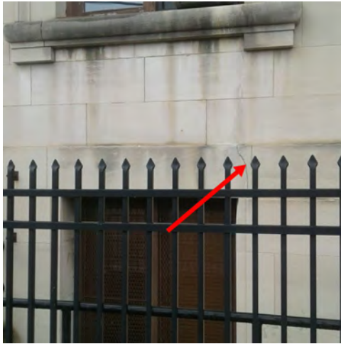
P61: Cracked limestone on E elevation.
