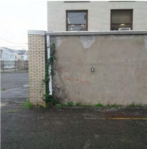
P52: Stucco damage at garage addition located at the S elevation.
