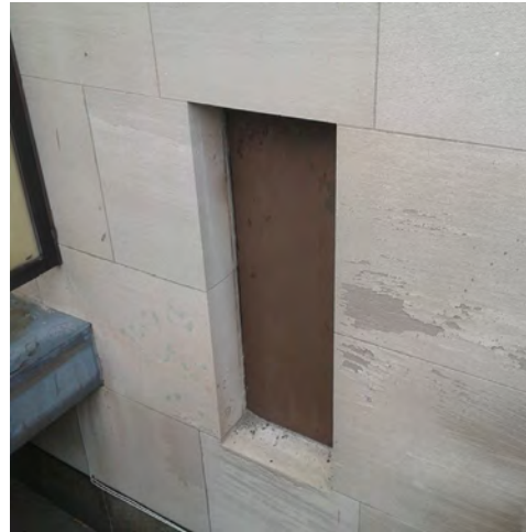
P68: Window boarded
