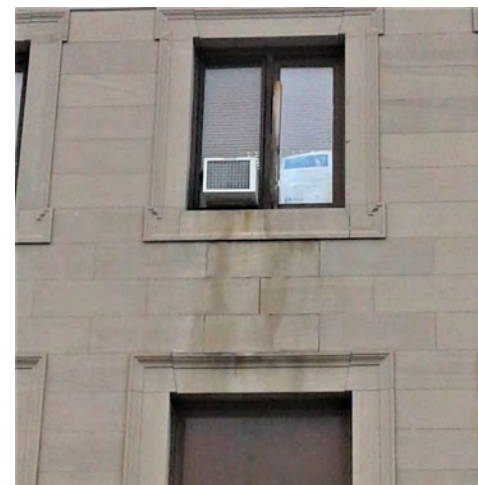
P147: Staining from a.c. window unit.
