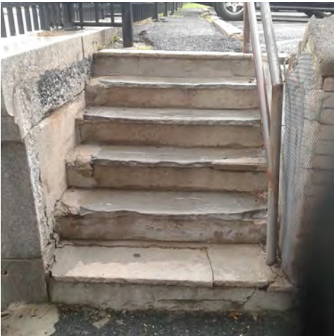
P82: Damaged steps and retaining wall from E. elevation to parking.
