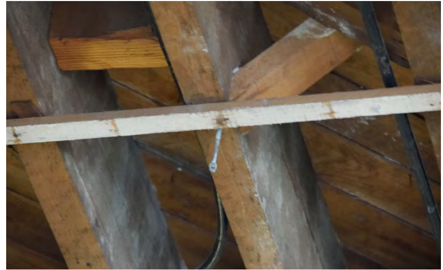
Photograph #2 – One of the Few Drop Ceiling Anchors Installed in a Floor Joist
