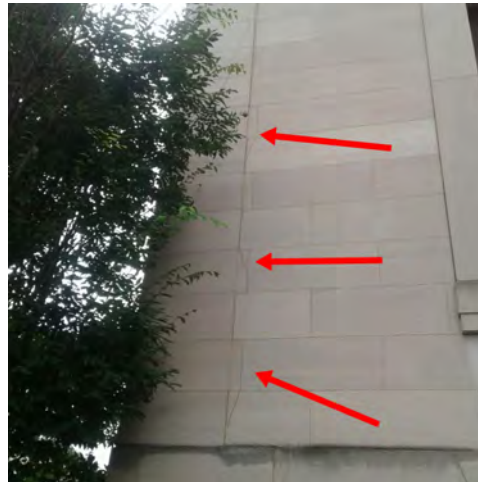
P 137: Cracked limestone
