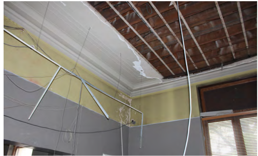
Photo 38: The suspended ceiling was hung from the plaster rather than the floor joists. After 40 years, the weight of it caused the ceiling to fall
