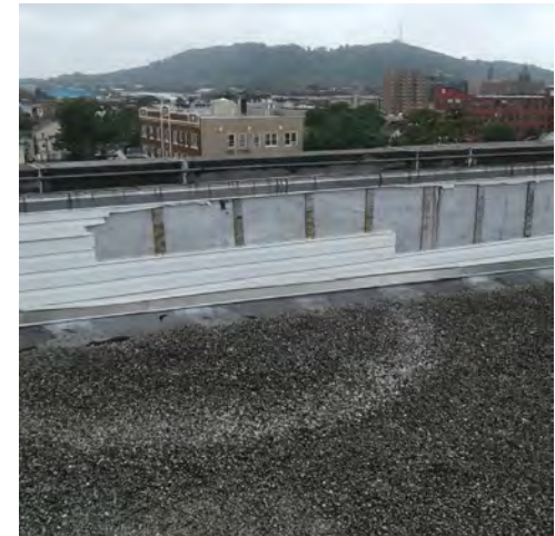
Pro8: Damaged material protecting the roof parapet, typical.
