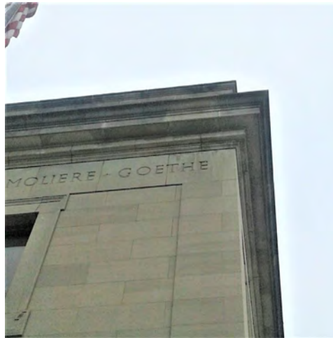
P29: Staining and saturation at cornice, typical.
