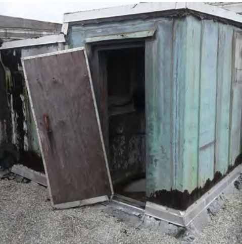
P100: Roof access door is damaged and off its hinges. Note the tar on the copper, causing corrosion.
