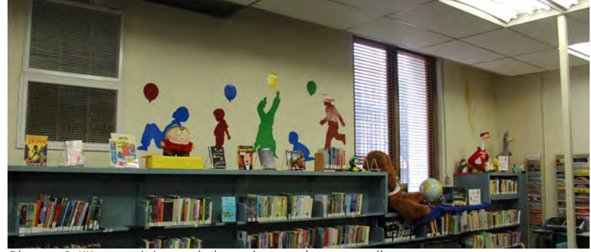
Photo 118: Water staining and plaster loss on the west wall
