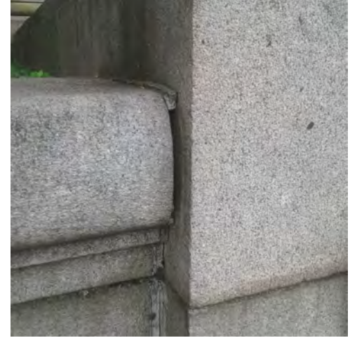
P12: Missing mortar adjacent to main entry stairs
