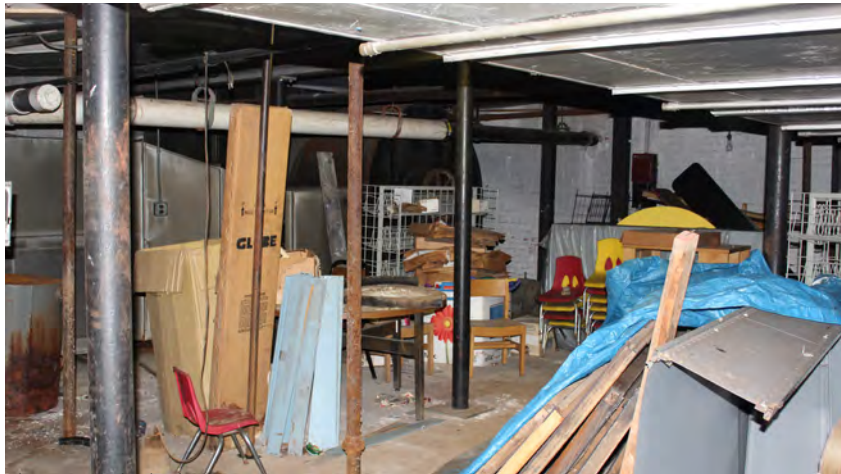
Photo 119: The boiler room
