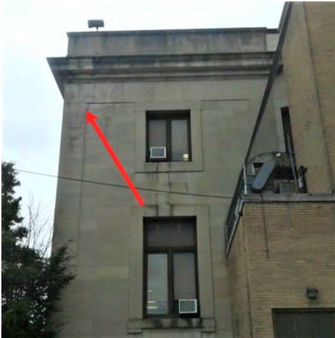
P133: Evidence of water infiltration, S elevation near E corner.
