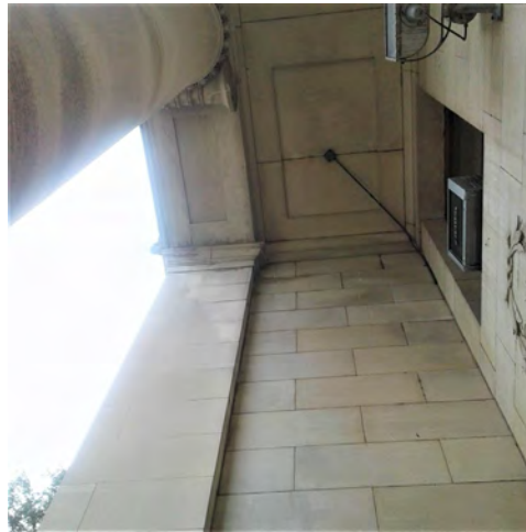
P41: Water intrusion saturation at top of portico.
