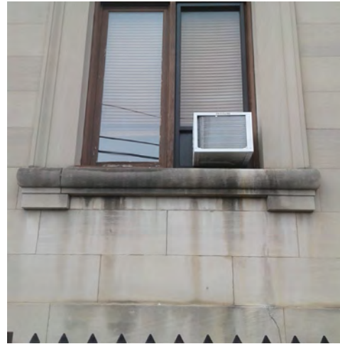
P62: Staining at window sill, typical. (E. elevation)
