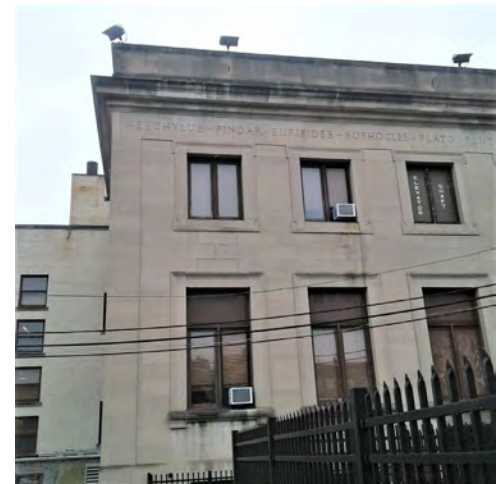
P78: Staining from a.c. window unit, typ. E. elevation.
