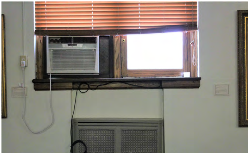
Photo 72: Most of the windows need reglazing
