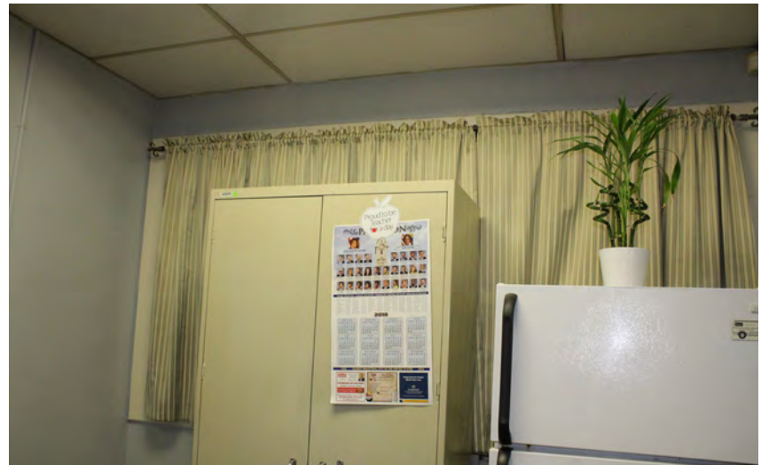
Photo 90: The internal business window is no longer used and should be removed in the long term
