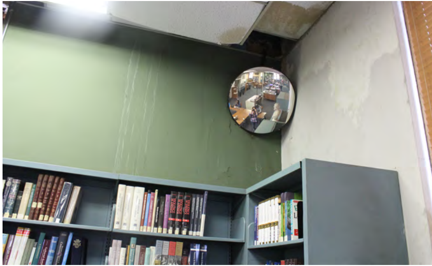
Photo 65: Water damage in the SW corner
