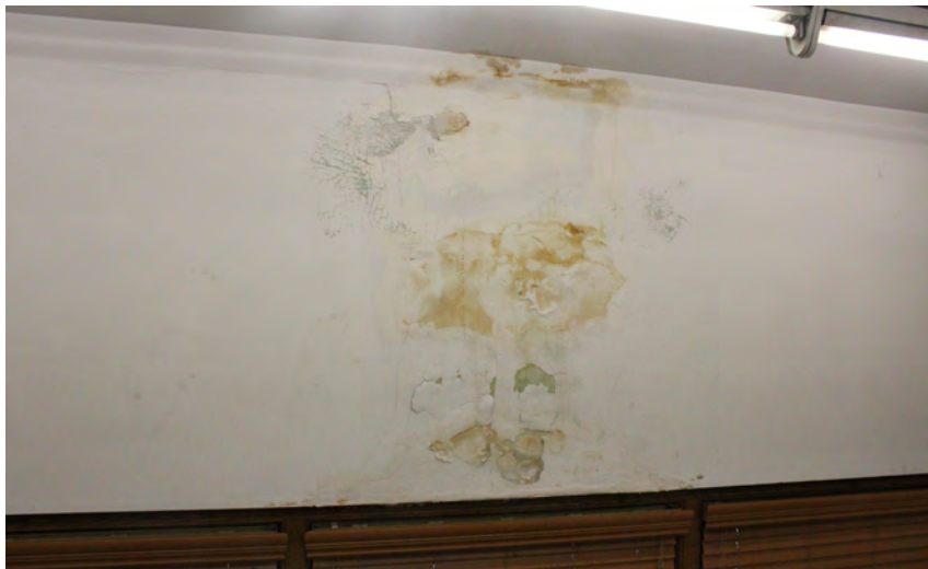
Photo 67: Water damage visible from the mezzanine on the south wall
