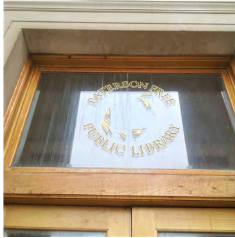
P38: Water damage at wood front entry doors.
