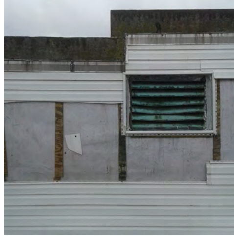
P110: Typical damage to material at the parapet.
