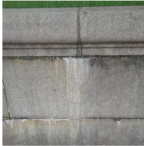
P8: Efflorescence/water infiltration at granite retaining wall, N elevation
