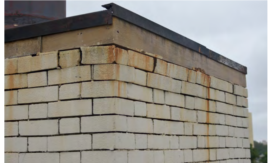
Photograph #8 – Loose Bricks and Limestone Coping
