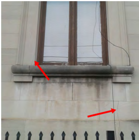
P64: Cracked limestone at first floor window at E elevation.
