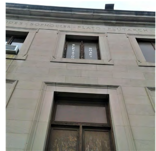
P66: Windows boarded at elevator, E elevation.
