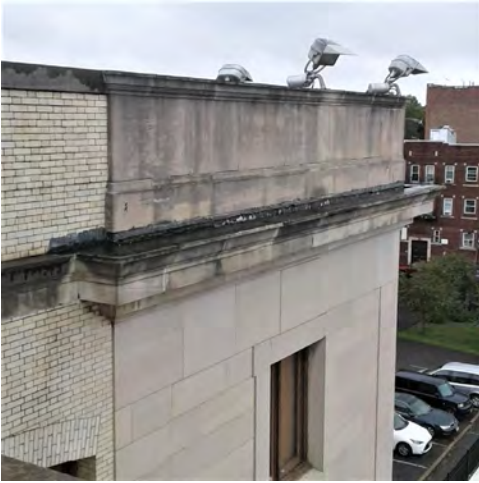
P97: Severe staining at cornice, rear (S) elevation, E corner.
