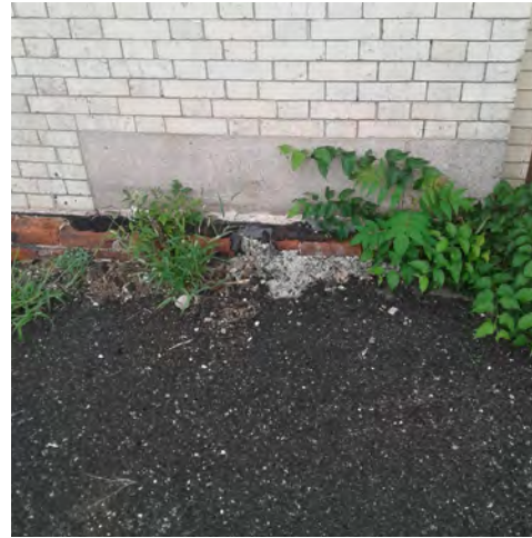
P92: Damaged brick at the base of the rear wing, SE corner.
