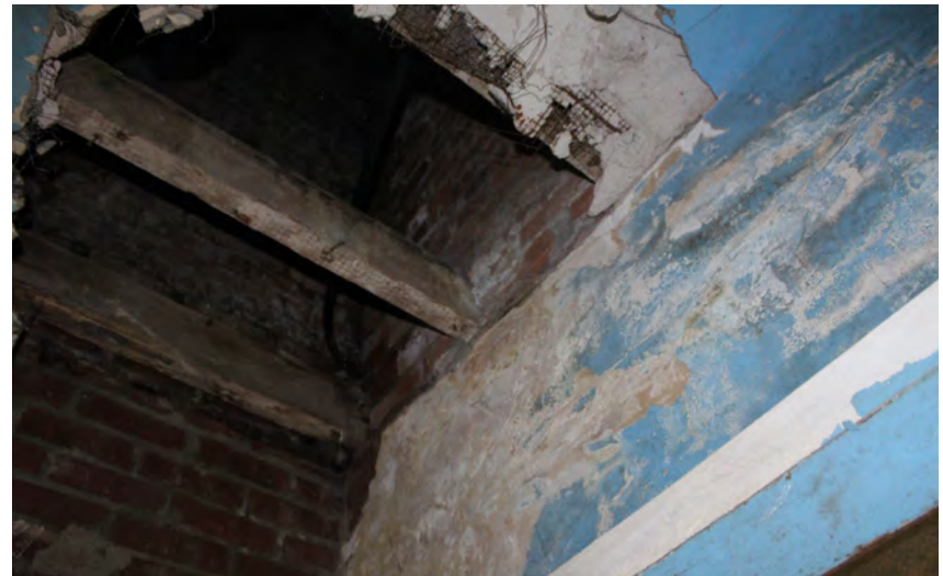
Photo 81: A leak caused damage, loss of plaster and heavy mold
