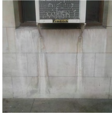
P32: Staining from a.c. window unit to right of main entry.
