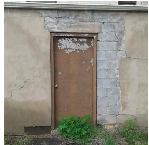
P54: Concrete spalling at garage addition.
