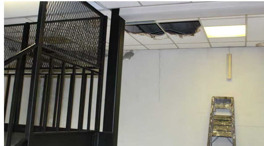
Photo 128: The tower is in poor condition with significant water damage
