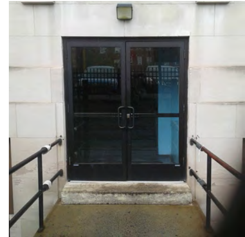
P69: Location of entry to stairs at E elevation. Stone is stained and concrete damaged.
