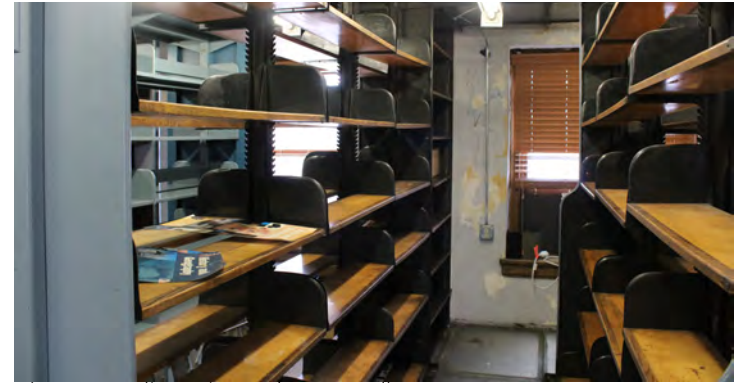
Photo 54: Peeling paint on the west wall
