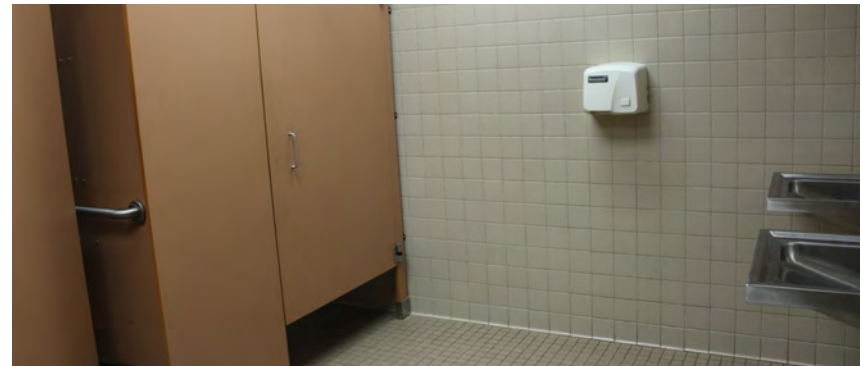
Photo 100: The women's room only has two toilets and two sinks
