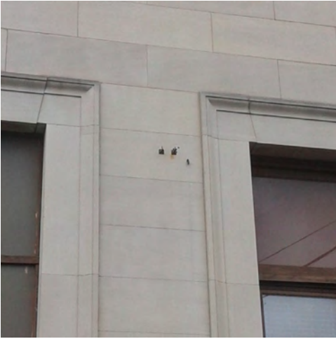
P79: Utility anchors abandoned in place, E. elevation.
