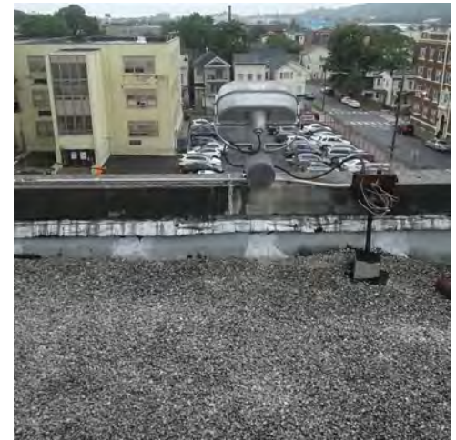
P102: Lighting attached to roof parapet.
