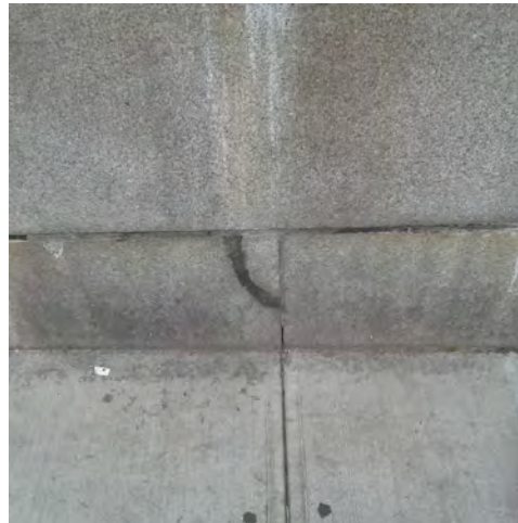
P11: Previous repair of cracked stone
