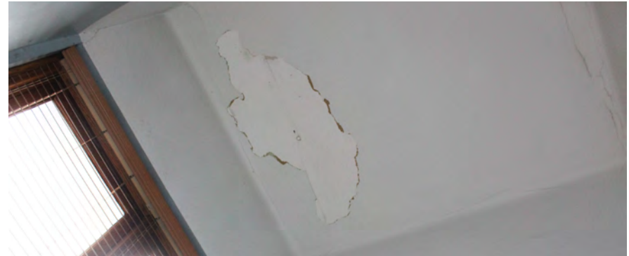
Photo 86: Water damage in the bathroom ceiling
