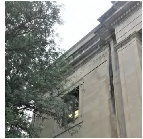
P51: Corrosion from previous repair copper straps, left side of N elevation.
