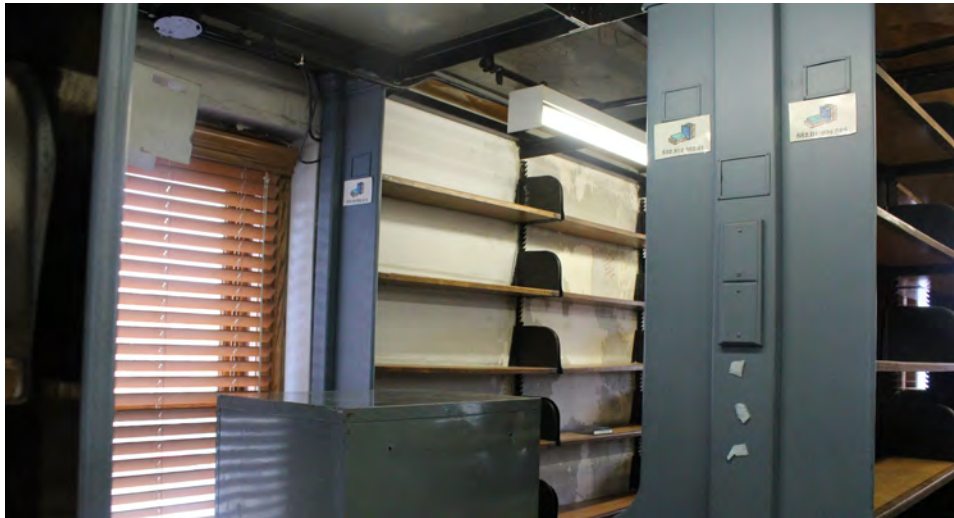
Photo 55: There is also water damage on the east wall
