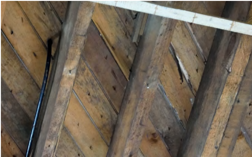
Photograph #3 – Furring Fasteners Pulled Out/Furring Pulled Over Fasteners
