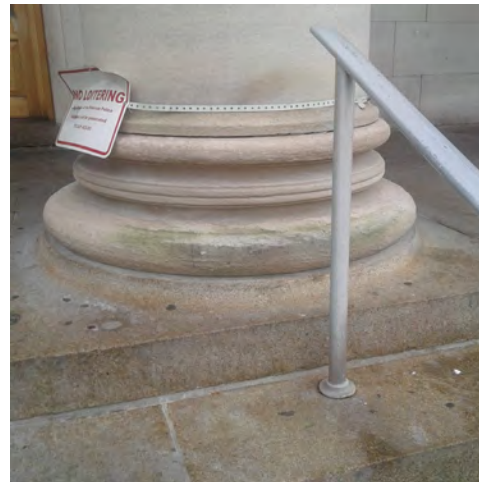
P35: Biological growth at limestone column base.
