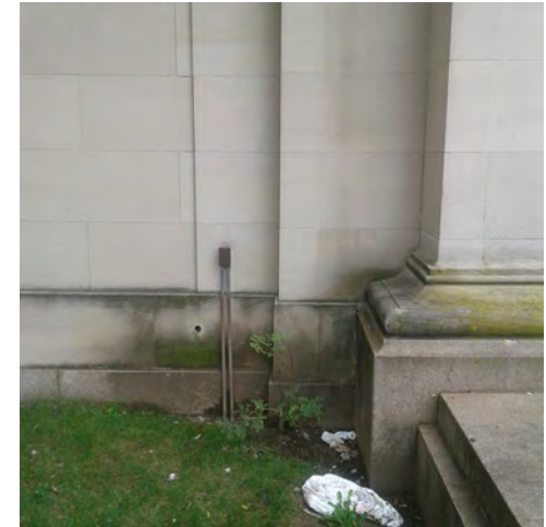
P45: Staining at base to left of main entry.
