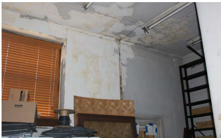
Photo 123: Additional water staining
