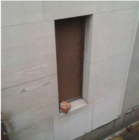
P67: Window boarded near elevator entry, E elevation.
