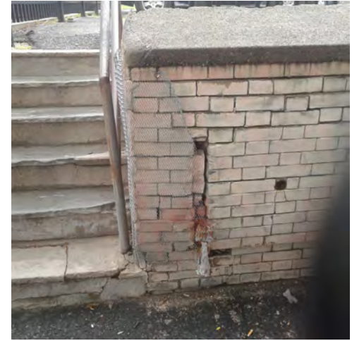
P81: Damaged steps and retaining wall from E. elevation to parking.
