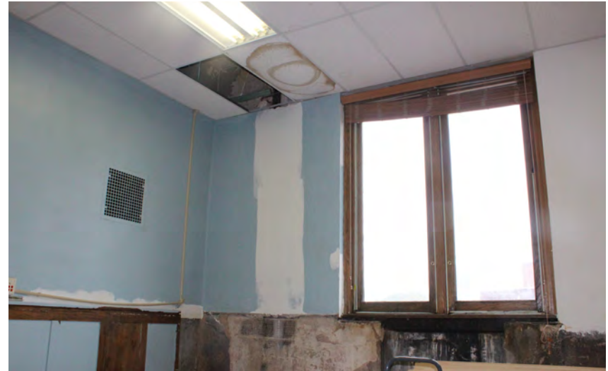
Photo 79: The wainscot is missing on the east wall
