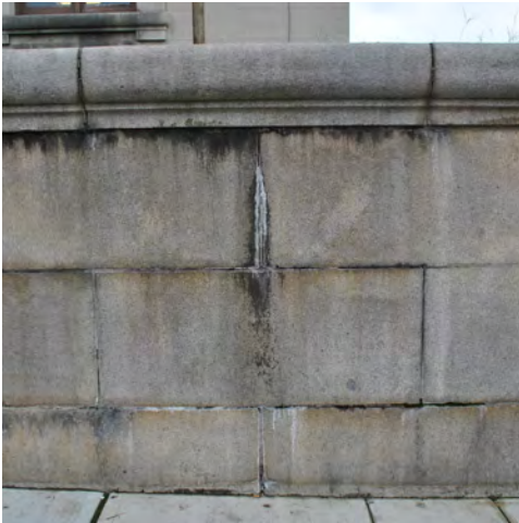
P1: Open mortar joints, mold and efflorescence typical at granite retaining walls.
