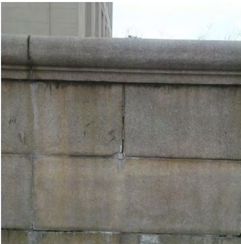
P16: Missing Mortar
