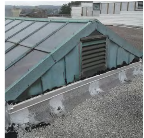
P126: Dissimilar metals at the new roof flashing and the historic skylight.
