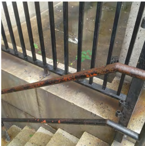
P154: Heavy staining at granite retraining walls.
