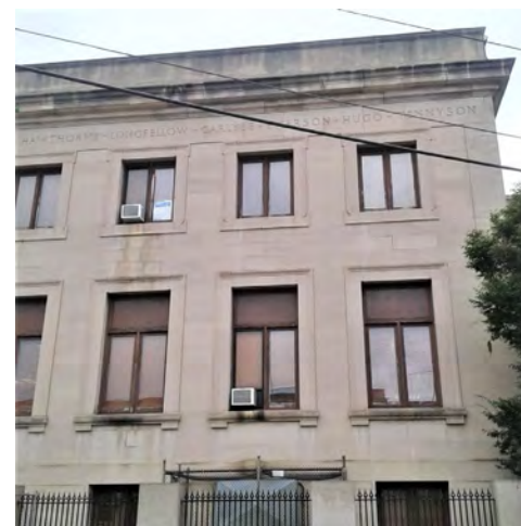
P144: General view of rear of W elevation. Note partially boarded windows, window units, etc.
