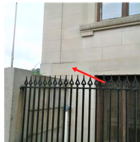
P 150: Cracked limestone at NW corner.
