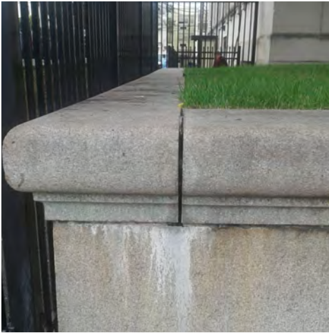
P7: Mortar missing at retaining wall cap, NE corner.
