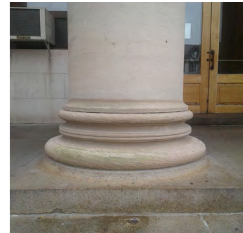
P36: Missing mortar, typical at column bases. Staining at limestone column base.
