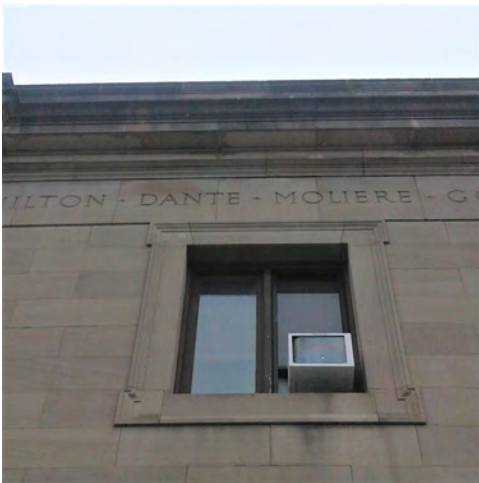
P28: AC unit installed in existing window, damaging the panel, typ. Window frame is damaged, and needs to be repaired and repainted. NE corner of the front elevation.
