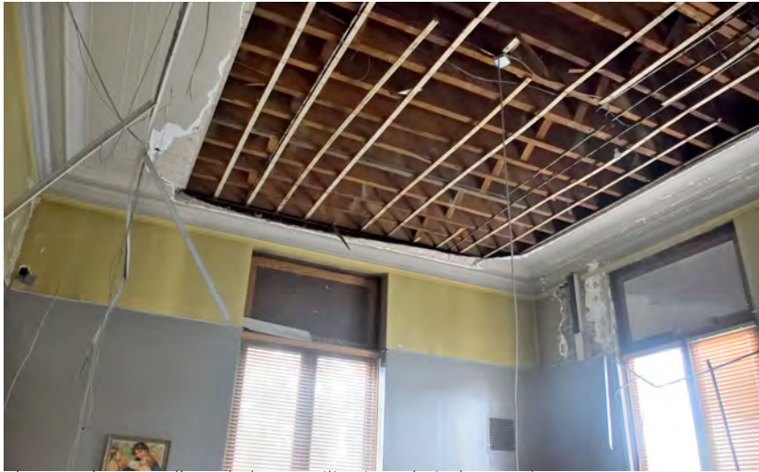
Photograph #1 – Collapsed Plaster Ceiling in Technical Processing Room
