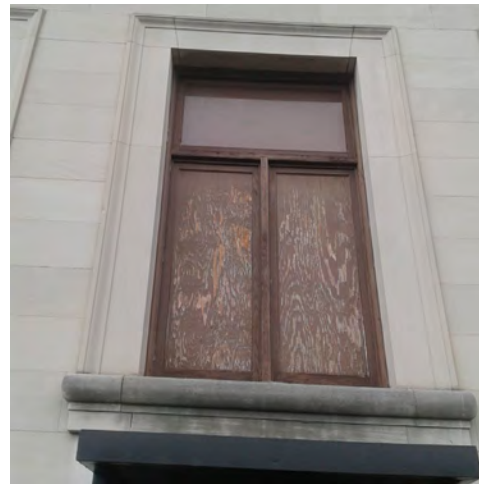
P65: Blocked windows, missing glass at E elevation.
