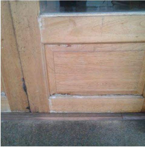
P37: Water damage at wood front entry doors.
