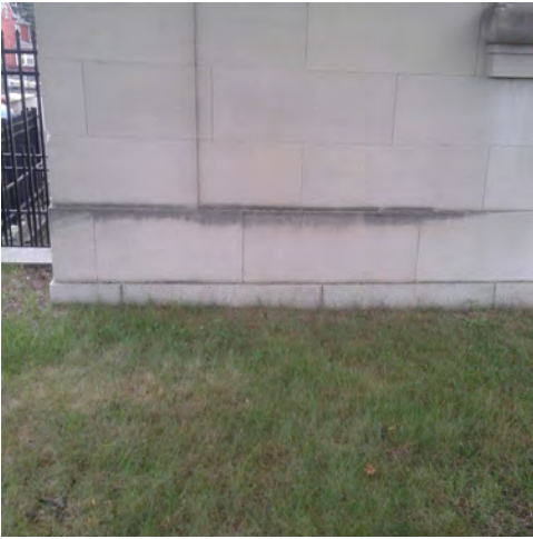
P49: Staining at limestone base, NE corner.
