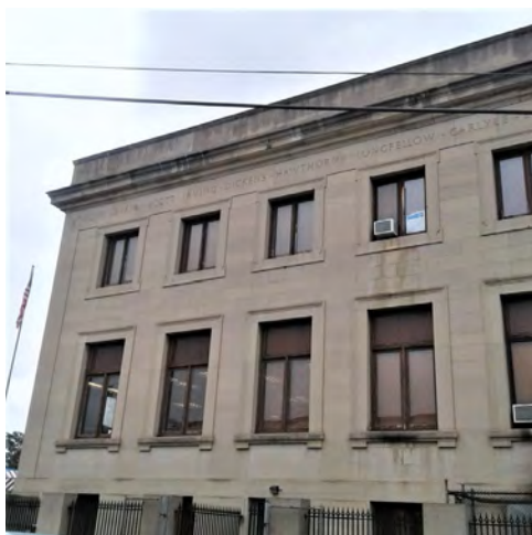
P145: Heavy staining at cornice on the W elevation.
