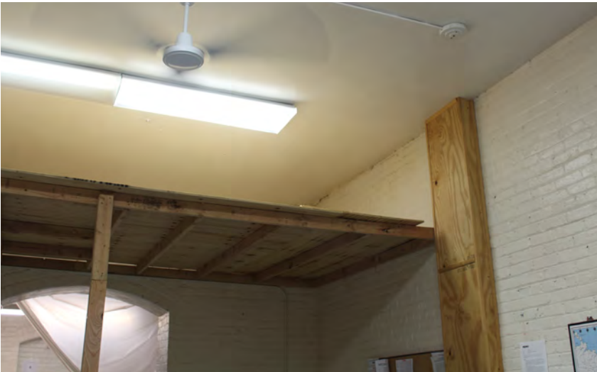
Photo 109: A crack in 007 caused maintenance to build this scaffolding for protection
