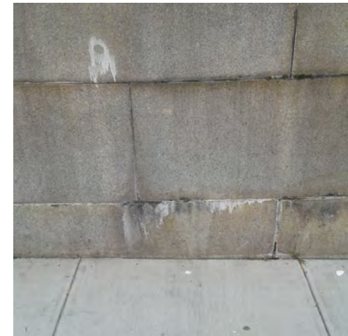
P18: Efflorescence/water infiltration at granite retaining wall.
