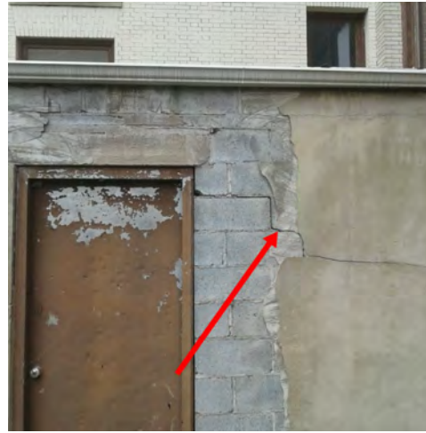
P56: Stepped cracking at cmu on the garage addition.
