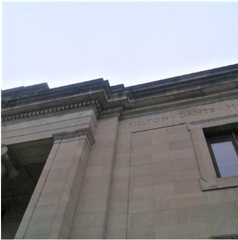
P31: Previously repaired cracked stone at cornice to right of main entry.
