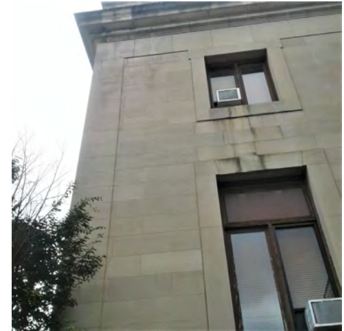
P135: Staining on limestone, blocked windows, and window AC units, S elevation near E corner.
