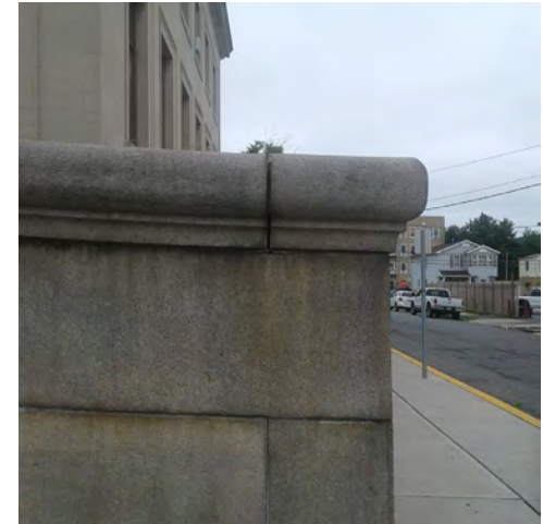
P15: Mortar missing at NE corner of main entry steps
