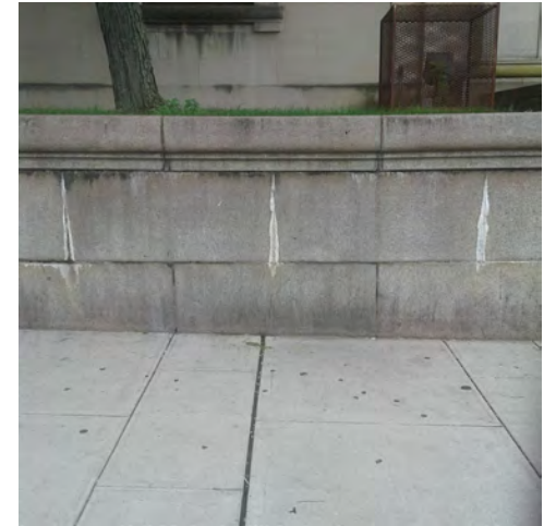
P9: Efflorescence/water infiltration at granite retaining wall, N elevation
