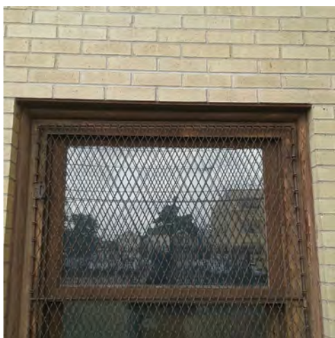
P139: Deterioration of wood windows on the rear addition, typ.
