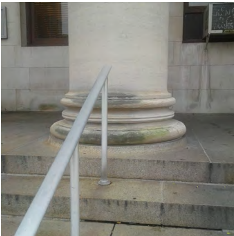
P34: Biological growth at limestone column base.
