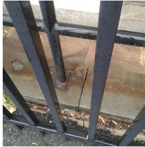
P74: Cracked limestone at fending on the E elevation..
