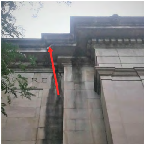
P46: Heavy staining/saturation at cornice extending down to ground level. Broken/Missing stone at cornice.
