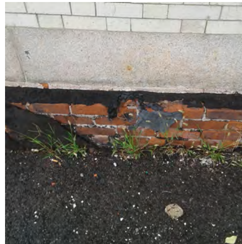
P95: Crumbling brick at foundation of rear wing.
