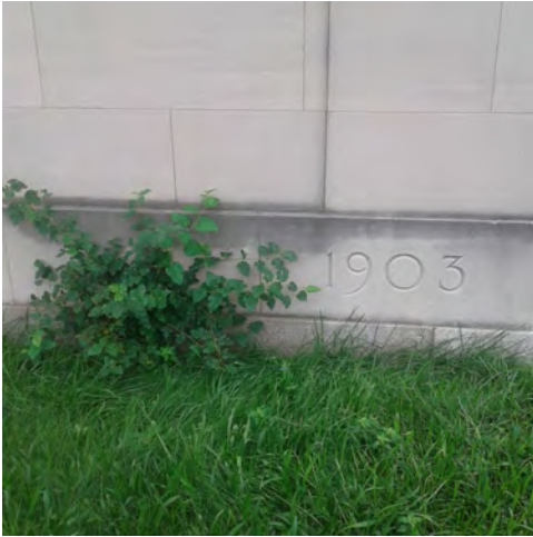
P25: Biological growth at limestone base, NW corner
