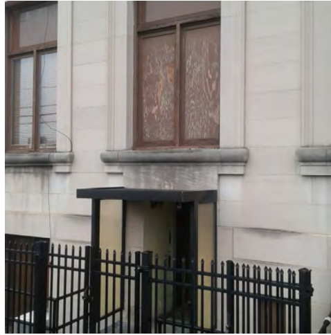
P80: Staining above entry canopy for elevator, E elevation.
