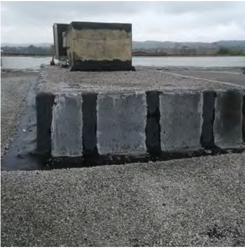
P115: Typical condition at changes in roof elevation, showing repairs at seams.
