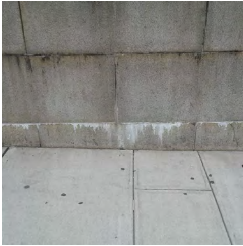
P19: Efflorescence/water infiltration at granite retaining wall, N elevation
