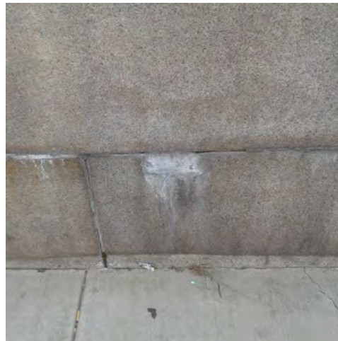
P17: Spalling at base of main entry steps, NW side.
