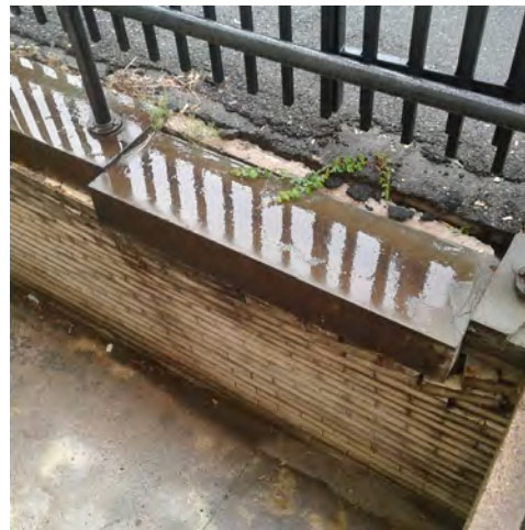
P71: Dislodged and buckling bluestone caps at retaining wall on the E side of the building.
