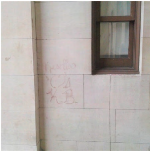
P40: Graffiti on side wall of portico.
