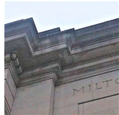
P30: Staining at front cornice, typ.
