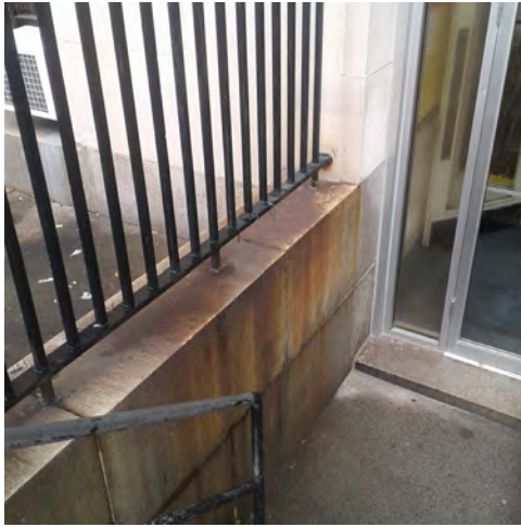
P151: Staining and rust at stairs to Children's Library entry.
