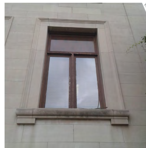
P141: Deterioration of wood windows, typ. W elevation.
