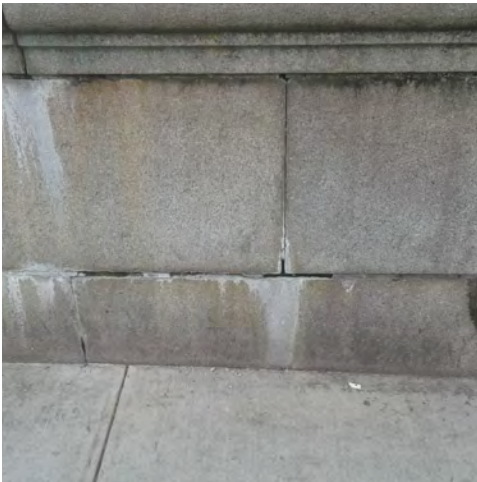
P10: Missing mortar and staining
