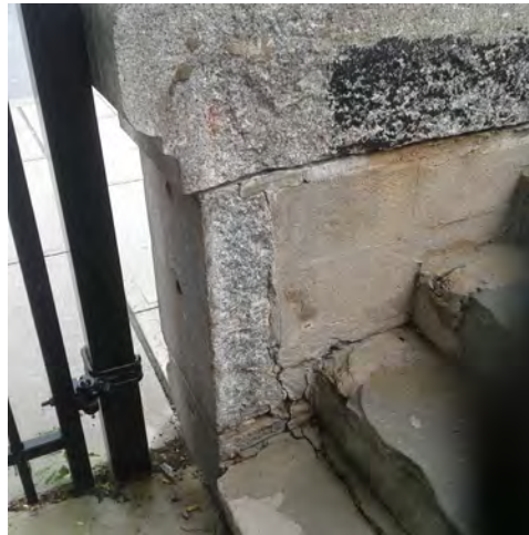
P83: Damaged steps and retaining wall from E. elevation to parking.
