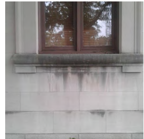
P48: Staining at window sill, first floor to right of main entry. Window needs to be repaired and repainted.
