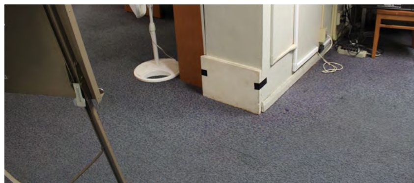
Photo 16: The original marble baseboard is now being held up by tape. This should be remedied immediately.
