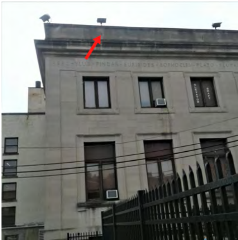
P76: Spalled limestone at cornice at rear of E elevation.
