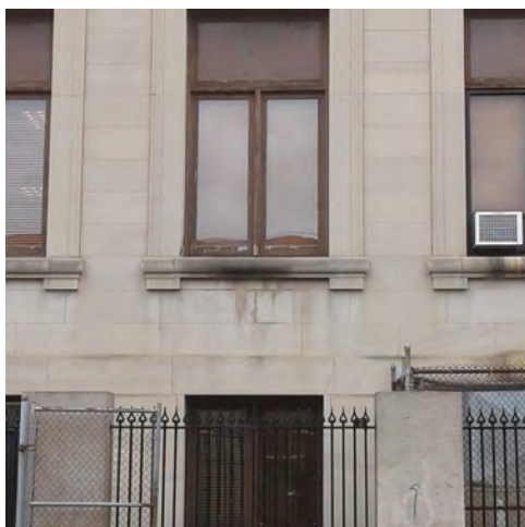
P148: Staining mold at window sill over Children's Library entry on the W elevation.
