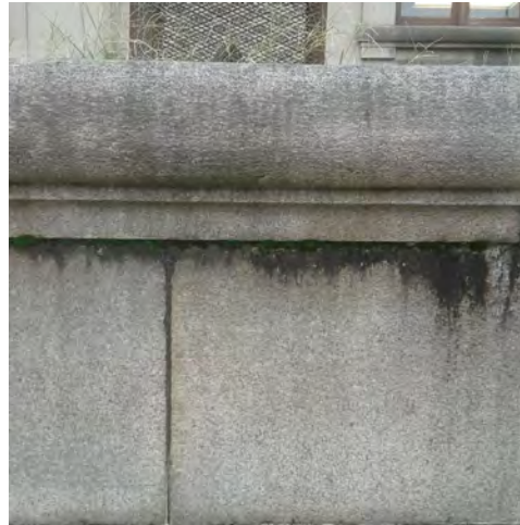
P20: Biological growth and staining under retaining wall cap, N elevation to right of main entry.
