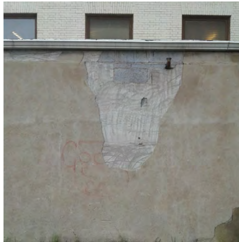
P53: Detail of stucco damage on E elevation of the garage addition.
