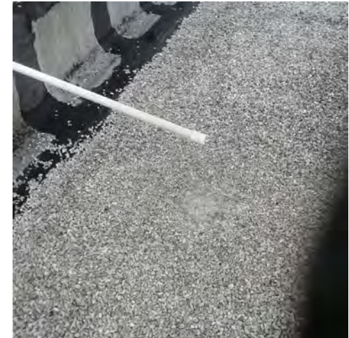
Pro5: Condensate drain from rooftop equipment flowing directly onto roof surface.
