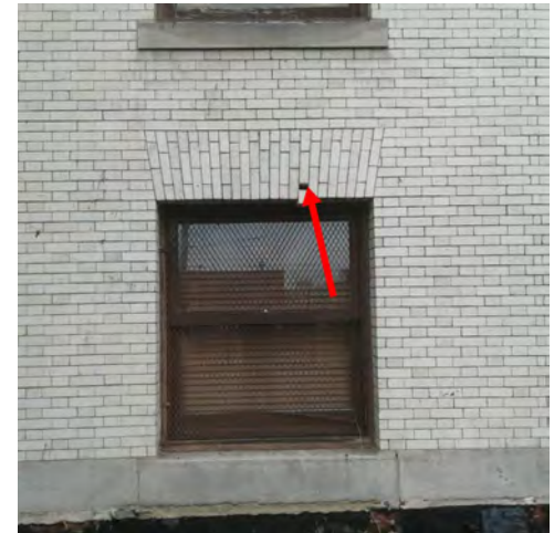
P138: Loose brick at header at E side of rear wing.
