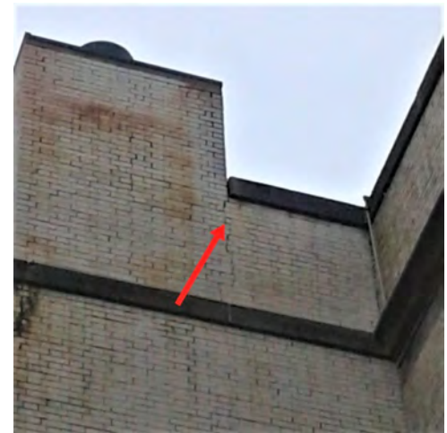
P60: Cracked and stained brick at rear wing.
