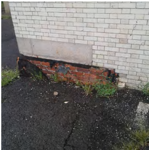
P94: Damage at the base of the rear wing, SW corner.
