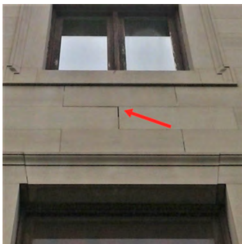
P142: Mortar missing over side entry door on W Elevation.
