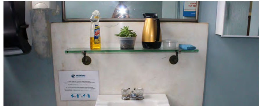
Photo 85: The original backsplash
