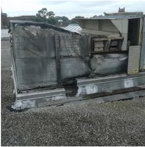
P127: Rooftop equipment.
