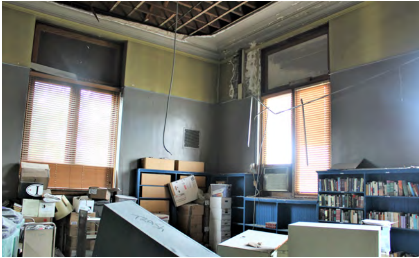
Photo 35: The NE corner of Room 109. The ceiling fell in the spring
