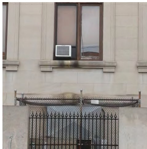
P146: Staining from a.c. window unit, and blocked opening from large HVAC unit at ground floor, W elevation.
