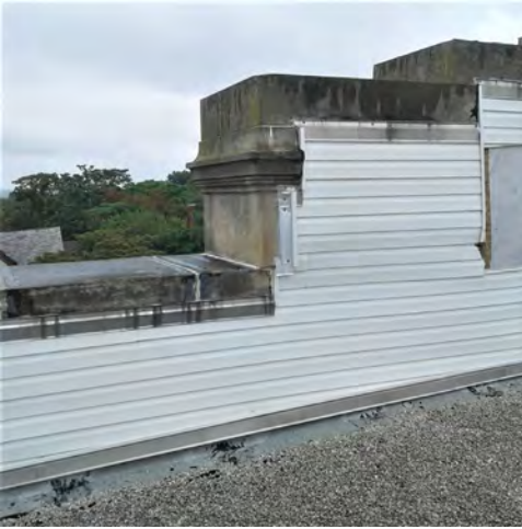
P109: Damaged siding at roof parapet behind main entry.
