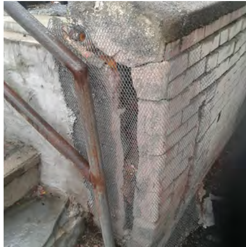
P2: Temporary repair at buckling brick retaining wall.
