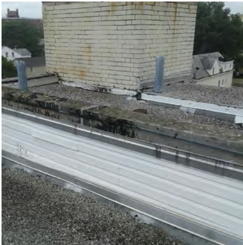
P130: Failing siding at parapet; damaged and stained brick at the exhaust chimney.
