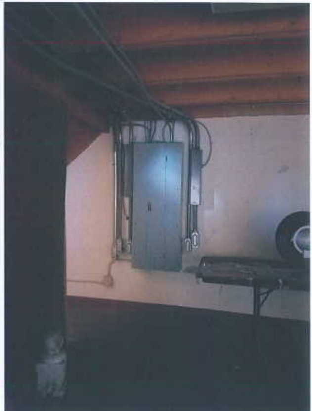
127. Electrical service located at the north end of the freight wing.
