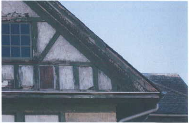
10. Detail, east elevation. Deteriorated stucco and peeling paint.
