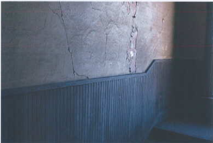
208. Room 205, peeling paint at plaster above historic wood floor, stair, and wainscoting.
