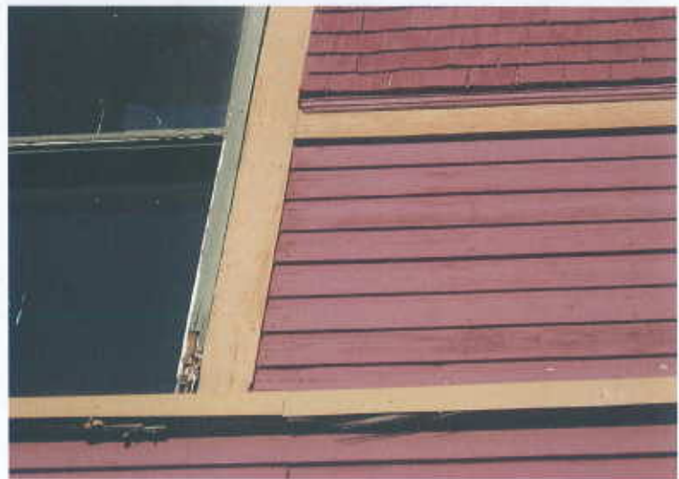
18. Detail, west elevation. Rotted storm window sash and different siding styles.
