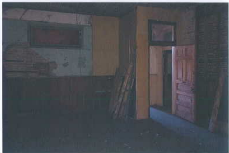
218. Room 211, exposed lath at ceiling and wood studs at walls, and windows are boarded.
