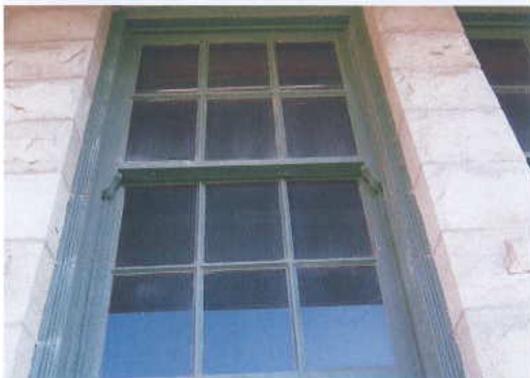
21. Detail, west elevation. Saw cuts at the window frame as a result of preparing masonry joints for repointing.
