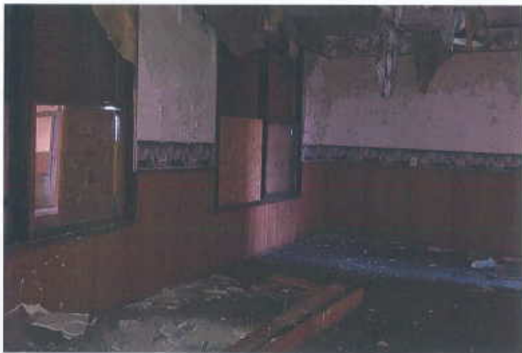
219. Room 212, ceiling, walls, and flooring in poor condition.
