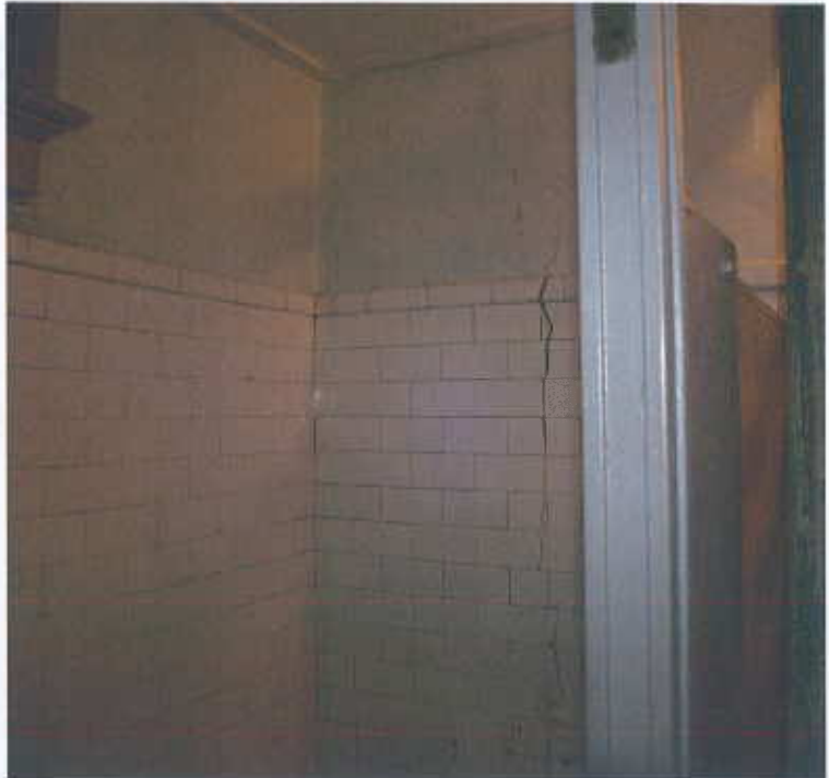
123. Room 105, cracked historic tile wainscoting.
