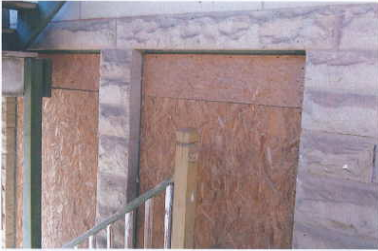
13. Detail, east elevation. Voids in brick masonry, boarded windows, peeling paint at altered stairs.
