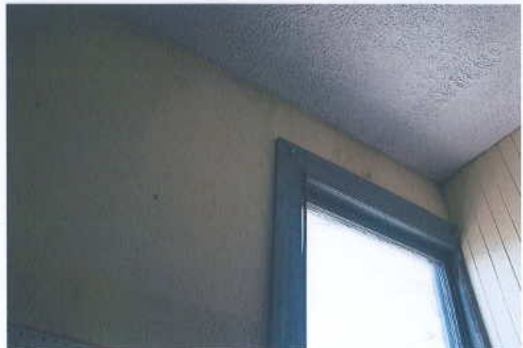
206. Room 203, water infiltration exhibited at ceiling line.
