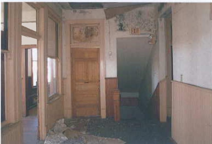
215. Room 210, historic corridor is in poor condition due to damaged ceiling and mold.
