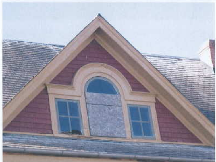
17. Detail, west elevation. Boarded windows and broken glass.
