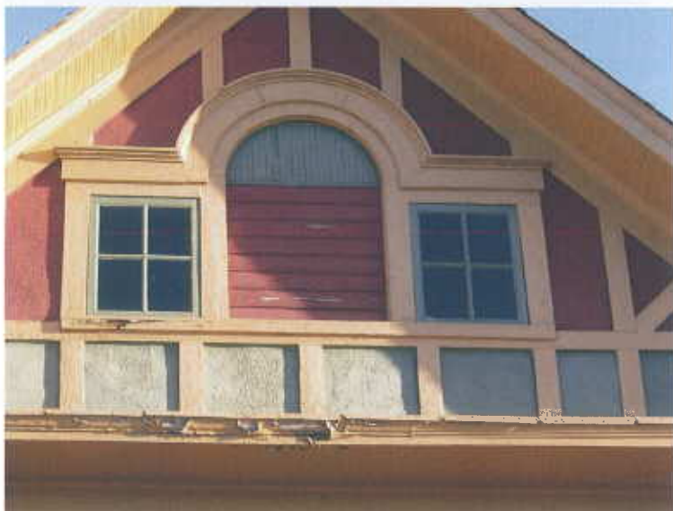
20. Detail, west elevation. Boarded windows, peeling paint.
