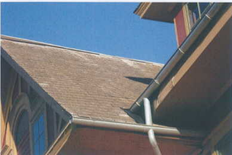
15. Detail, west elevation. Missing shingles at uplifted ridge cap.
