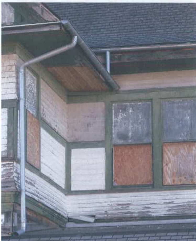
9. Detail, east elevation. Boarded windows, damaged siding, peeling paint, round metal downspouts, half round metal gutters.
