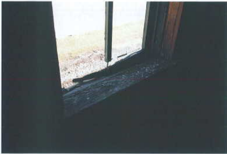
301. Attic, deteriorated wood window and sill.
