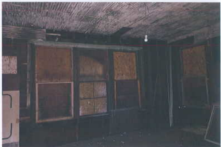
217. Room 211, exposed lath at ceiling and wood studs at walls, and windows are boarded.
