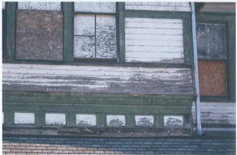
11. Detail, east elevation. Boarded windows, peeling paint.
