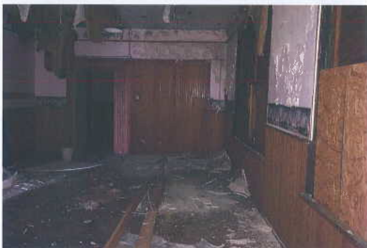
220. Room 212, ceiling, walls, and flooring in poor condition.
