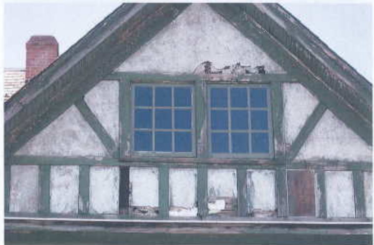
12. Detail, east elevation. Deteriorated stucco and peeling paint.
