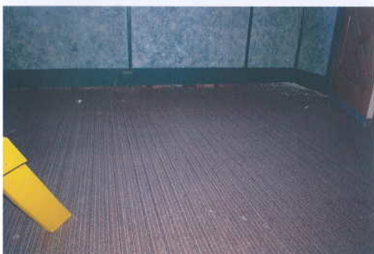
115. Room 102, sagging floor in northwest corner, bricks exposed at floor line.
