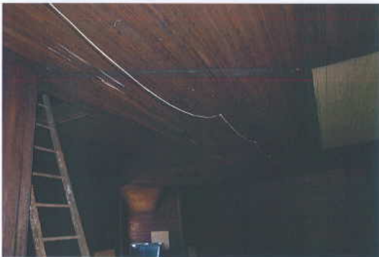
302. Attic, beadboard ceiling with some damage and alterations.
