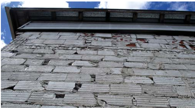
The poor condition of the pre-1940 addition's exterior walls
