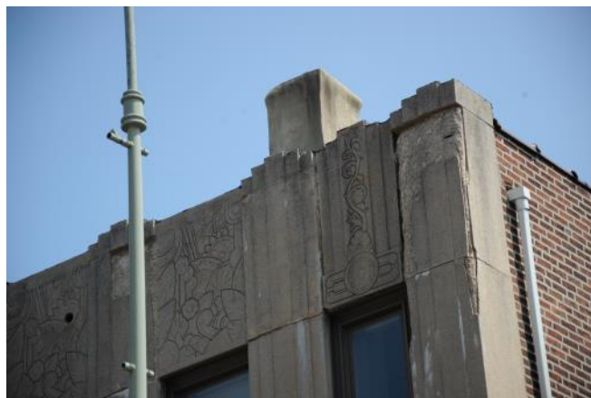
Distinctive architectural details, like the carved relief at the upper limestone panels of this limestone-clad art deco building in Ardmore, should be restored to match the existing.
