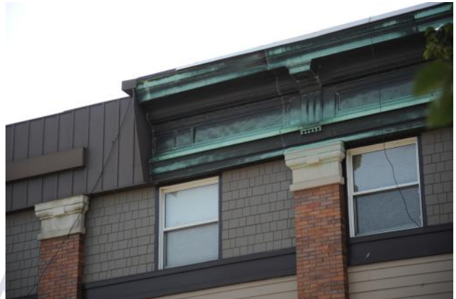
Conspicuously missing major architectural components, like half of the original copper cornice of a commercial building on Lancaster Avenue in Ardmore, should be restored to match the original existing adjacent cornice.
