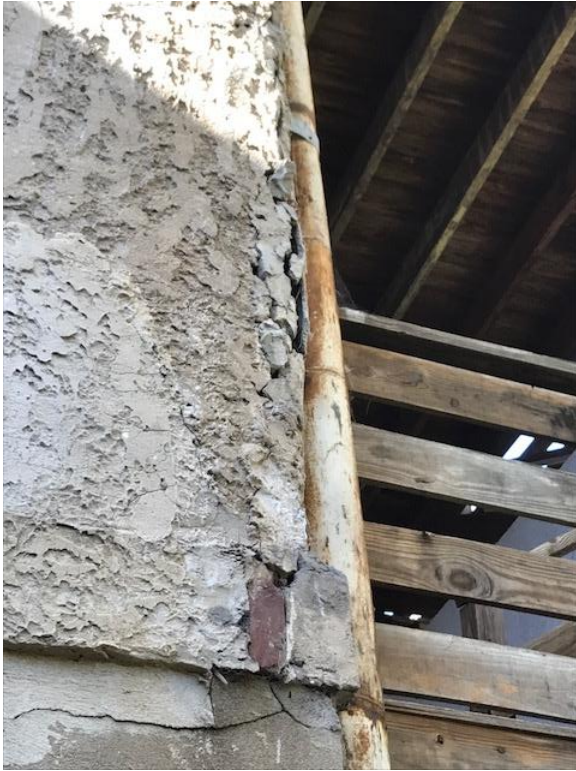
Figure 8 Water damage to stucco corner
