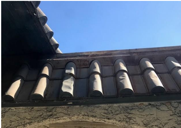
Figure 13 Dented metal roof tiles
