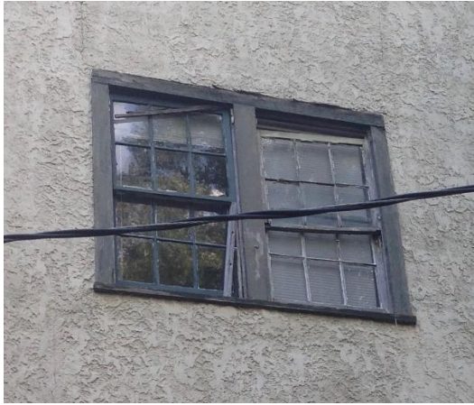
Figure 12 Double hung window in disrepair
