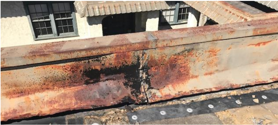
Figure 7 Parapet wall and cap rust
