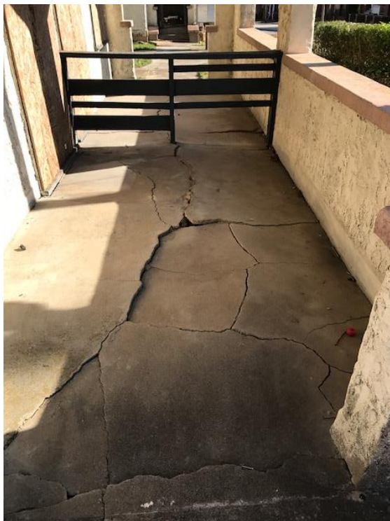
Figure 11 Balcony foundation failing from improper drainage
