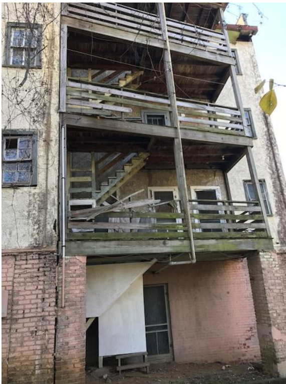
Figure 9 Rear porch with mildew and broken rails
