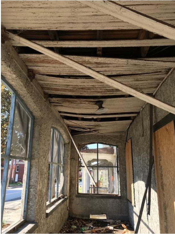
Figure 10 Balcony ceilings failing from water infiltration
