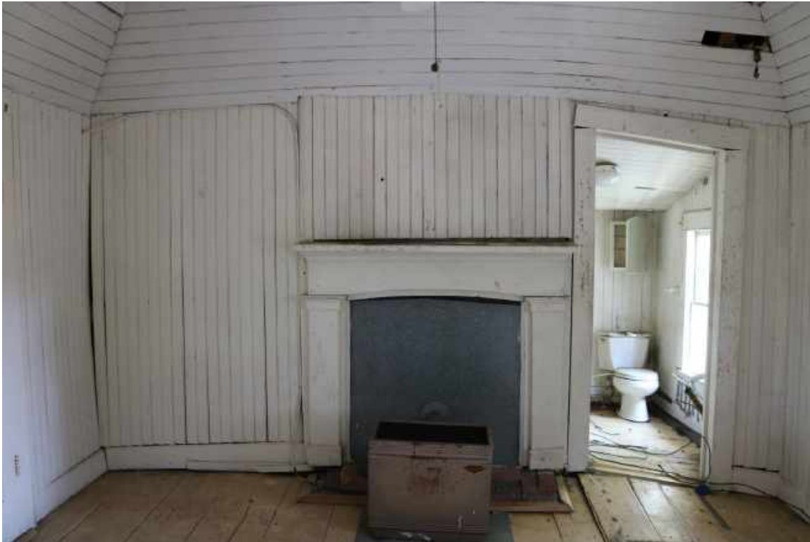
Figure 96: Room 202, Looking West: Note settlement at the northwest corner. The mantle located within this room appears to be the oldest within the structure and is a typical antebellum style.
