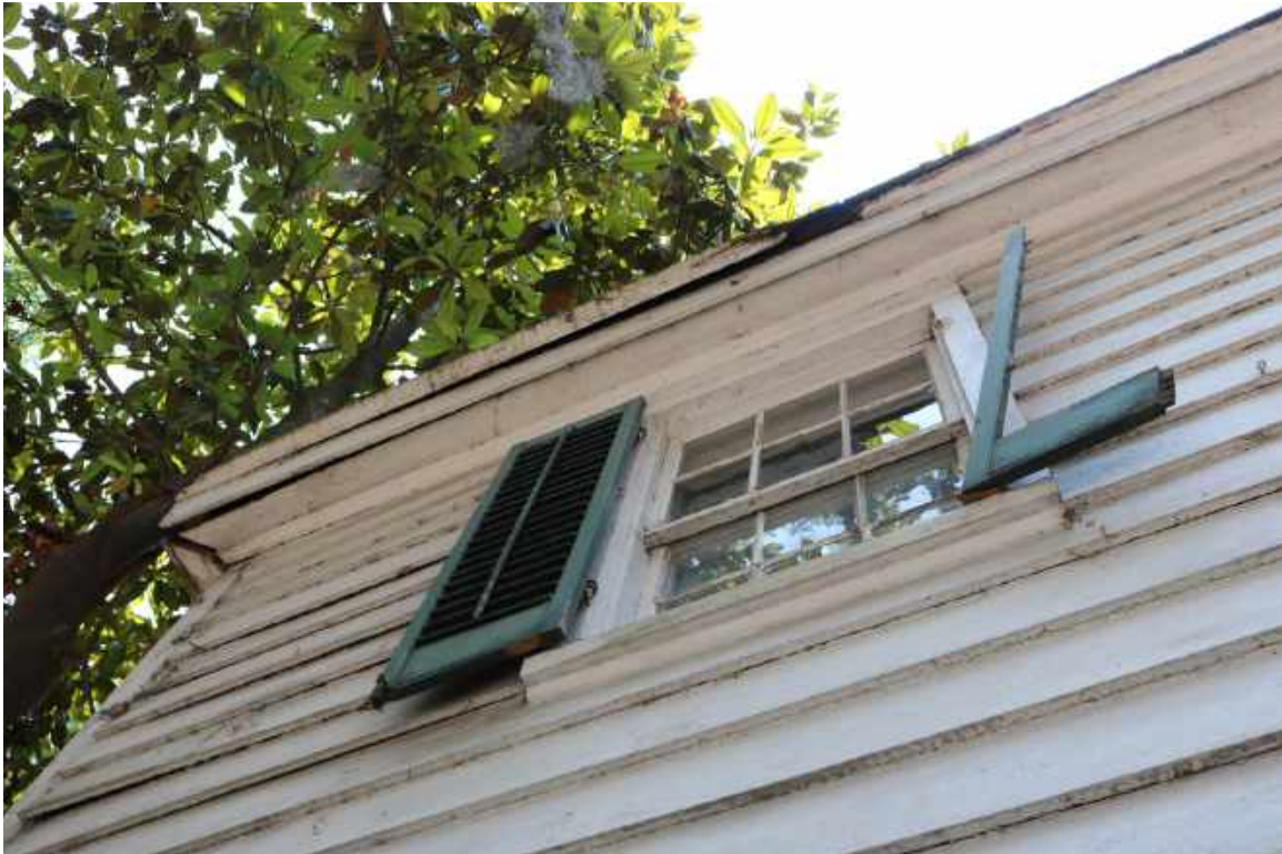
Figure 68: North Elevation of Two-Story Building: Detail of dislodged siding to the left of the window. Note the deterioration within the soffit.
