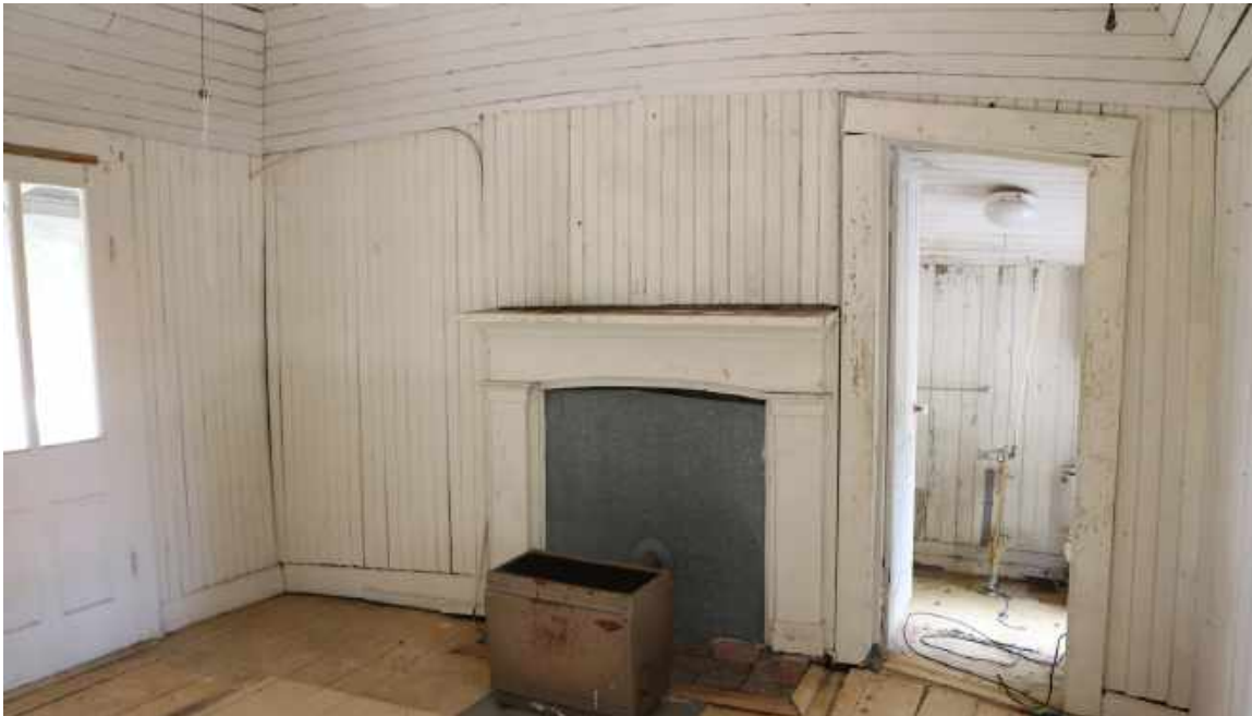
Figure 194: Room 202: Change over time is readily evident throughout the structure.
