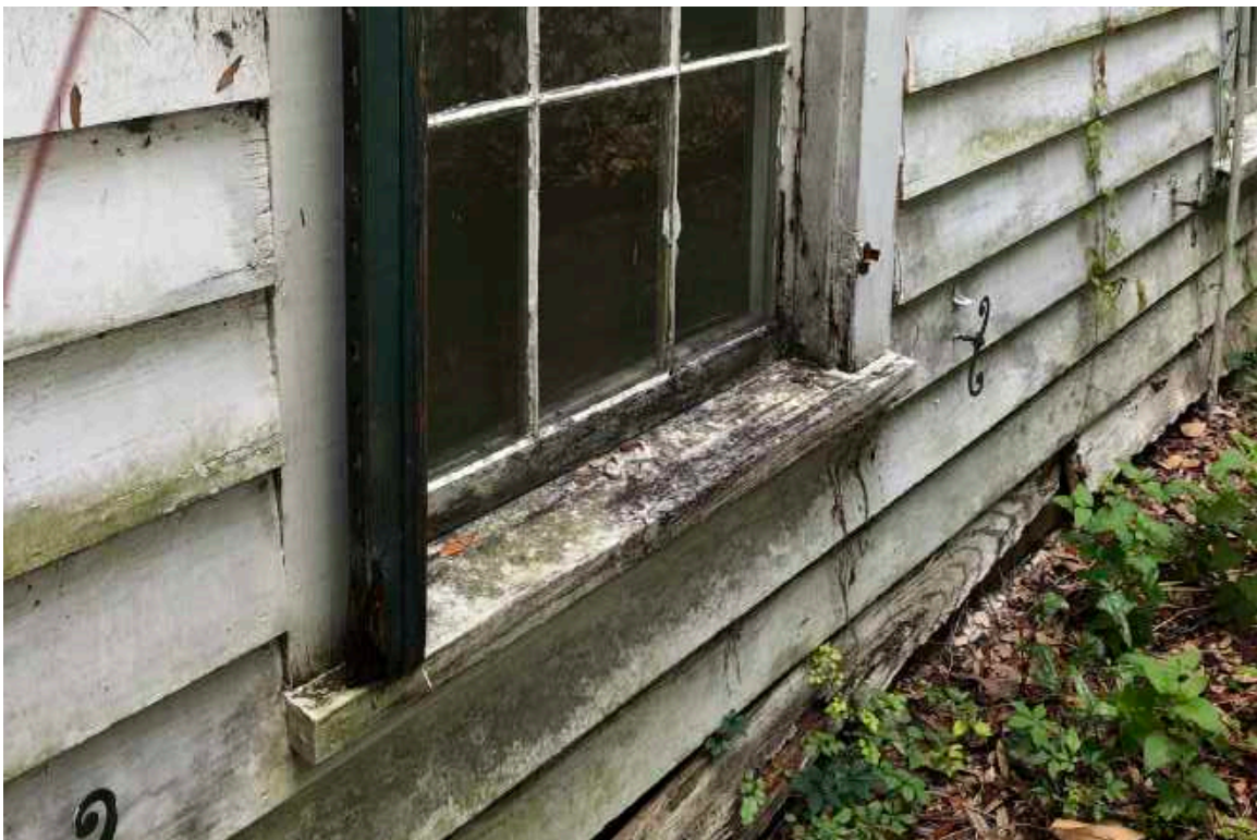
Figure 65: North Elevation of Two-Story Building: Detail of sill conditions.
