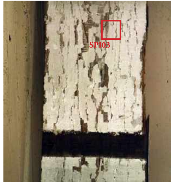
Figure 167: Detailed photograph of limewash finishes found on the underside of the floor board in Room 204. Note location of paint sample SPI03. The extracted paint sample was brittle and easily broken when handled.
