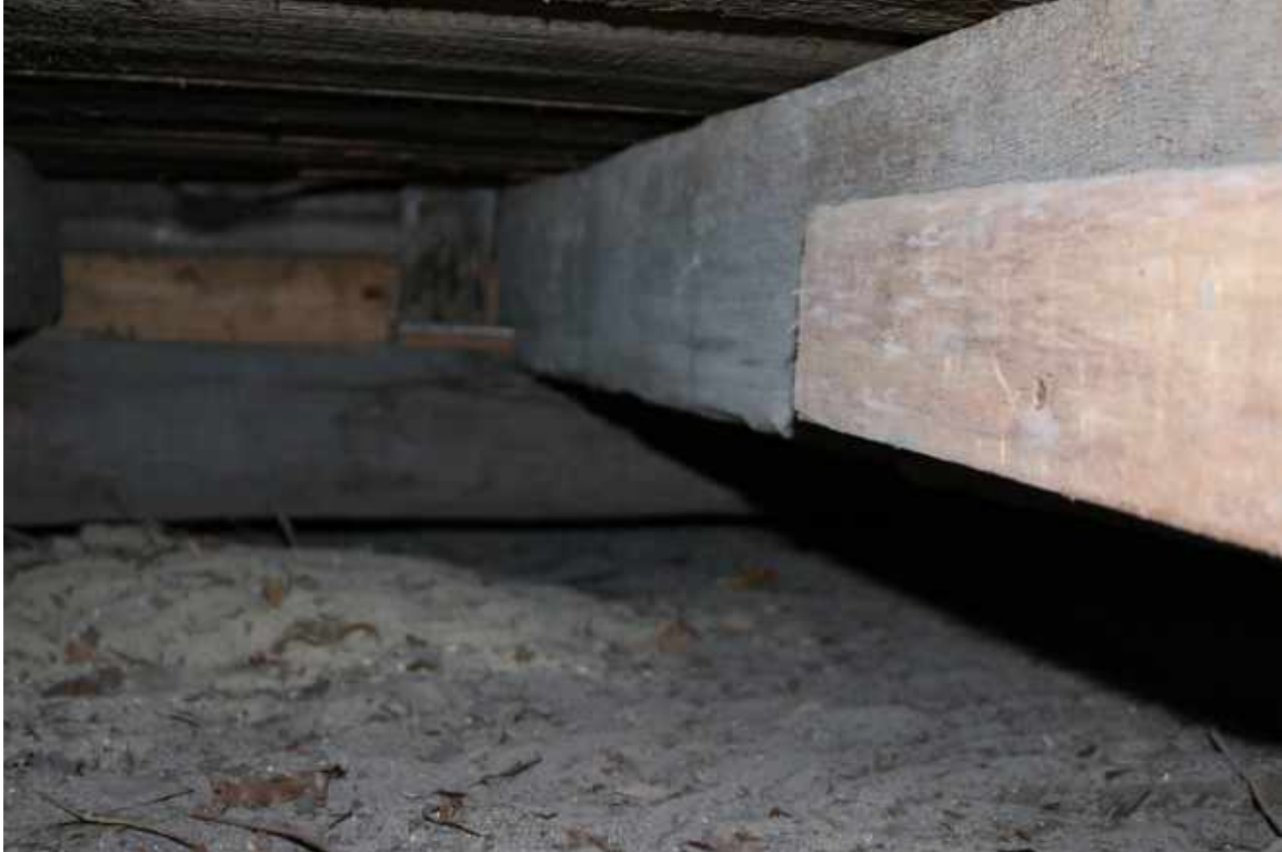
Figure 56: Crawlspace Below Room 103, Looking South: Detail of Floor Joist. The joist appears to be in fair condition.
