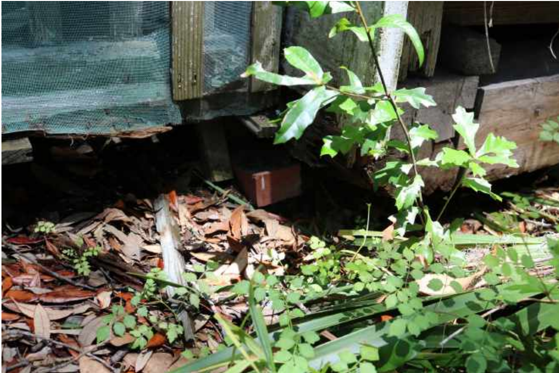
Figure 141: South Elevation: Masonry rubble located beneath the exposed perimeter sill.
