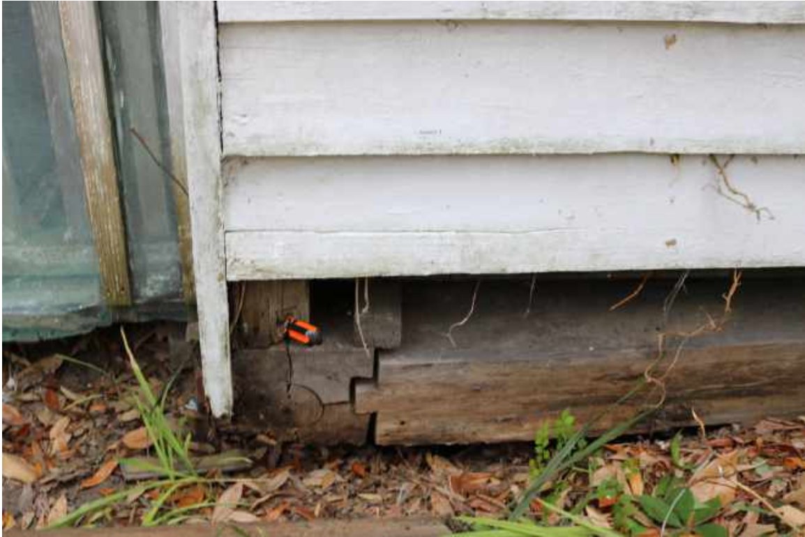
Figure 53: South Elevation of One-Story Building, Southwest Corner: Detail of exposed perimeter sill resting at grade. The bottom of each sill is deteriorated.
