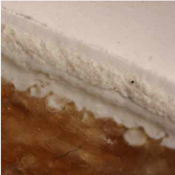
Figure 179: Visible Light 100x- SPI08. Four paint layers are visible in cross section. This sample substantiates the hypothesis that the wall boards were installed prior to the cant boards.
