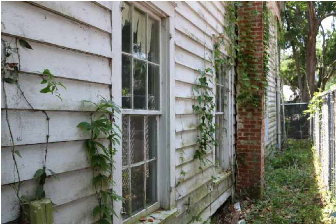
Figure 64: North Elevation of Two-Story Building: Detail of window conditions on this elevation. The original shutters are missing. Biogrowth is prevalent.
