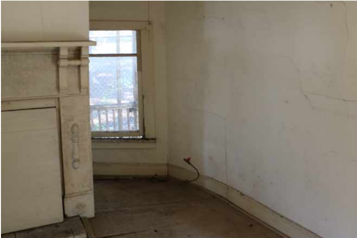
Figure 119: First Floor, Room 101 Northwest Corner: Detail of location #2.
