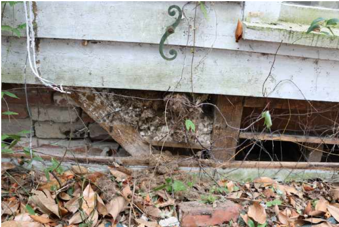
Figure 59: North Elevation of Two-Story Building: Deteriorated corner post at the northeast corner. The internal diagonal chimney is present behind the post.
