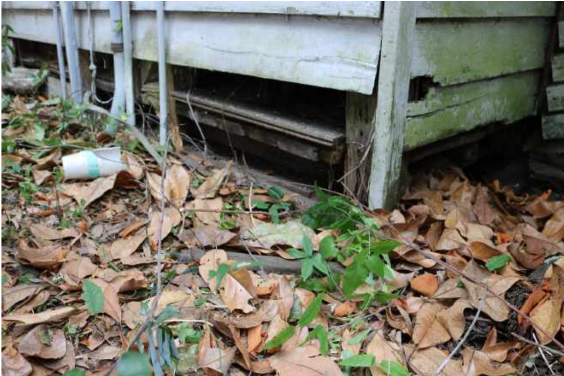
Figure 51: Northeast Corner of One-Story Building, Northwest Corner: The corner post has completely deteriorated. The perimeter sill is covered by soil.
