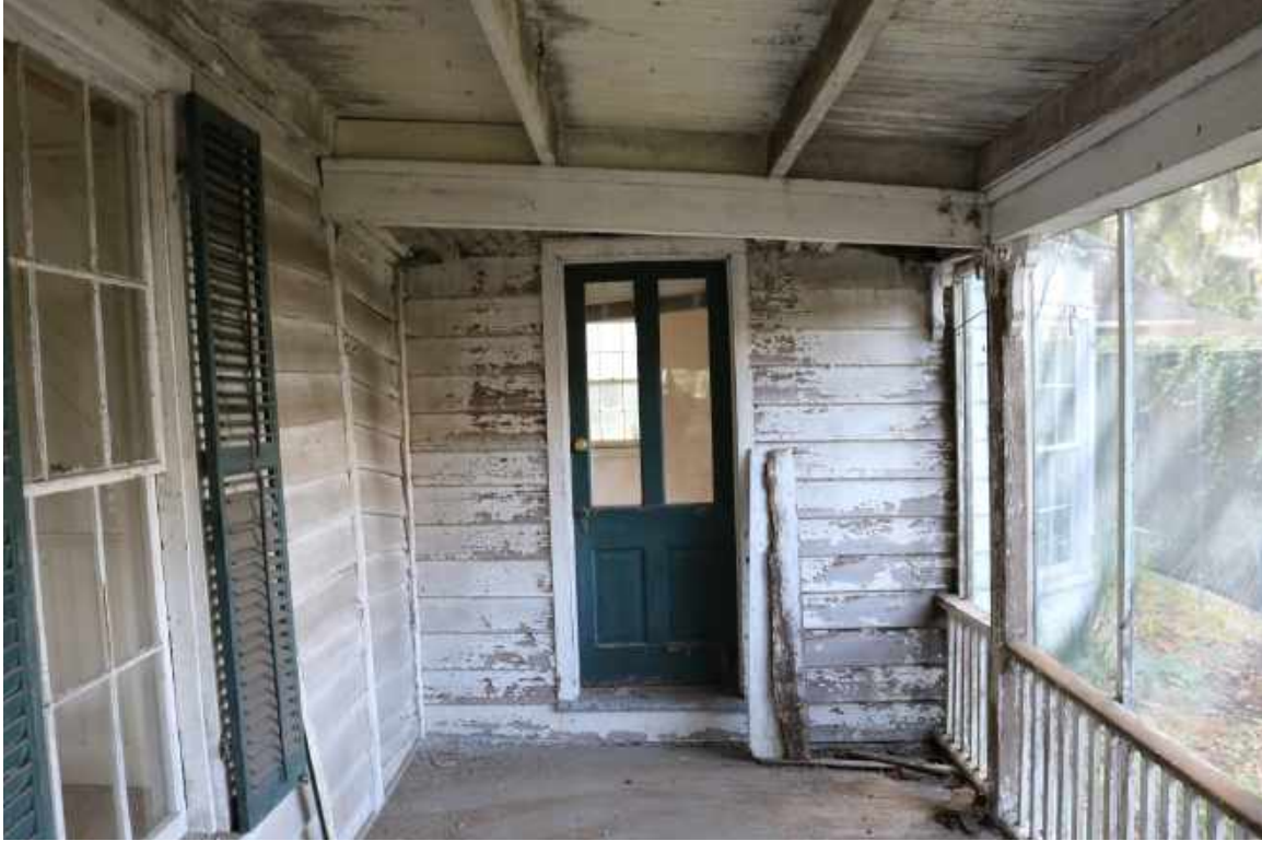
Figure 74: South Elevation, Hyphen Porch: Detail of complete failure of the porch structural elements at the hyphen where it intersects the smaller building.
