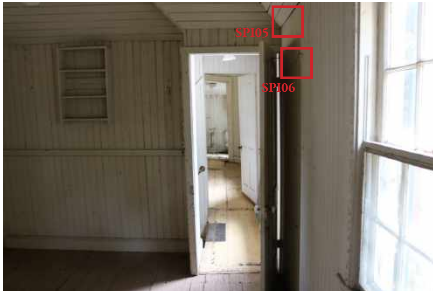
Figure 170: Photograph of Room 204. The wall board and ceiling cant boards were both sampled to confirm whether the cant at the upper section of the wall was installed after the wallboard. Examination of fasteners in the room appear to support this hypothesis.
