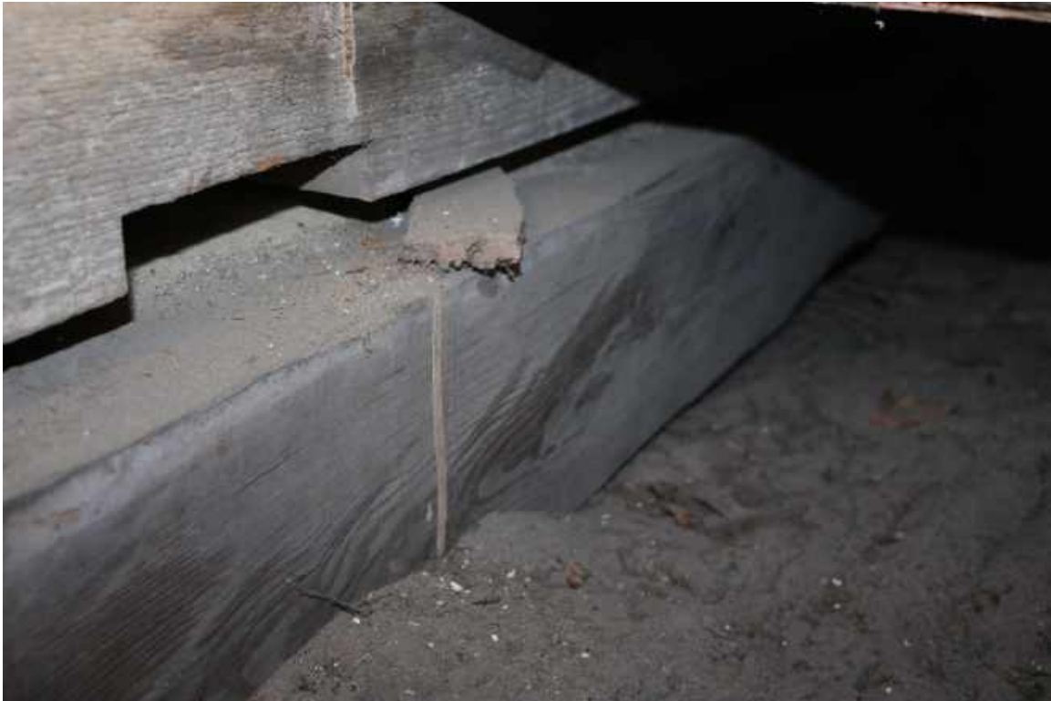
Figure 139: Foundation System - Detail of settlement of foundation members.
