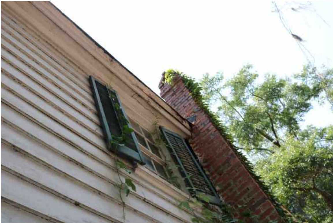
Figure 78: North Elevation of the Two-Story Building: Detail of the north chimney. The chimney is currently leaning away from the structure.
