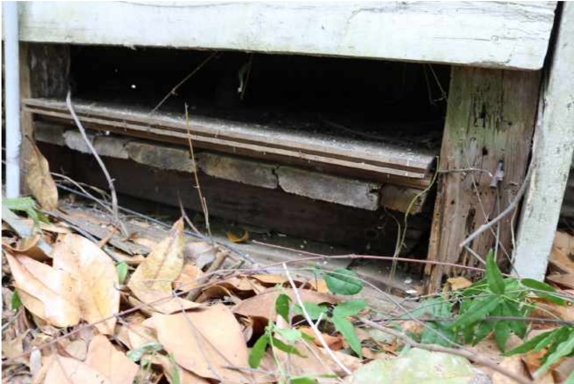
Figure 60: North Elevation, One-Story Building: Detail of floor joists and flooring at this location. Deterioration is evident where the members are in direct contact with the ground.
