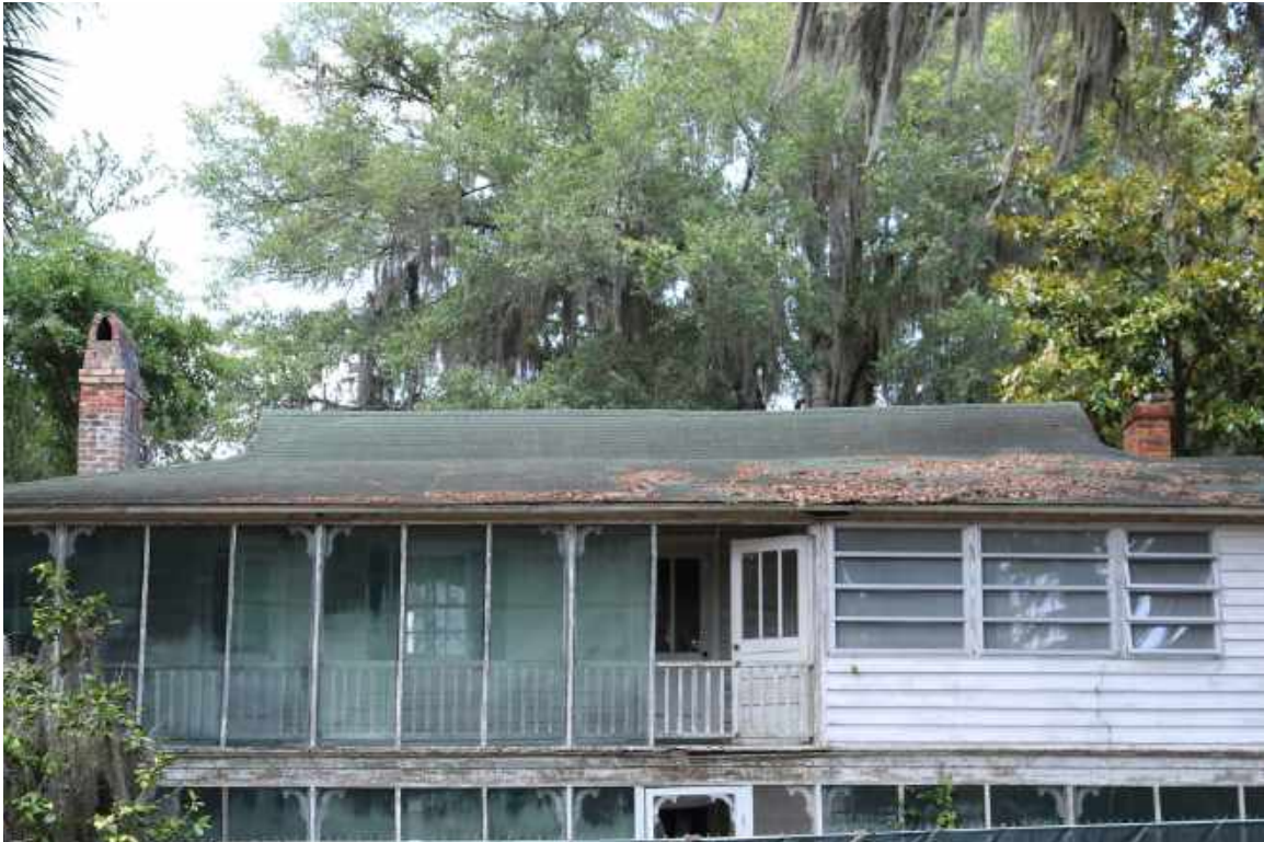
Figure 80: Two-Story Building Roof: The roof is covered with modern green asphalt shingles. The roof has reached the end of its usable service life. Leaf debris commonly accumulates on the low sloped portions of the roof.
