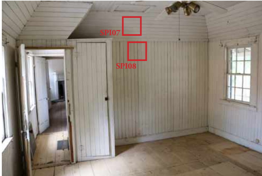
Figure 176: Photograph of Room 202. The wall board and ceiling cant boards were both sampled to confirm whether the cant at the upper section of the wall was installed after the wallboard. Examination of fasteners in the room appear to support this hypothesis.
