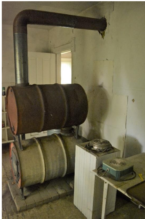
SD_Day County_Anderson House_0011: View of boiler, camera facing southwest.
