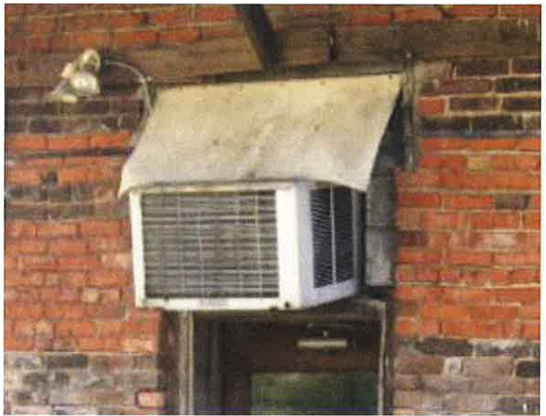
Install window air conditioning units on rear elevations out of public view (15 Webb Road East).
