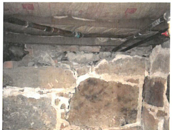
Basement Room 1 – Right Front Corner with Minor Cracking
