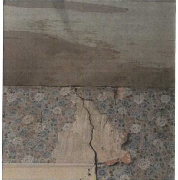
Bedroom 201 – Structural Crack above Front Window
