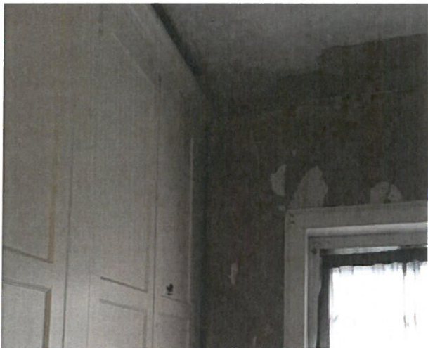
Room 201 – Separation Between Cabinet and Plaster at Front Wall and Ceiling Gap
