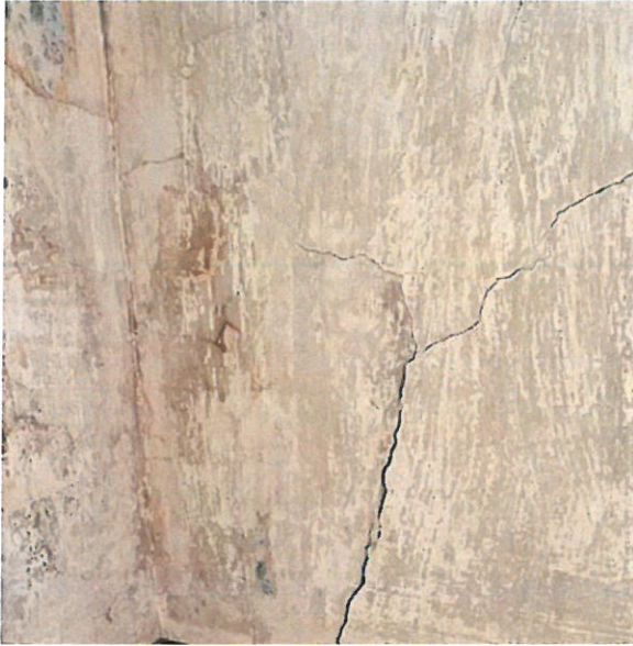
Bedroom 201 – Hairline Cracking in Plaster
