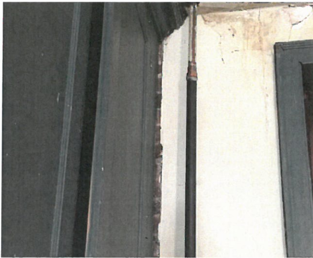
Room 105 – Separation of Press Cabinet and Plaster
