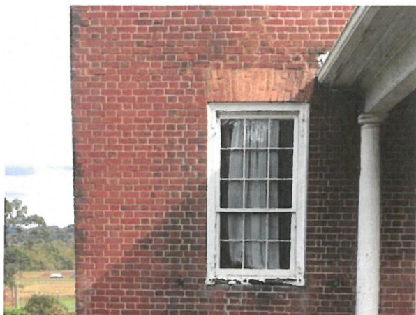
Left Front – Crack Below Rotted Window Sill
