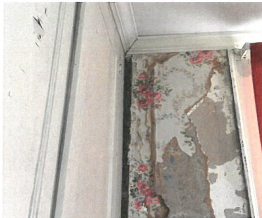
Dining 101 – Enlarged Cabinetry Separation from Plaster
