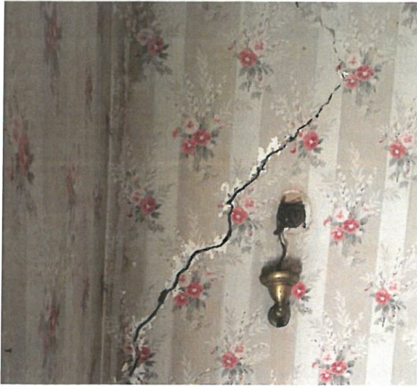
Bedroom 204 Mail Wing – Showing Structural Crack in End Wall
