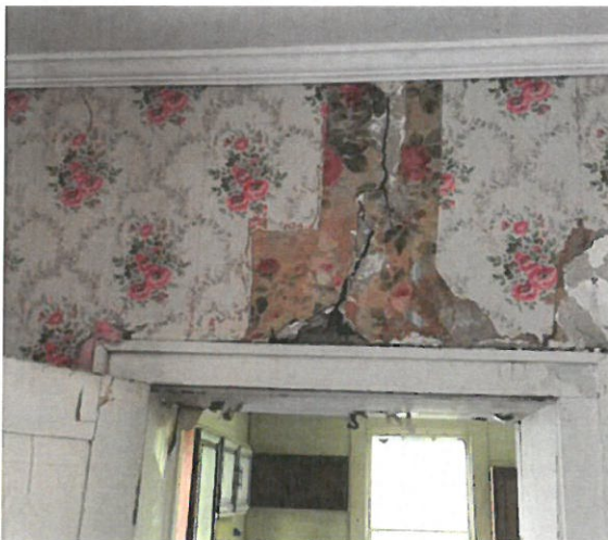
Dining 101 – Crack in Brick Lintel
