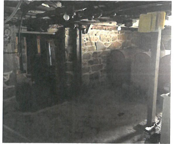
Basement Room 2 – Looking at Fuel Tanks
