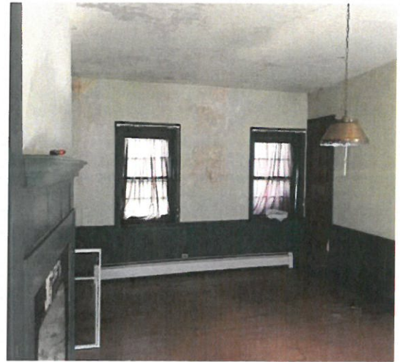
Bedroom 205 – Rear Wall
