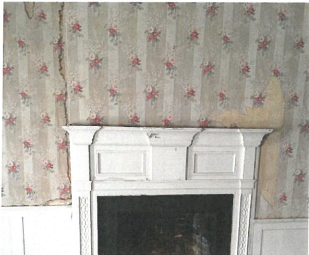
Bedroom 204 – Showing Crack Beside Cabinetry Tie Turnbuckle
