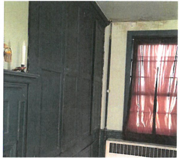
Room 105 – Rear Corner with Cabinet and Plaster Gap
