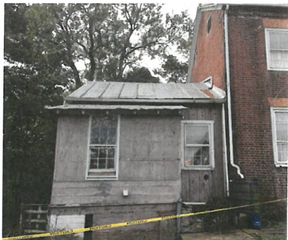
Right Rear – Cracking at Cornice and Between Windows
