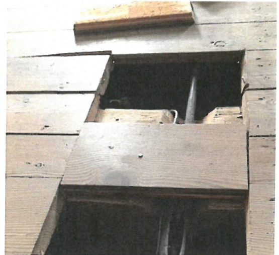
Bedroom 204 – Floor Access to Cable
