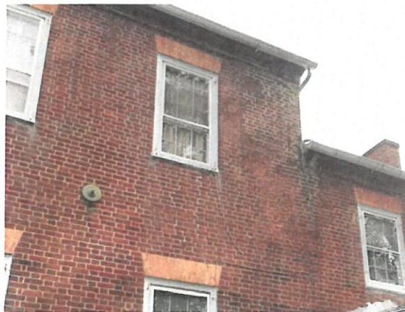
Right Front Upper Level – Previous Repointing Work
