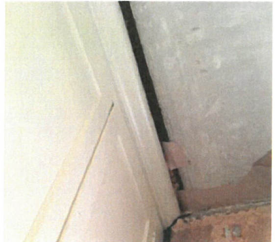
Room 201 – Separation Between Cabinetry and Ceiling
