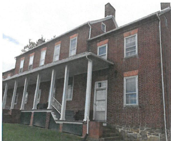
Left Rear – Cracking Below Window and Foundation Repointing
