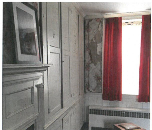
Dining 101 - Front Wall Separation Between Plaster and Cabinet
