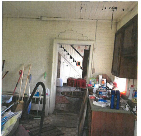
Interior Wall – Showing Cracking in Door Lintel
