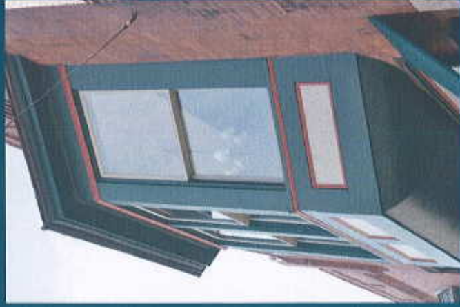
Wood replacement window
