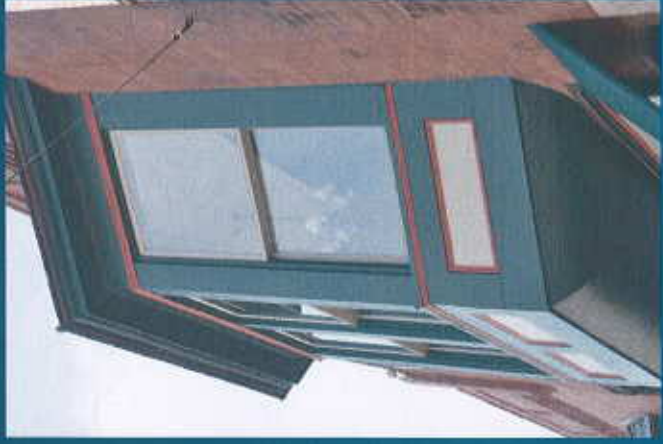
Wood replacement window
