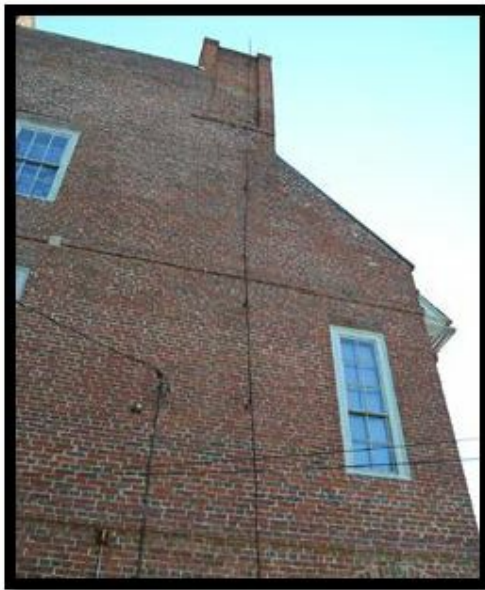
Image of lightning protection at the Warner House in Portsmouth.
