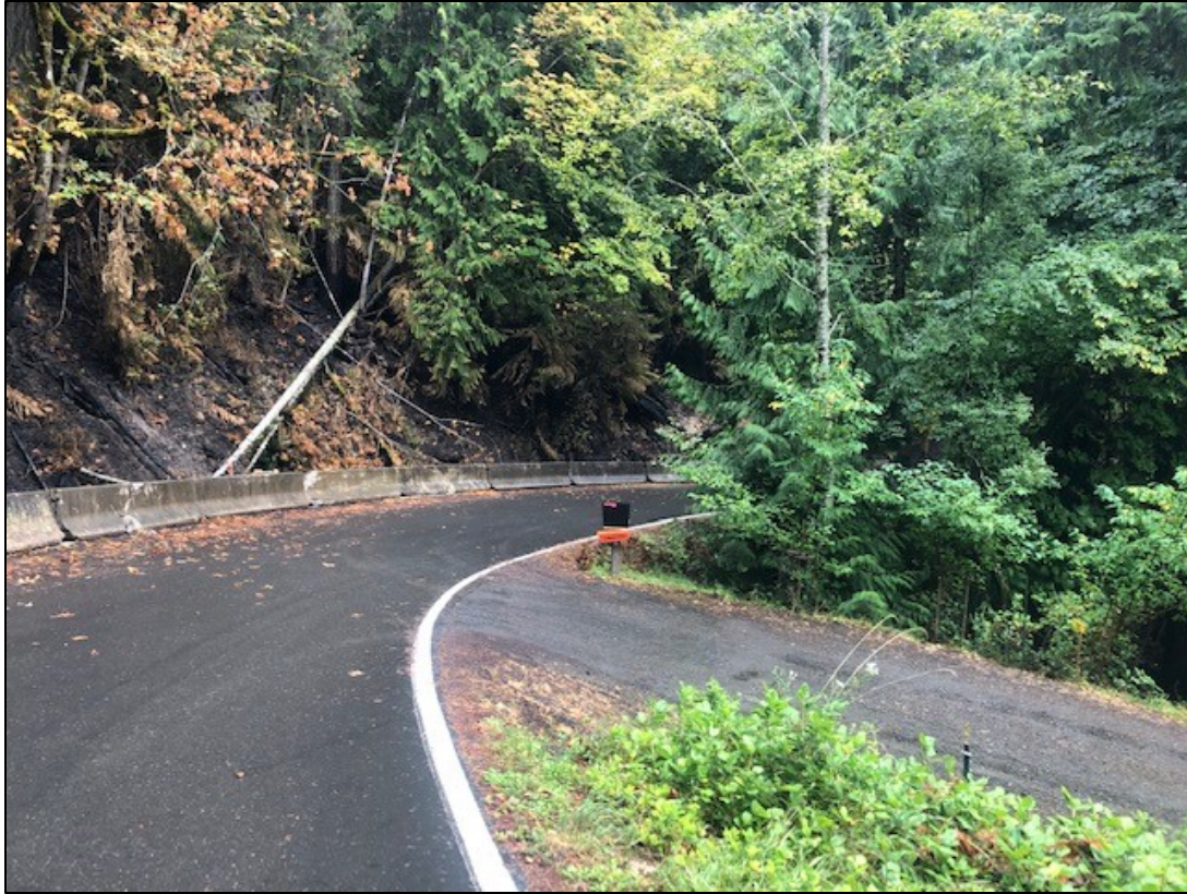
Figure 11: Several homes appear to be directly in the path of potential rock- and treefall. The existing line of Jersey barriers at the edge of the road provides some critical protection.
