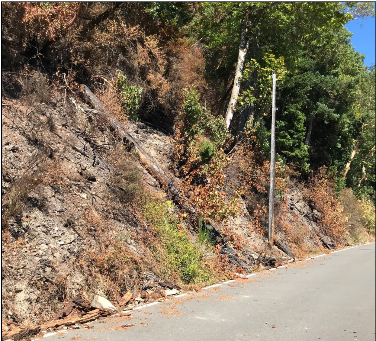
Figure 13. East Beach Road ditch filled with slope debris.
