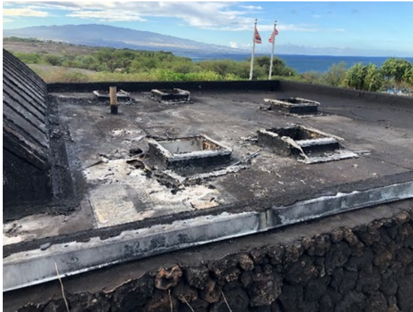
Photo 1. Roof of fire-damaged comfort station.
