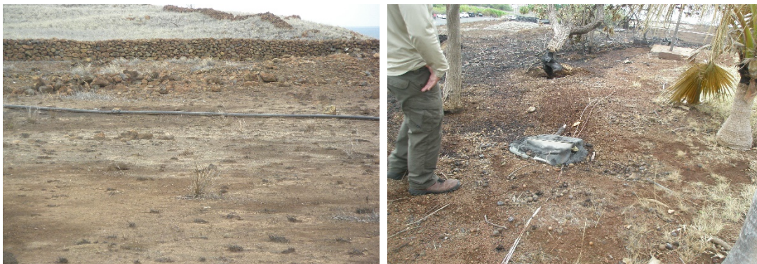
Photo 2. Fire-damaged water supply line (left) and irrigation system (right).
